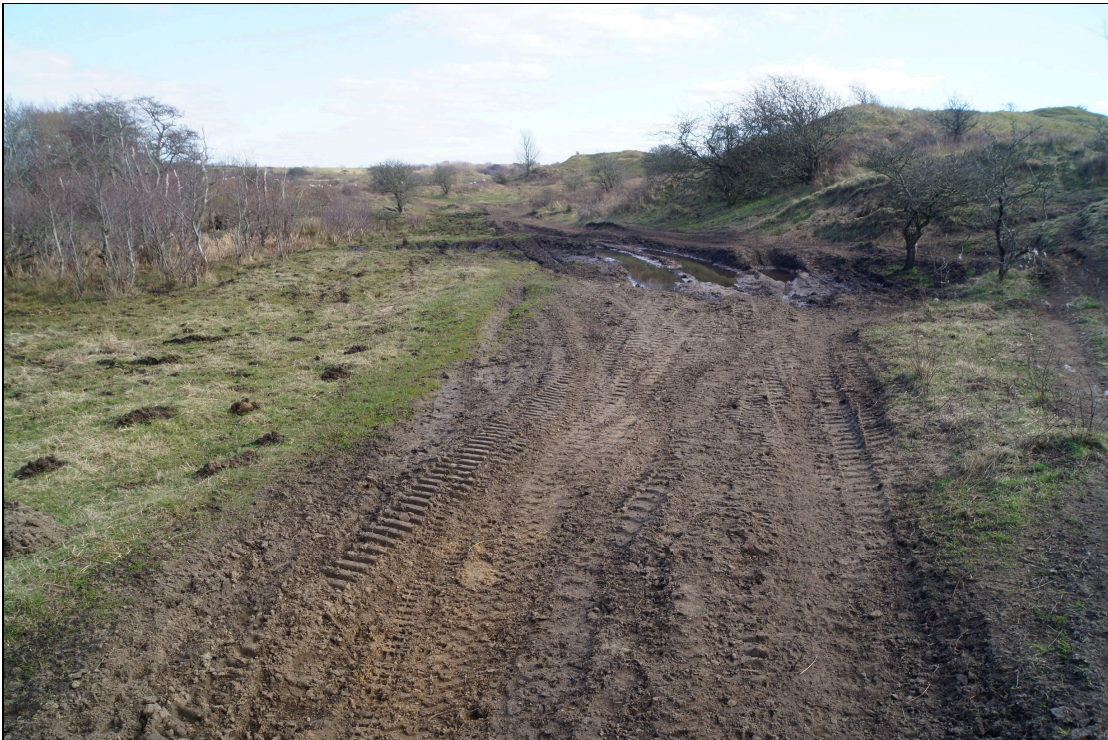
Plate 39: KFD2021_139. A section of trackway outside the Scheduled Monument. Bog mats were not used here. Looking east-southeast. SS7987482595
