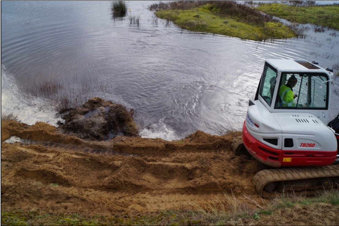
Plate 19: KFD2021_119. The start of the excavation work at the Horseshoe Slack. Looking south. SS7918282819
