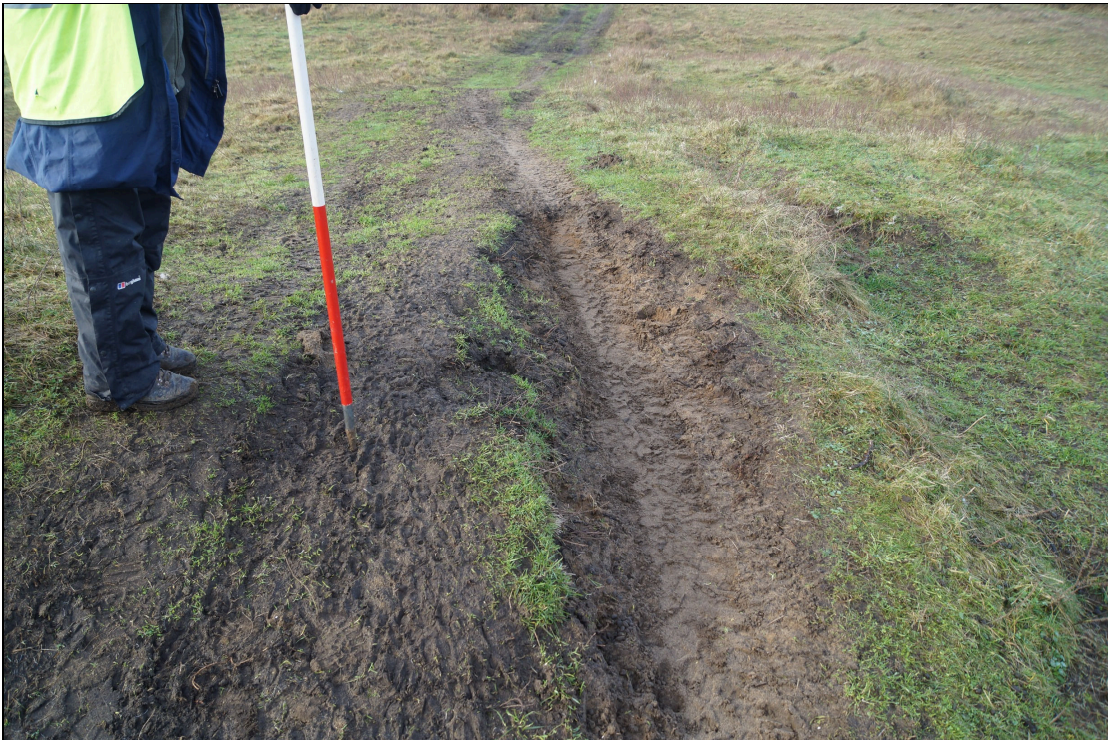
Plate 5: KFD2021_105. Part of the trackway through the Scheduled Monument before the bog matting was put down showing existing erosion, looking west-southwest.
