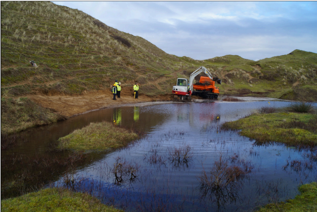
Plate 21: KFD2021_121. The start of the excavation work at the Horseshoe Slack. Looking east. SS7917082810
