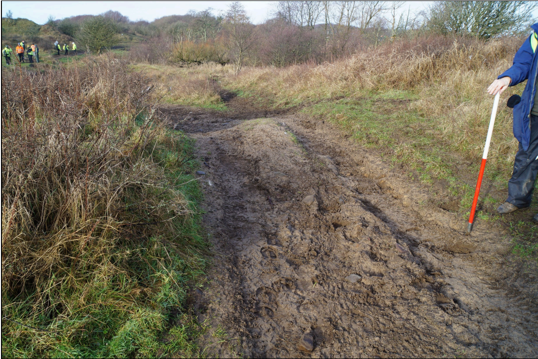
Plate 7: KFD2021_107. This is the point where the trackway crosses the town boundary in the Scheduled Monument, looking west-northwest. This shows existing erosion before the bog mats were put down. Stones are becoming exposed, SS7997882593.
