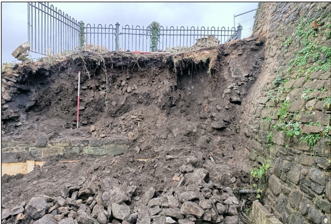
Plate 16. View to east of controlled demolition of the Boundary Wall [007] following the collapse of the section.
