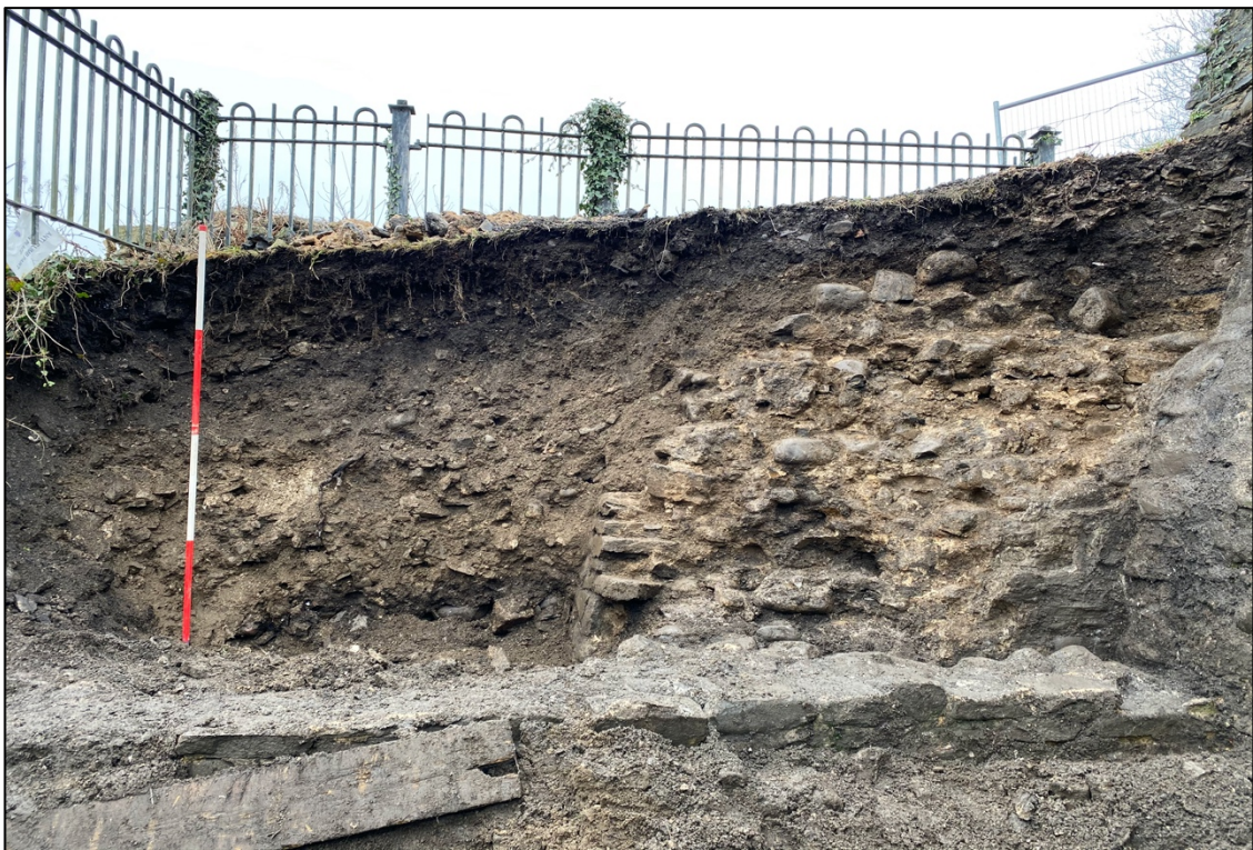
Plate 18. View to the east of the excavated and cleaned section (following the collapse) showing the masonry of the Northeast Tower [012], medieval deposits (011) and later back-filling deposits (013, 014 and 015).
