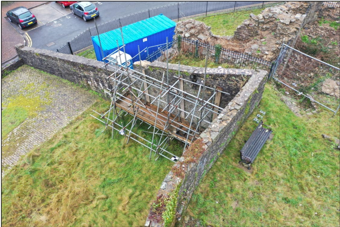
Plate 11. Oblique view to NE of the collapsing Boundary Wall and Quakers Wall atop the North Curtain Wall.
