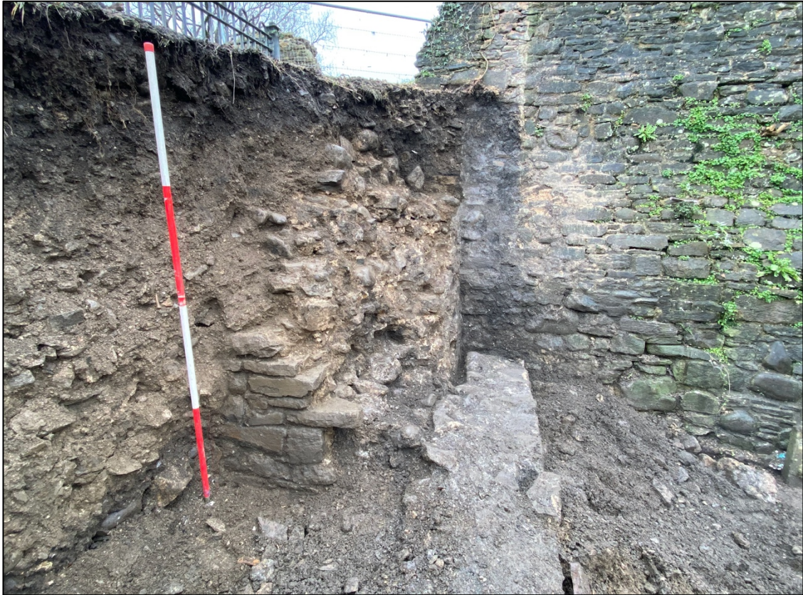
Plate 19. View to the south showing the masonry of the Northeast Tower [012], including surviving facing stones, medieval deposits (011) and later back-filling deposits (013, 014 and 015).
