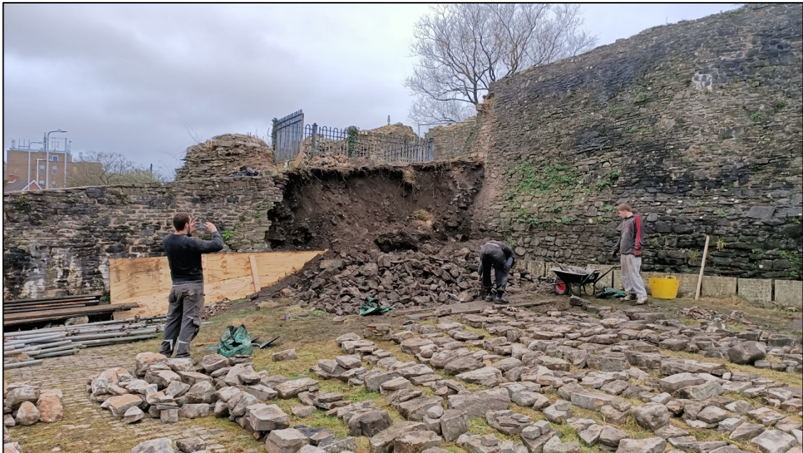
Plate 15. View to southeast of controlled demolition of the Boundary Wall [007] following the collapse of the section.
