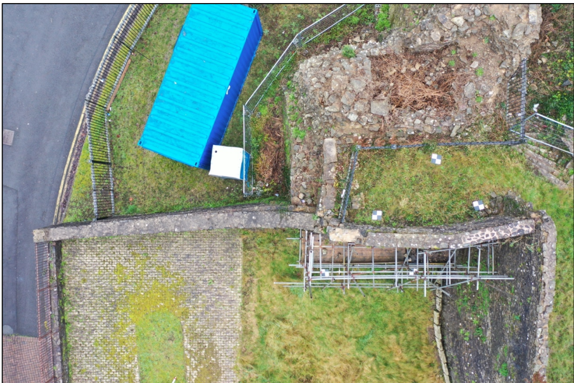
Plate 12. Nadir view of the collapsing Boundary Wall and Quakers Wall atop the North Curtain Wall.
