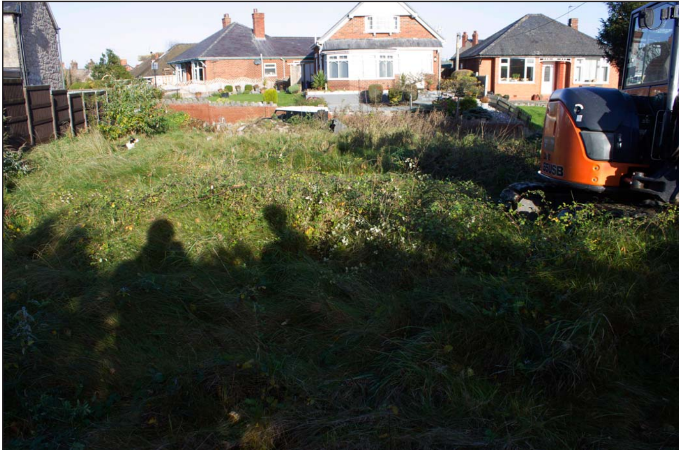
Plate 02: Pre excavation shot of plot adjacent to Castle Hill, Hylas Lane, Rhuddlan, Denbighshire - from the south - no scale
