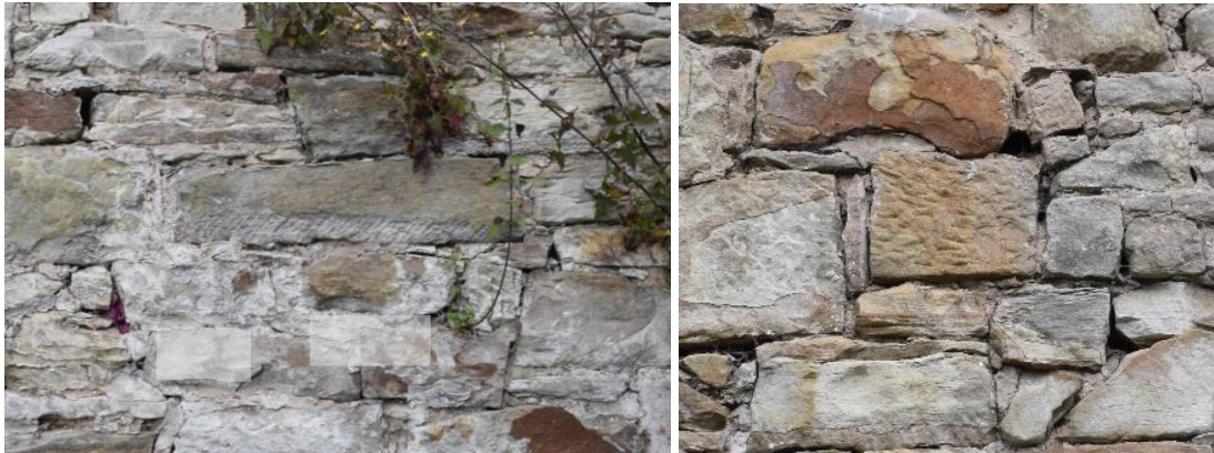
Fig. 6. Dressed stonework within the perimeter wall between near 'The Mount' CPAT Photo 5003_25 and 26
