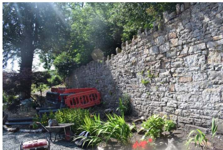
Fig. 5. Pre-removal shot of damaged section of perimeter wall CPAT Photo 5003_3
