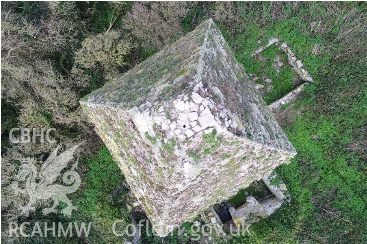
Figure 41 Vertical UAV view of the tower's roof showing vegetation and weeds taking hold on the pyramidal sides and loose, mortarless stones becoming fragmented at the apex. A small drain hole can be seen in the apex (© CHERISH Project, 26 November 2018. Puffin_Island_UAV_26112018_0120.TIF).
