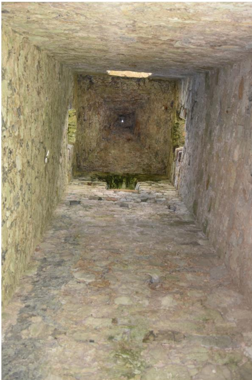
Figure 44 View inside the twelfth century tower; note the small drain hole at the apex of the roof (© CHERISH Project, 21 June 2018 - CH2019_093_005).
