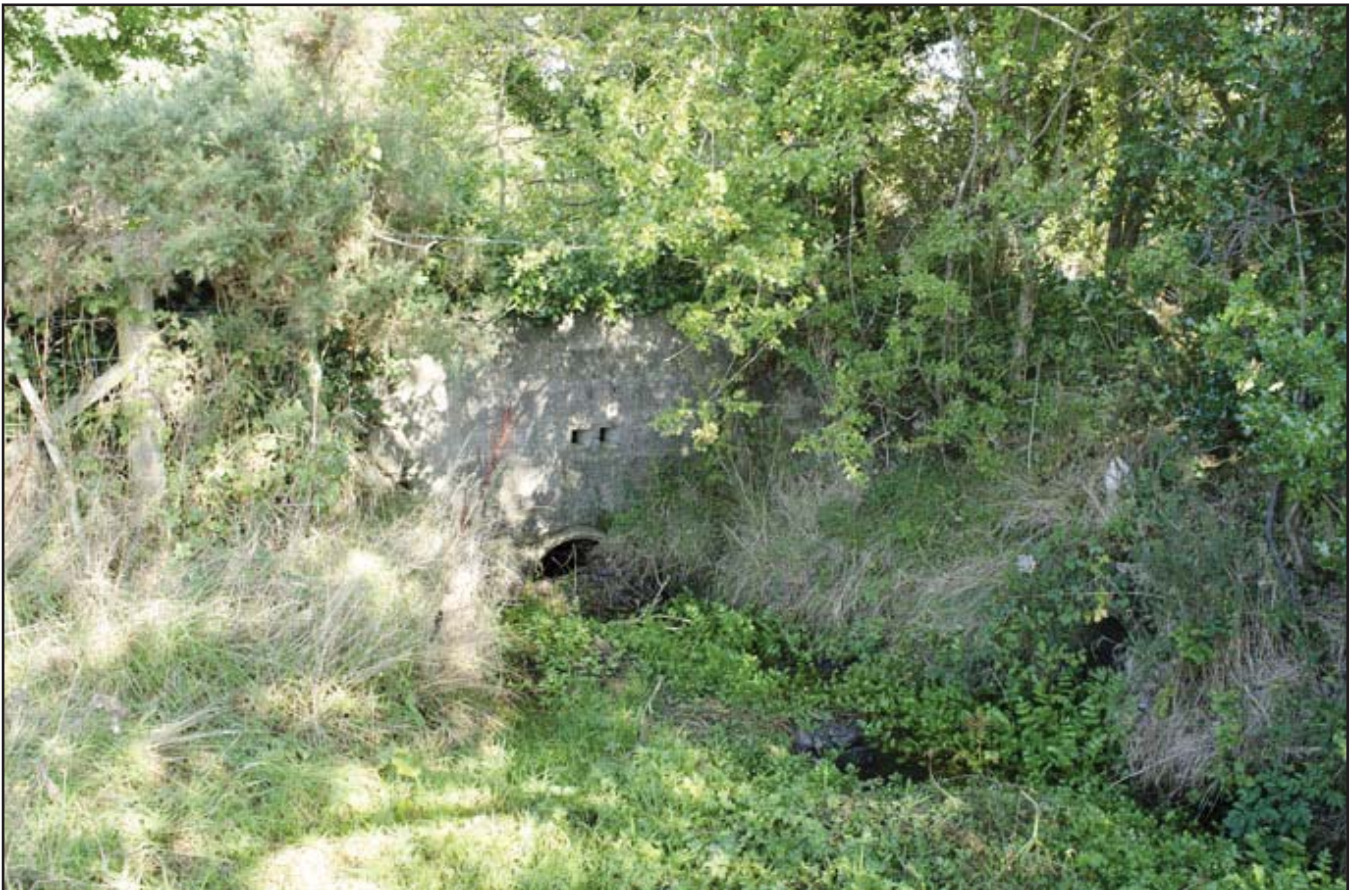
Plate 16: Concrete wall & pipe culvert at northeast corner of Field 1; scale not used; view from S (archive reference: G2739_013).
