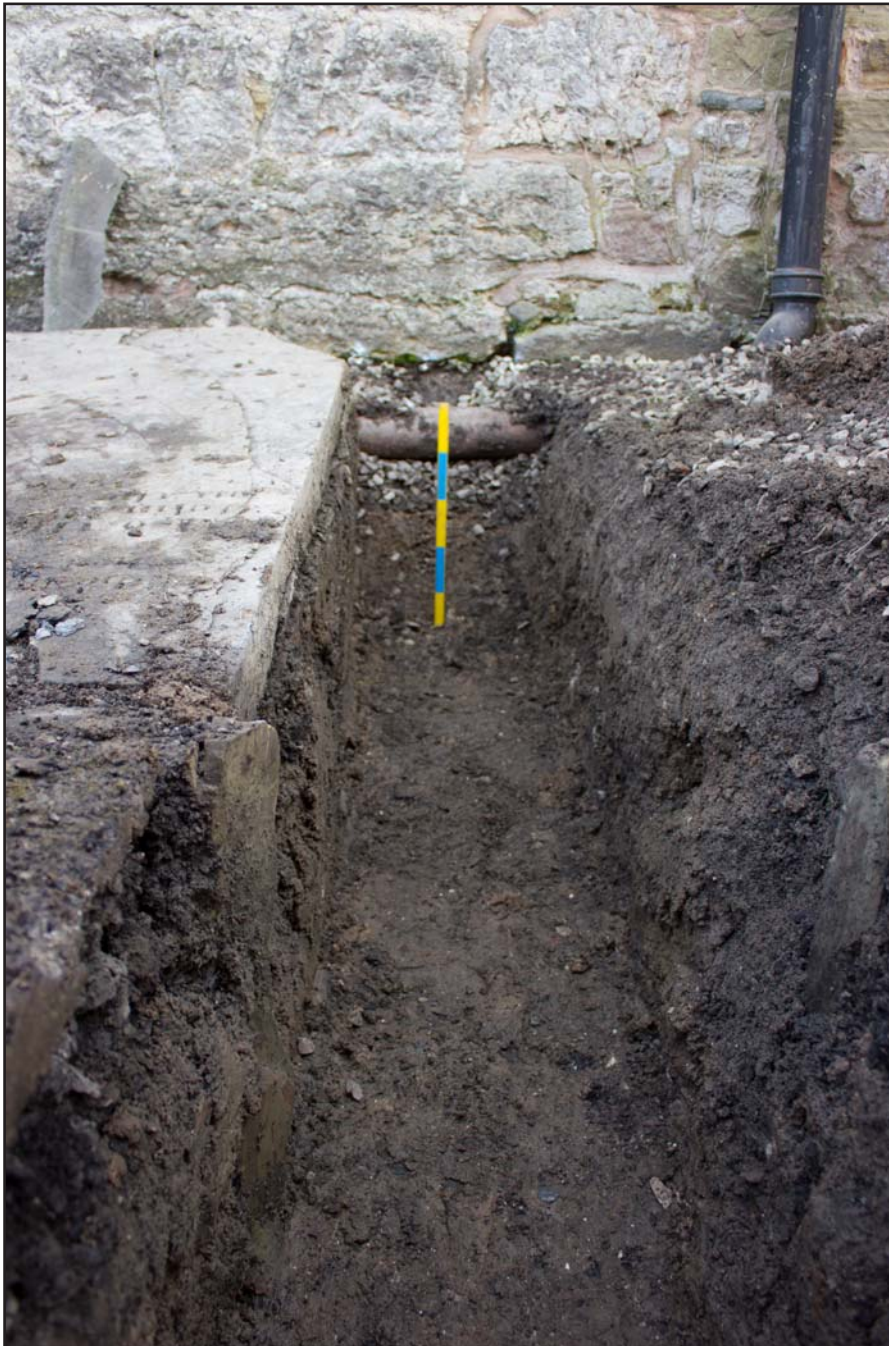
Plate 36: First inlet (southern) to main drainage trench at St. Asaph Parish Church, St. Asaph, Denbighshire - from the west - scale 0.50m
