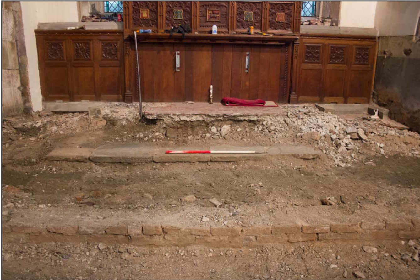
Plate 24: Sandtone slabs foundation footing for altar at St. Asaph Parish Church, St. Asaph, Denbighshire - from the west - scale 0.50m
