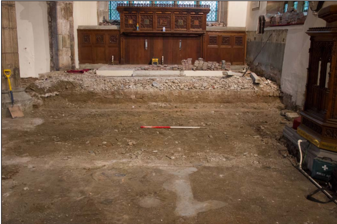
Plate 22: Post removal of limestone kerbs at St. Asaph Parish Church, St. Asaph, Denbighshire - from the west - scale 1m
