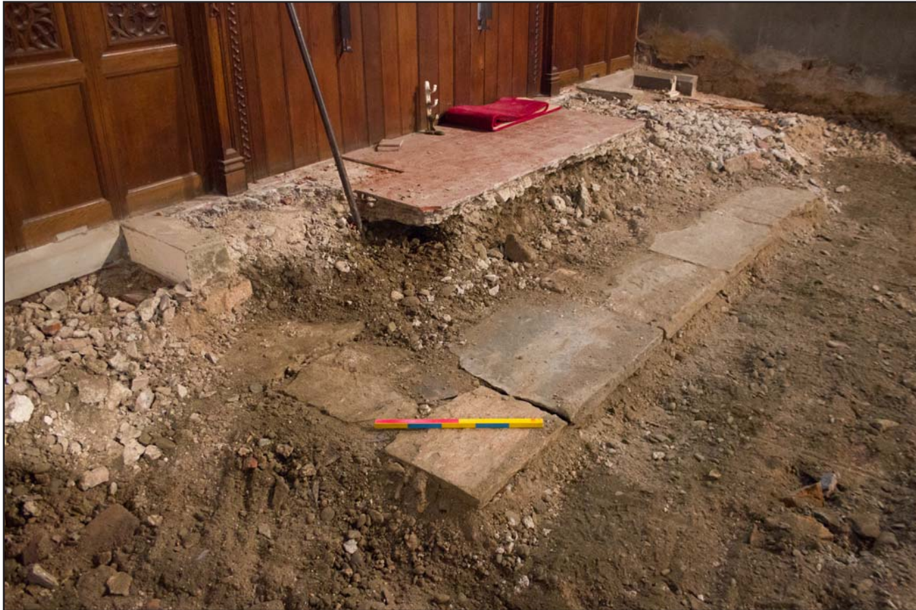
Plate 25: Sandtone slabs foundation footing for altar at St. Asaph Parish Church, St. Asaph, Denbighshire - from the northwest - scale 0.50m
