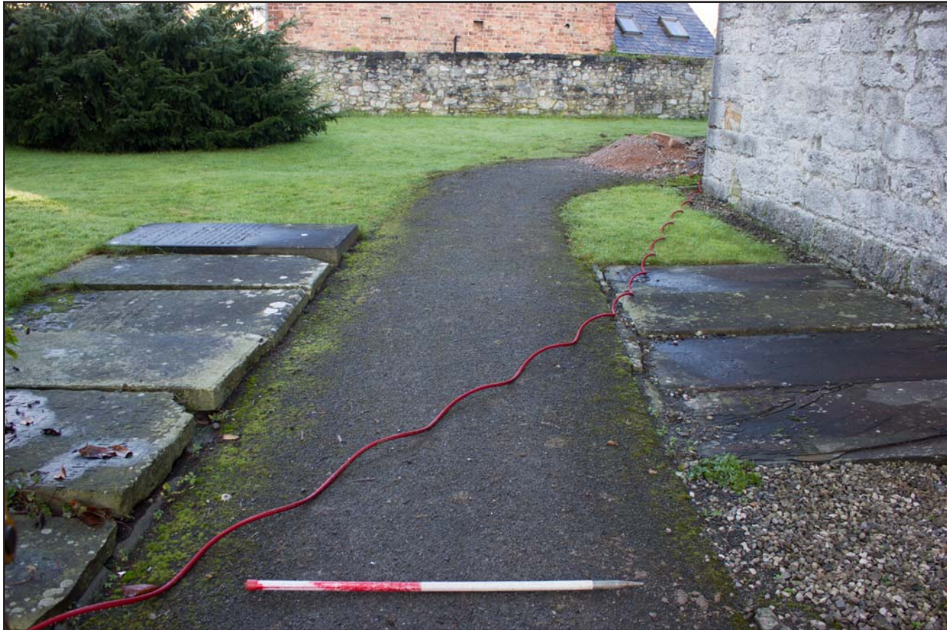
Plate 28: Pre excavation shot of drainage route to the west of St. Asaph Parish Church, St. Asaph, Denbighshire - from the south - scale 1m
