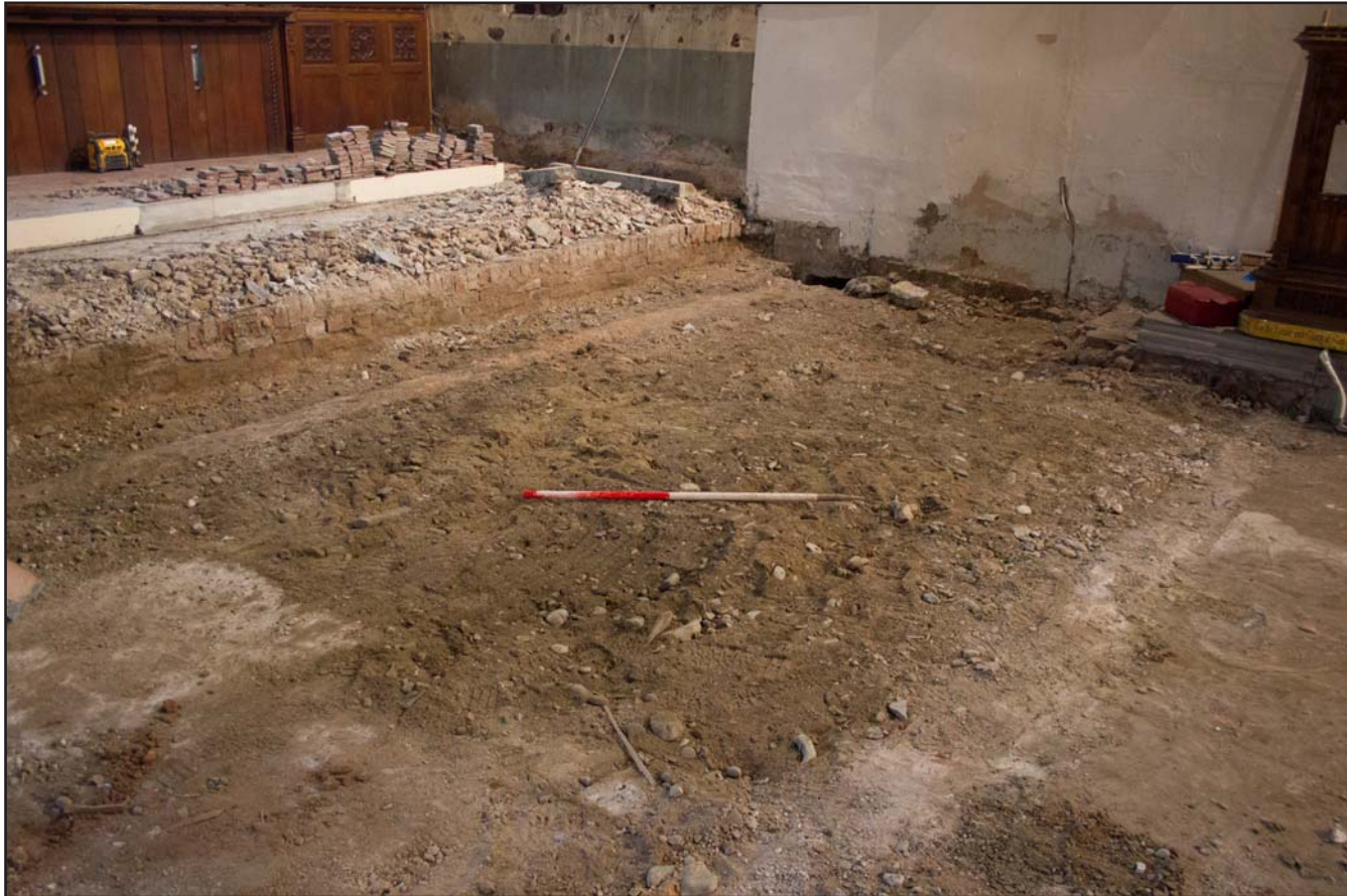
Plate 23: Post removal of limestone kerbs at St. Asaph Parish Church, St. Asaph, Denbighshire - from the northwest - scale 1m
