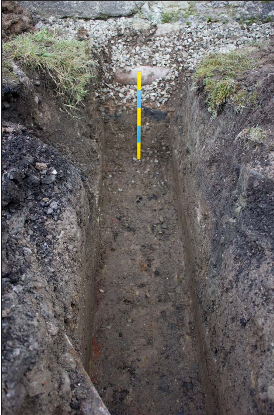
Plate 37: second inlet (northern) to main drainage trench at St. Asaph Parish Church, St. Asaph, Denbighshire - from the west - scale 0.50m
