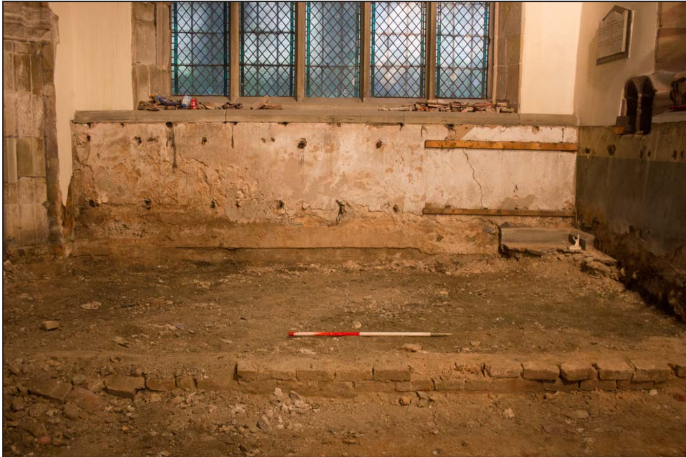
Plate 26: Post removal of carved altar at St. Asaph Parish Church, St. Asaph, Denbighshire - from the west - scale 1m
