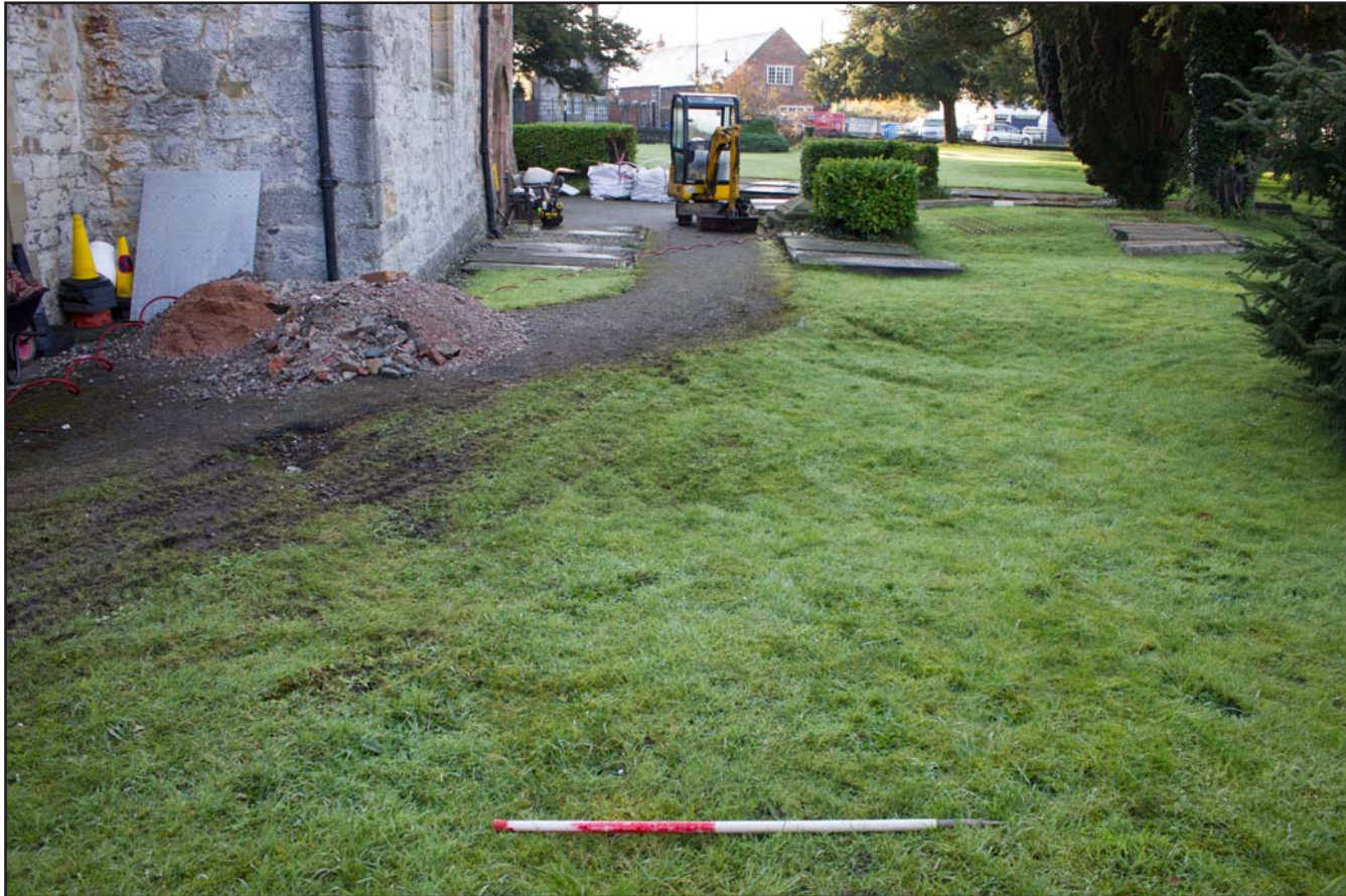
Plate 29: Pre excavation shot of drainage route to the west of St. Asaph Parish Church, St. Asaph, Denbighshire - from the north - scale 1m
