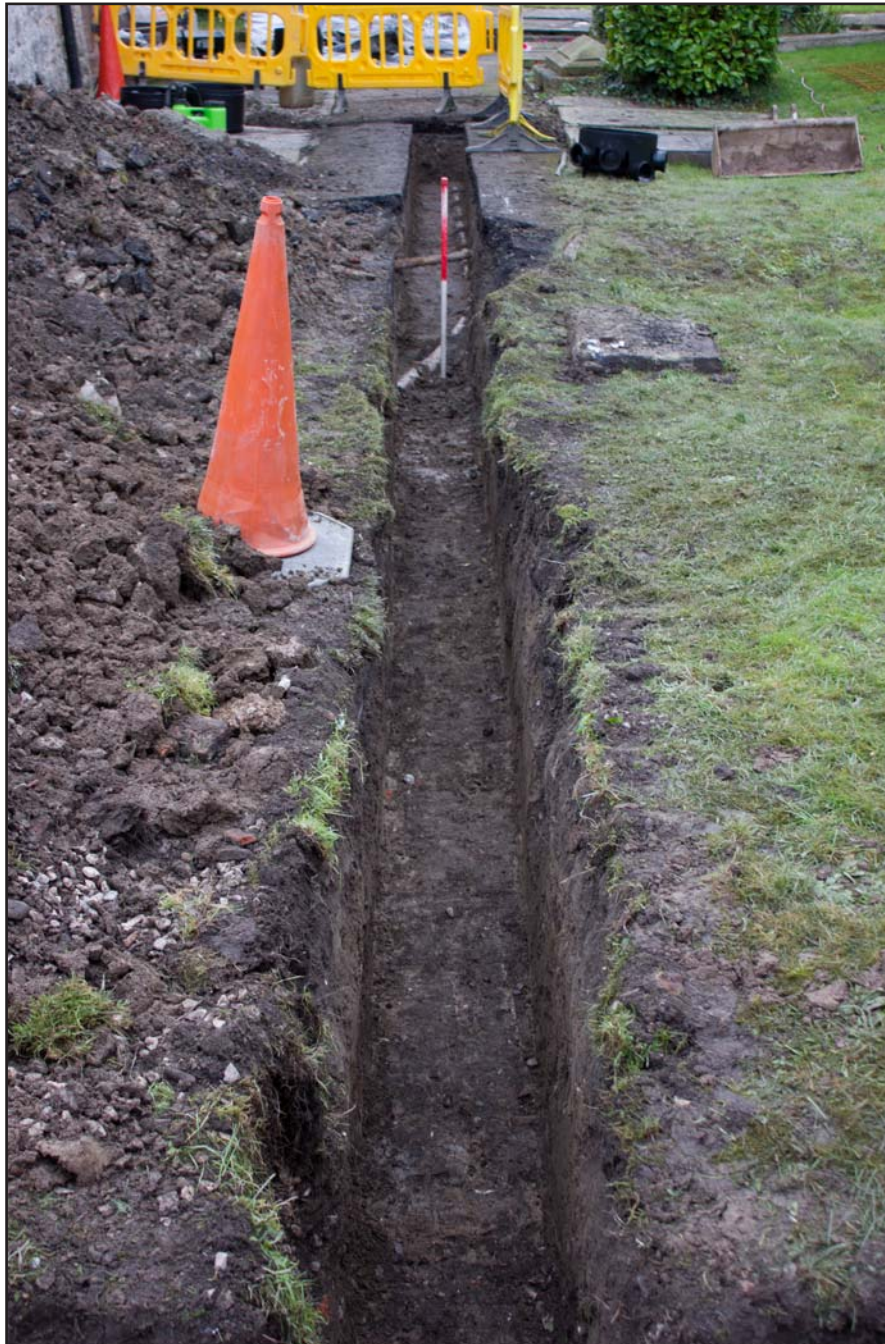
Plate 33: Main drainage trench to the west of St. Asaph Parish Church, St. Asaph, Denbighshire - from the north - scale 1m
