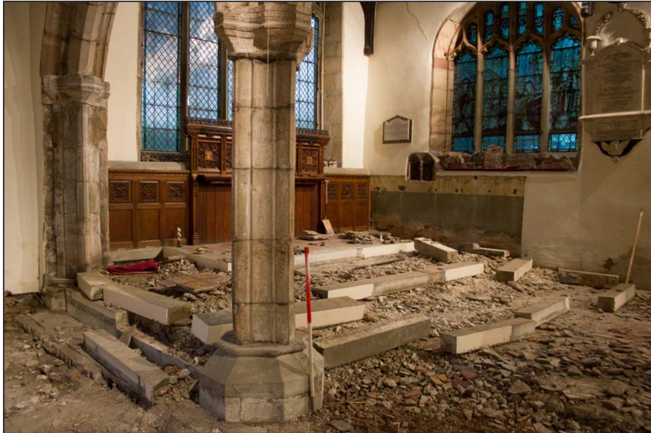
Plate 21: Pre removal of limestone kerbs at St. Asaph Parish Church, St. Asaph, Denbighshire - from the northwest - scale 1m
