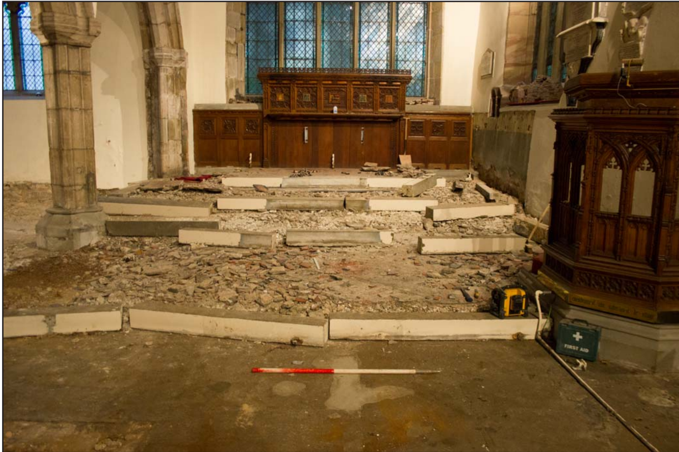
Plate 20: Pre removal of limestone kerbs at St. Asaph Parish Church, St. Asaph, Denbighshire - from the west - scale 1m
