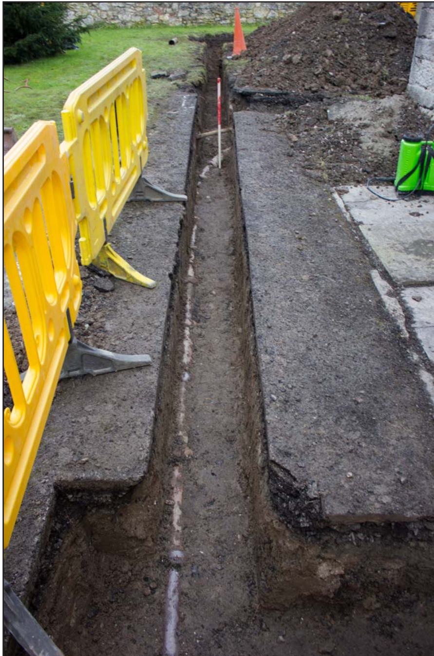
Plate 32: Main drainage trench to the west of St. Asaph Parish Church, St. Asaph, Denbighshire - from the south - scale 1m
