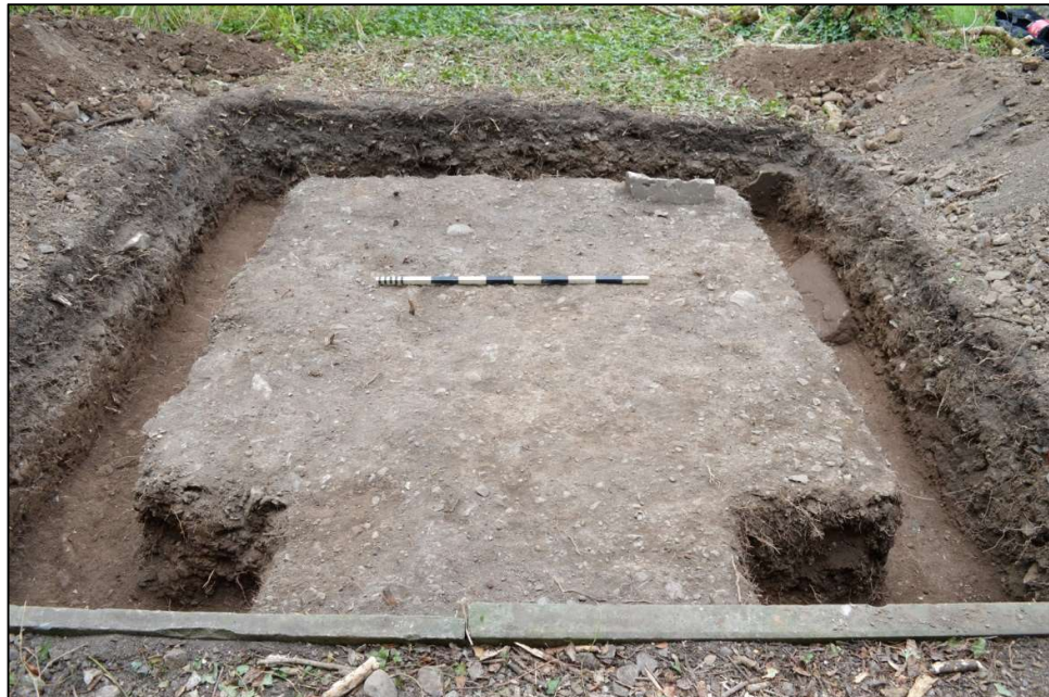
Fig. 7: The completed excavation of the extension foundations, viewed from the west. Photo CPAT 4928-0012
