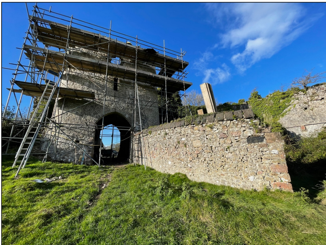
Plate 10. Inner wall topped with coppers slag coping stones and some copper slag blocks. View to NNW.
