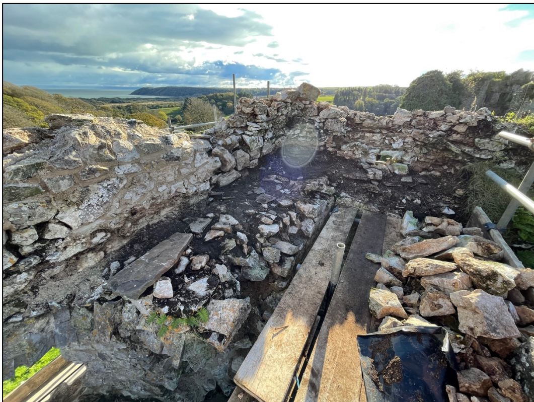
Plate 3. Wall walk (SW side) along the south eastern internal wall of the gatehouse during masonry conservation and prior to archaeological investigation.
