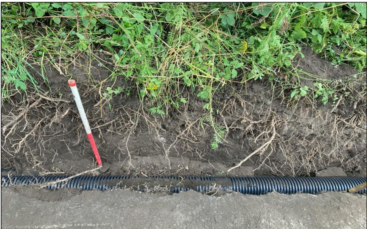
Plate 12. Representative section of excavations along roadway leading up Chapel Hill (south-facing section)
