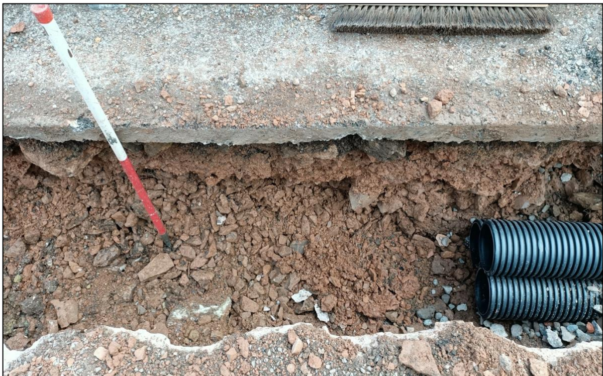
Plate 8. Representative section of excavations through pavement on north side of A466 (south-facing section)
