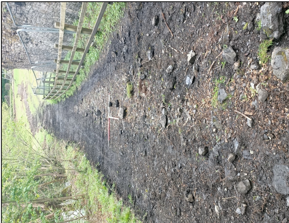
Plate 8. Downslope view of proposed pathway, after excavation, approaching base of hillslope to southwest of site (view northeast, scale 2x1m)
