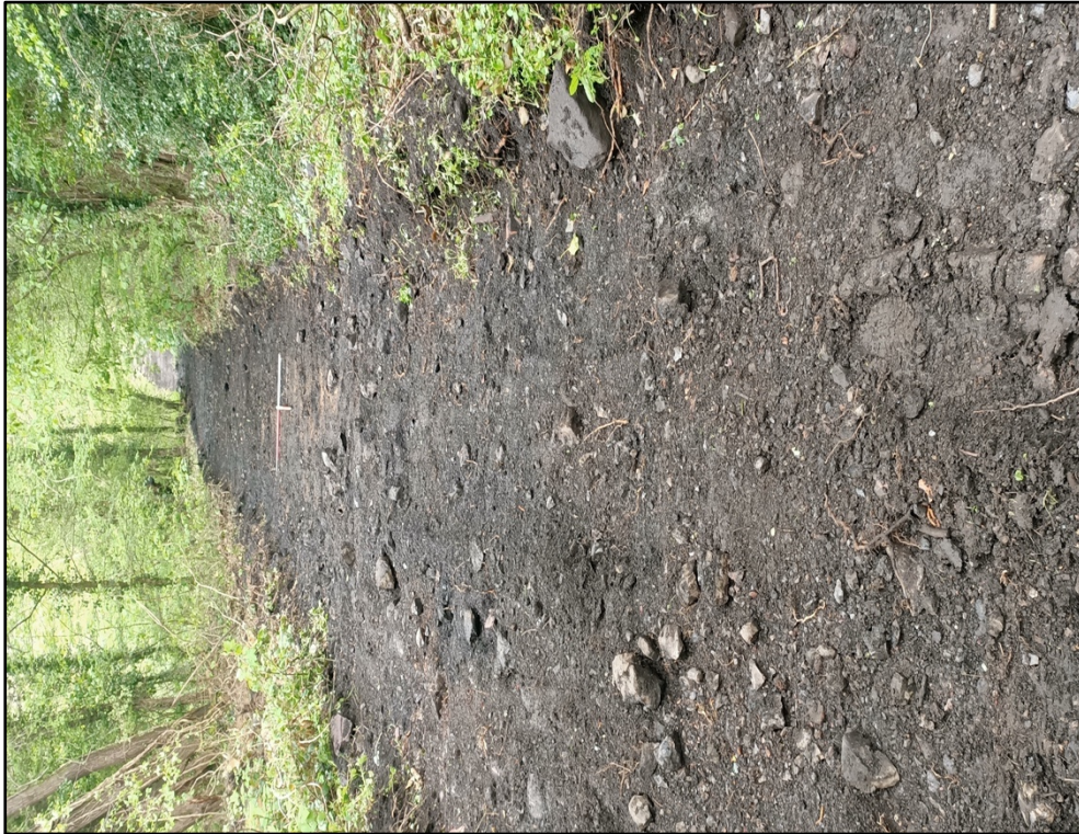
Plate 7. Downslope view of proposed pathway, after excavation, towards middle of hillslope to southwest of site (view northeast, scale 2x1m)
