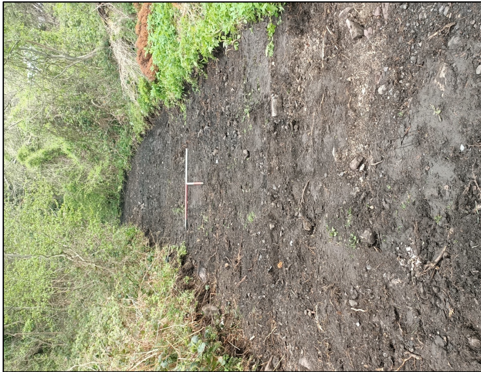
Plate 5. Upslope view of proposed pathway, after excavation, towards middle of hillslope to southwest of site (view southwest, scale 2x1m)
