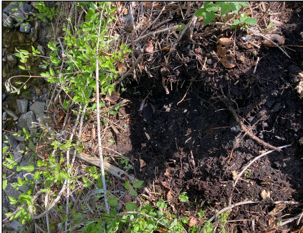
Plate 11. First test pit excavated in advance of construction of fence line to southwest of Smart's Bridge
