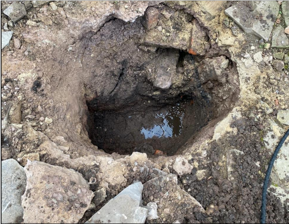
Plate 1. Plan view of Test Pit 1, with wall [102] running along its northern edge (view north)
