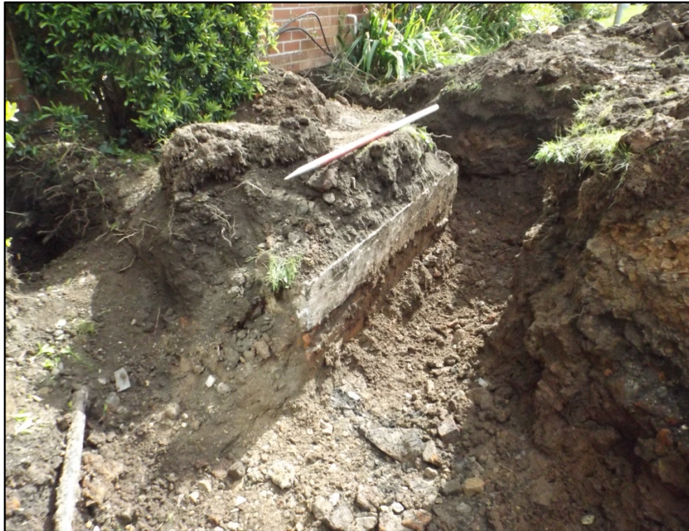
Plate 3. Oblique shot of inspection chamber [008] within the west-facing section of excavation area
