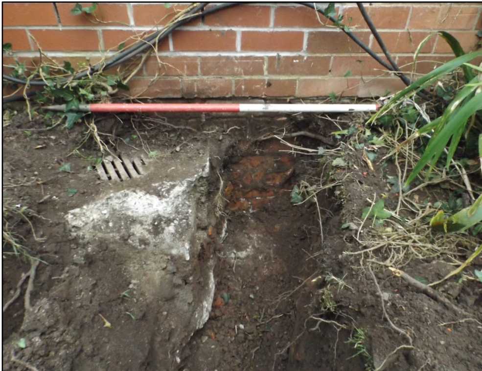
Plate 5. West-facing section towards east end of excavation area, showing wall foundation [011] and gully pot [009]
