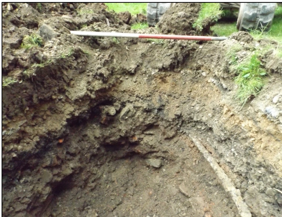
Plate 2. East-facing section towards western end of excavation area, showing cut [006], power cable [005] and fill (007)
