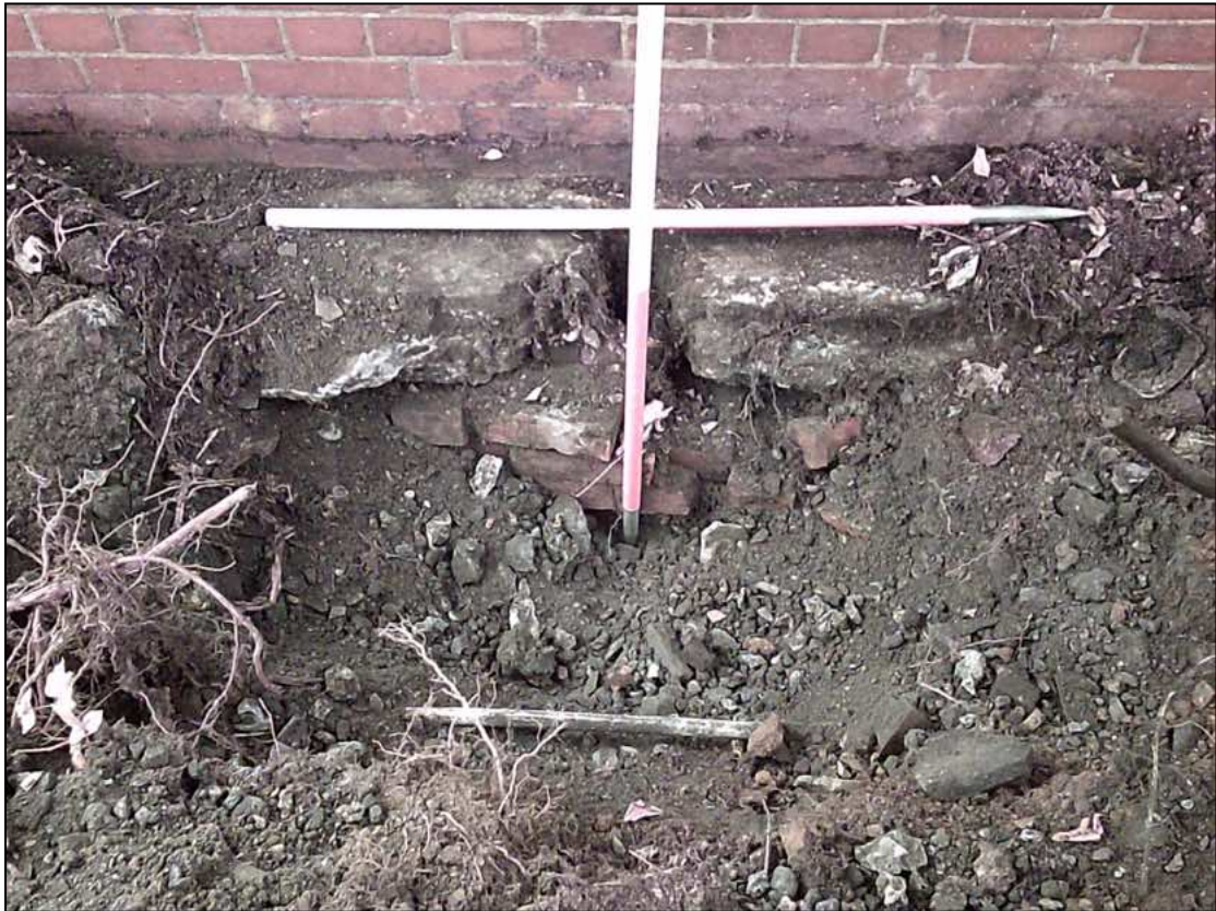
Plate 17. North facing section of Test Pit 12 showing foundation pier [1203] and concrete foundation slab [1202]. The in-situ lead pipe can be seen in the foreground.
