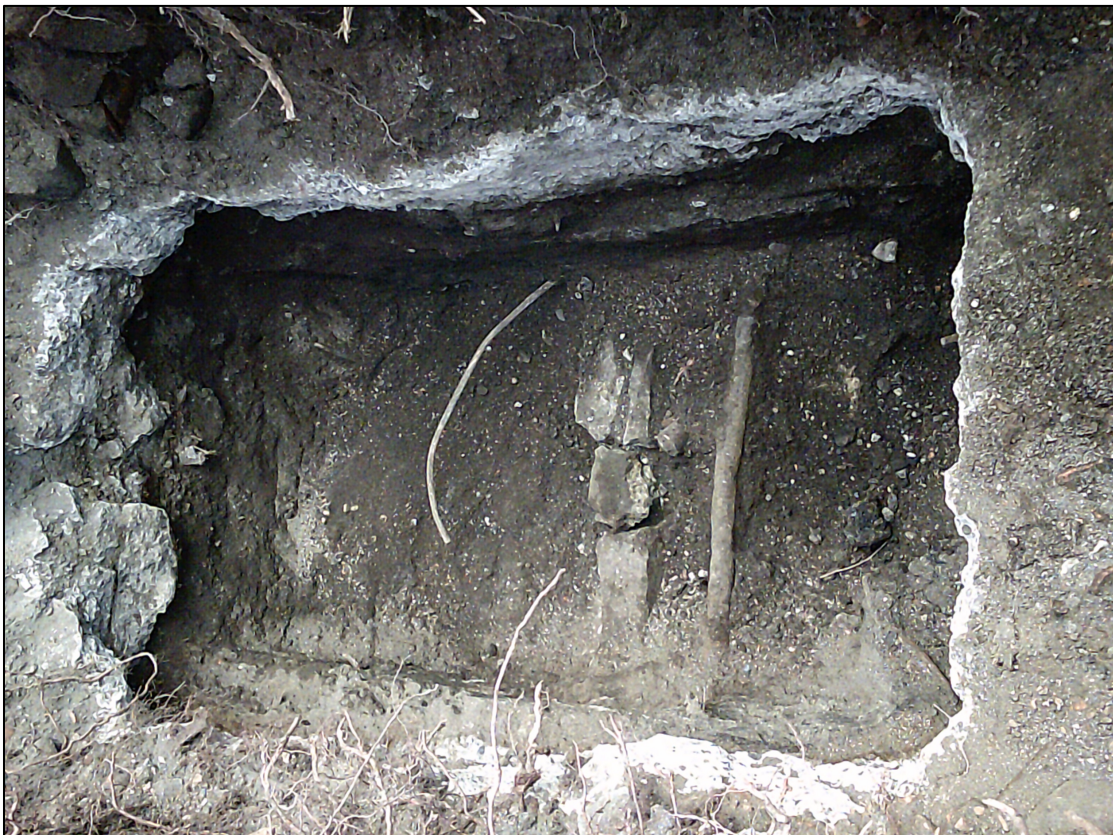
Plate 14. Plan view, facing east, showing in-situ lead service pipe, N/S aligned kerb and adjacent slag-rich deposit (1104).
