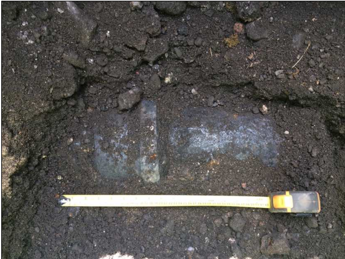
Plate 29. Large gauge NW/SE aligned metal water pipe uncovered in the base of Test Pit 15.
