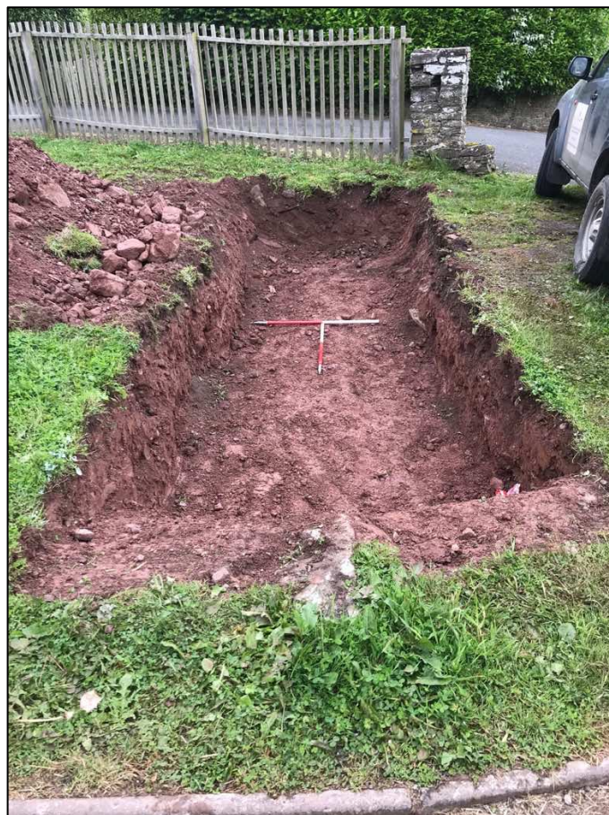
Plate 4. Trench 1, view W. Scale 1m in 0.5m sections. Note area of unexcavated gas main bottom of photograph.
