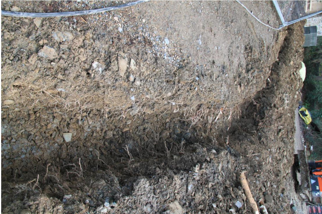
Plate 56 - AD010-D1-009 - Service trench 1 at top of bank and returning back towards the Former Coach House.
