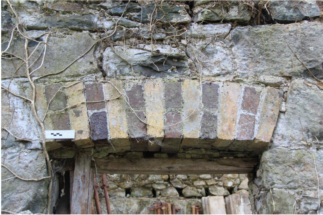
Plate 13 - AD010-BR-013 - Yellow and red brick flat segmental arch to window head, north elevation.
