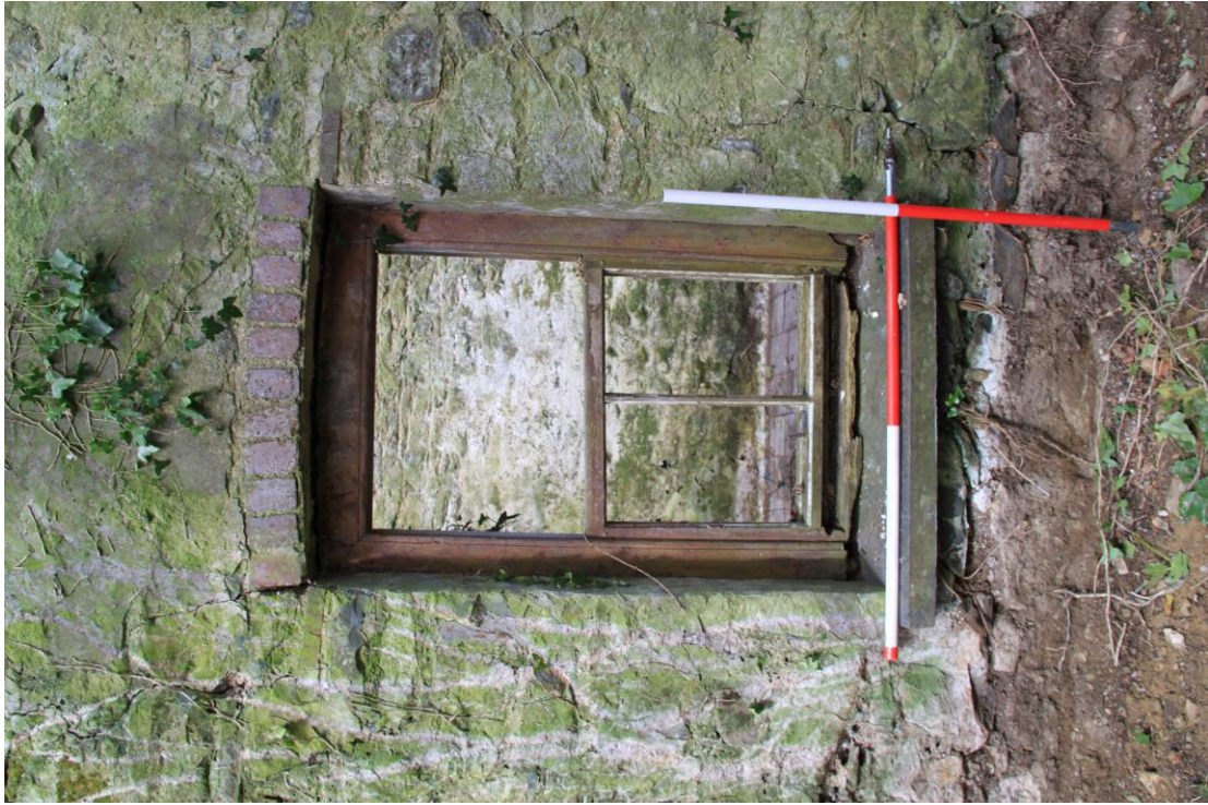
Plate 47 - AD010-BR-047 - Remains of four light box sash window, Extension A east elevation.
