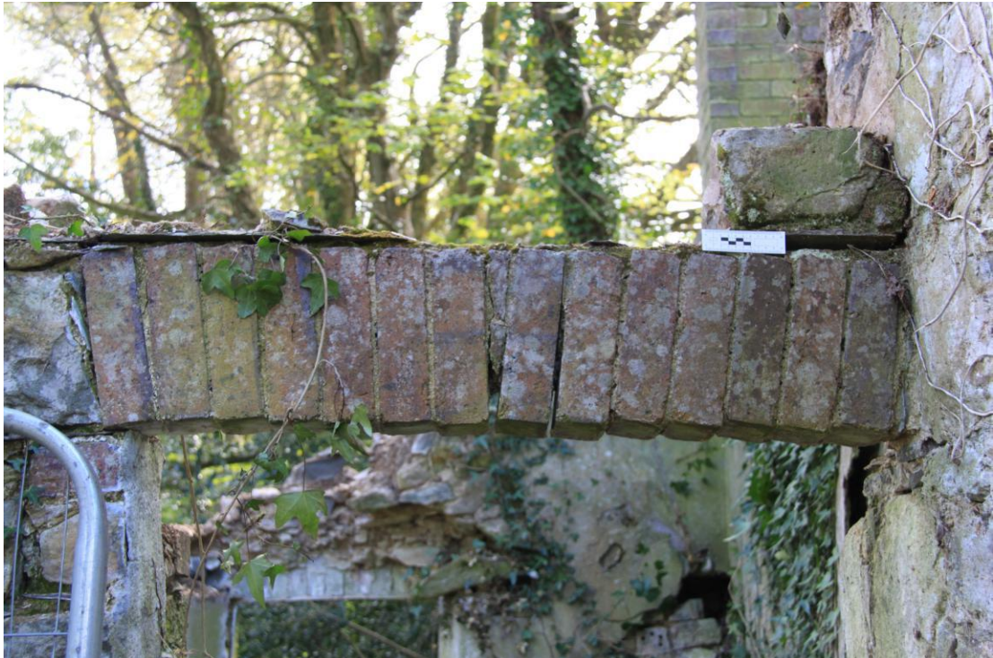
Plate 32 - AD010-BR-032 - Red brick flat arch door head to Extension B.
