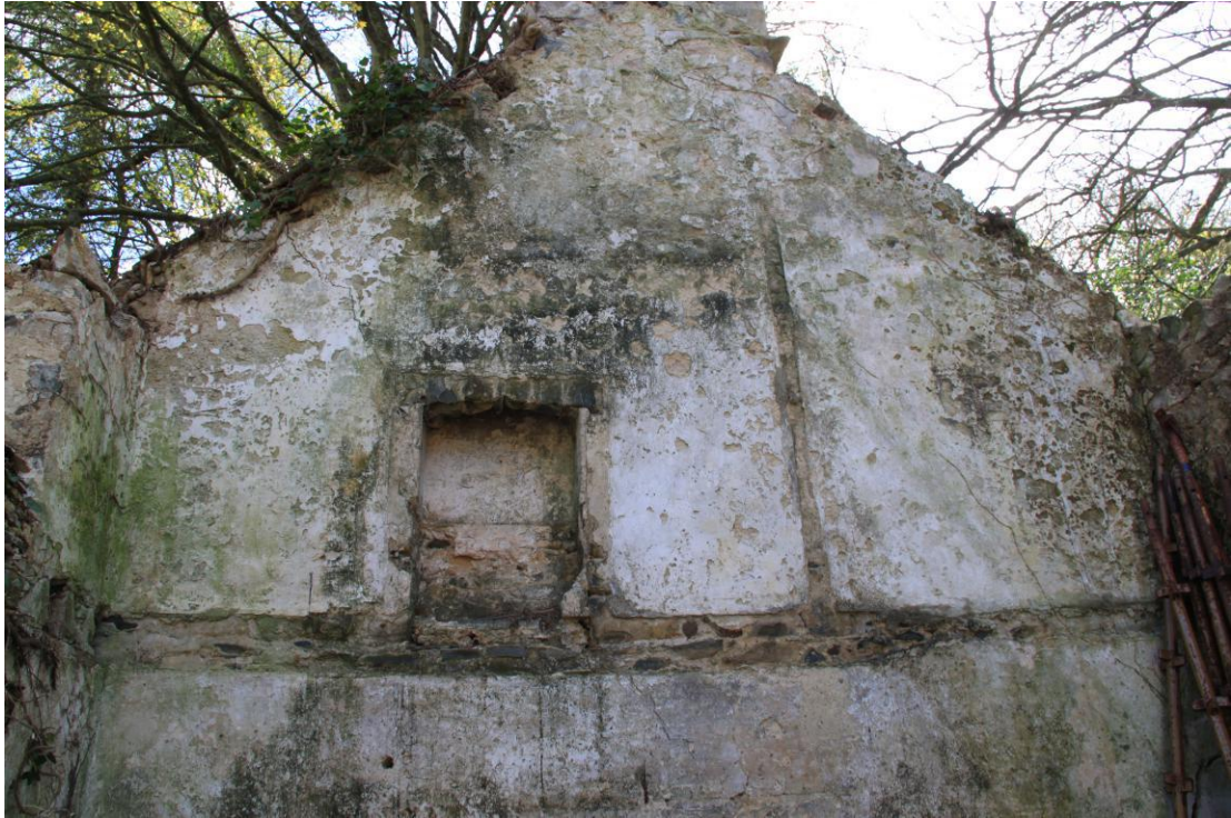
Plate 25 - AD010-BR-025 - First floor fireplace, internal east wall, Former Coach House. N.B. Partition division mark to plaster.
