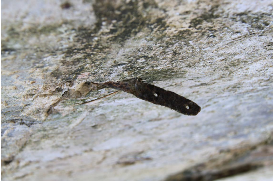
Plate 27 - AD010-BR-027 - Misc metal bracket, internal, north wall.
