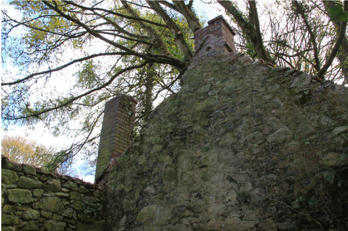
Plate 41 - AD010-BR-041 - Internal view of Extension B towards the east, showing chimney stacks.
