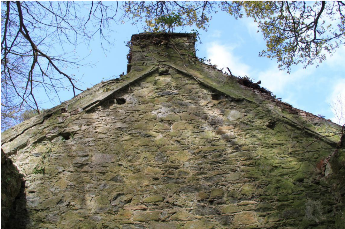
Plate 44 - AD010-BR-044 - Gable wall between Former Coach House and Extension A, showing two purlin and one ridge sockets.
