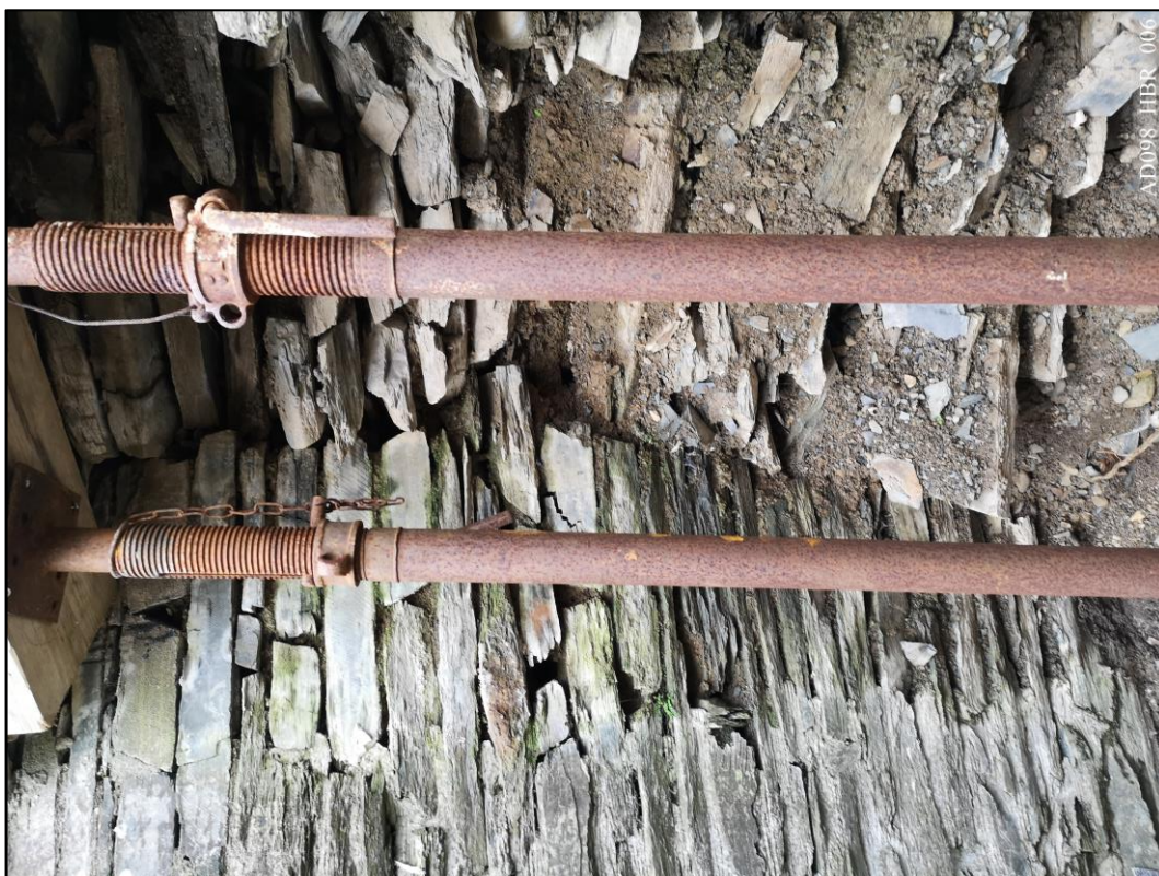
Plate 6 – View north-west, showing joint between modern retaining wall and historic core. Photo rotated 90° anticlockwise.
