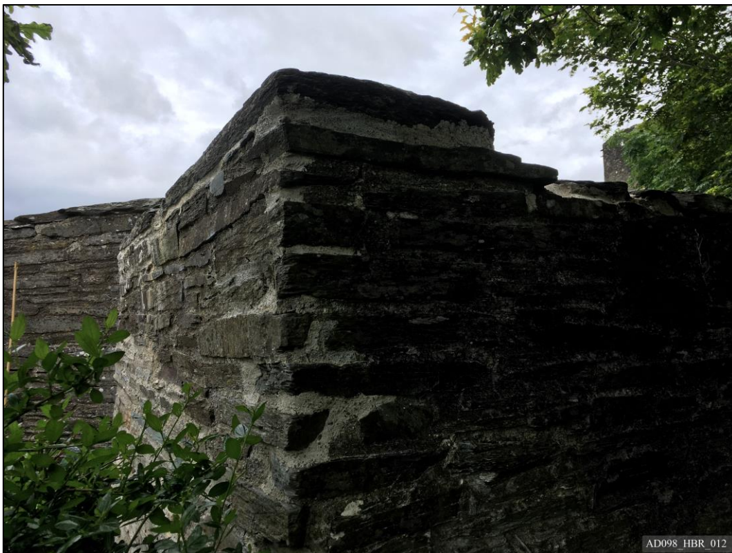
Plate 12 - View north-west, showing repair to south-west corner of retaining wall. Photo courtesy of Joseph Cliff, Cadw.
