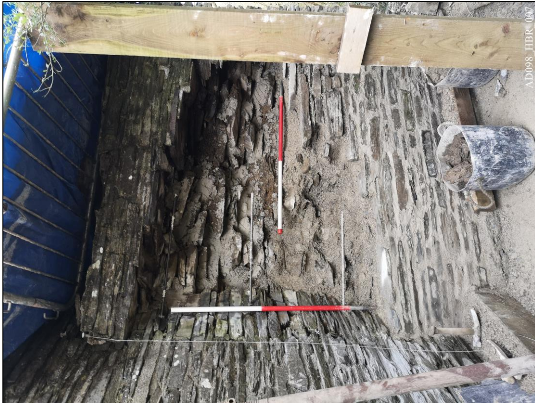
Plate 7 – View north, showing rebuilding of new retaining wall to historic core. Photo rotated 90° anticlockwise.
