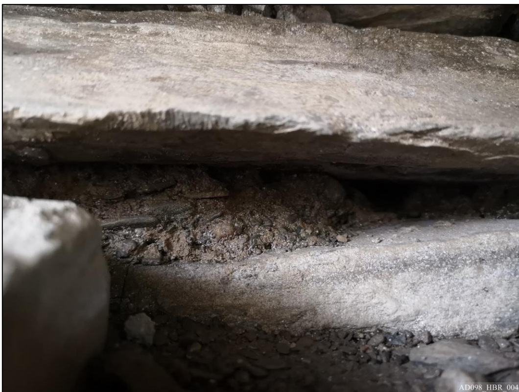
Plate 4 – View north, showing mortar in situ between coursed rubble fill of curtain wall core.
