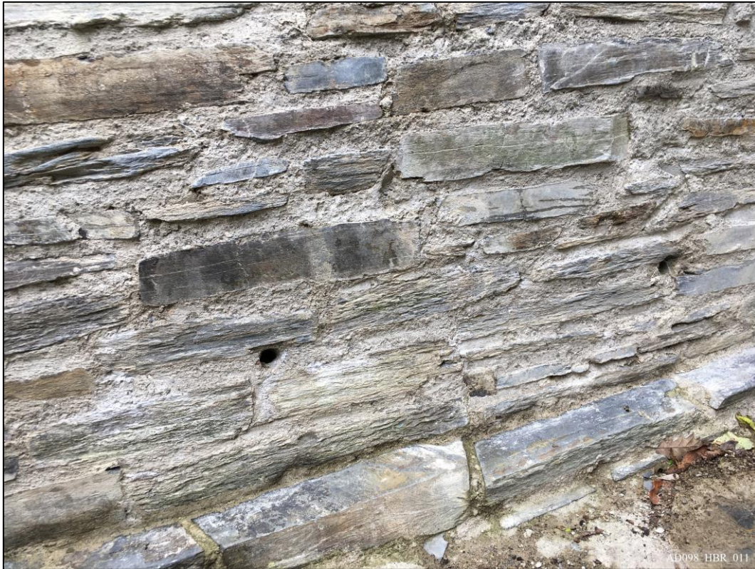
Plate 11 – View north, showing drainage holes to base of new retaining wall. Photo courtesy of Joseph Cliff, Cadw.
