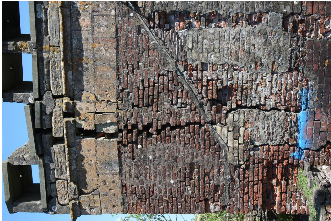
Plate 15 - AD042_WB_015 - West elevation, showing crack, caused by northern flue falling away.
