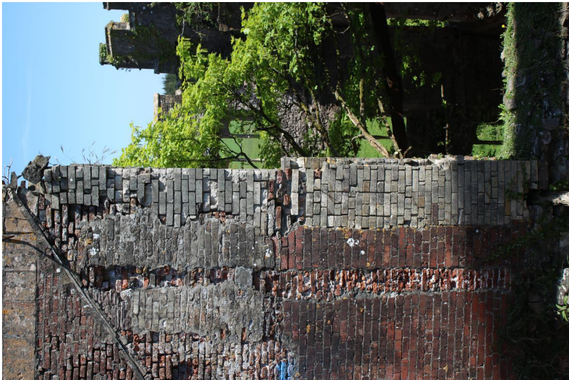
Plate 14 - AD042_WB_014 - West elevation, showing later inserted/added brickwork (white brick) for additional fireplace and flue; and former wall scar.
