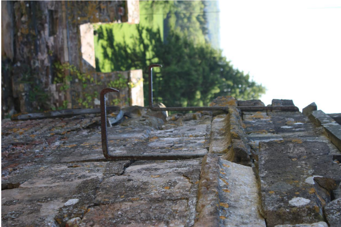
Plate 35 - AD042_WB_035 - East elevation, showing iron hook/strap.
