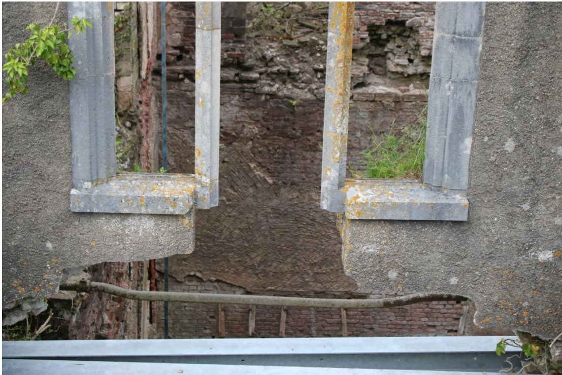
Plate 123 - AD042_WB_123 - South window exterior, showing sills and fallen masonry.
