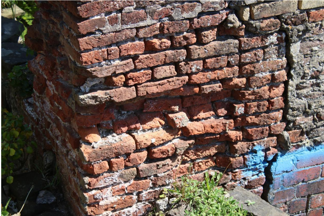
Plate 25 - AD042_WB_025 - West elevation, showing pinch spalling.
