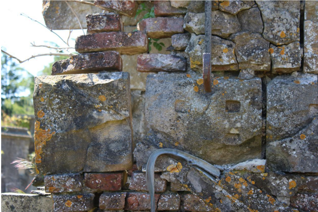
Plate 49 - AD042_WB_049 - East elevation, showing collapsing masonry and later lead flashing to 1783 roofline.
