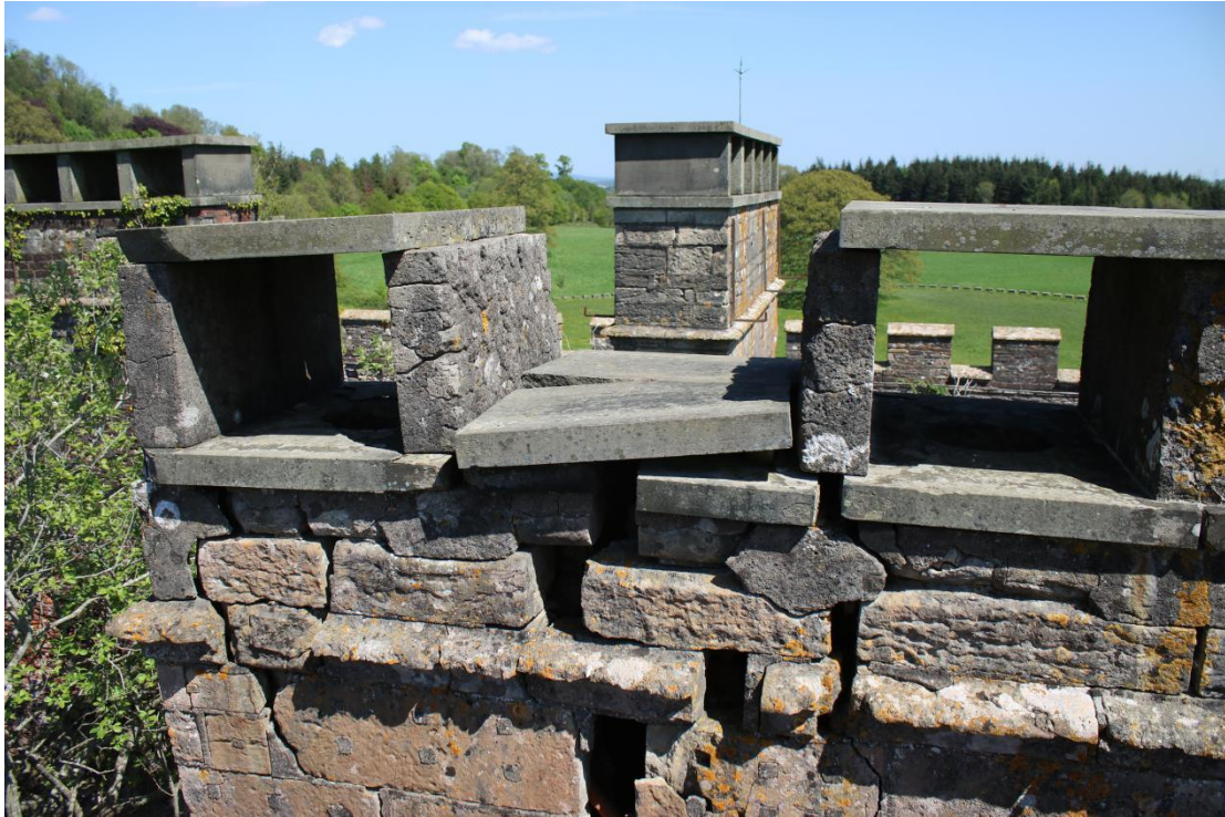
Plate 21 - AD042_WB_021 - West elevation, showing capstones and flue stones, with cast concrete uprights.
