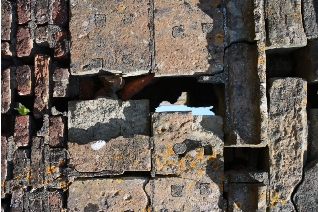
Plate 19 - AD042_WB_019 - West elevation, showing crack to sandstone ashlars opening through to east elevation.
