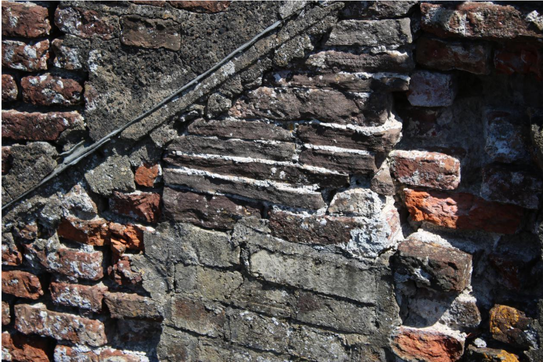
Plate 11 - AD042_WB_011 - West elevation, showing lead flashing and limestone and later brick patch-repair.
