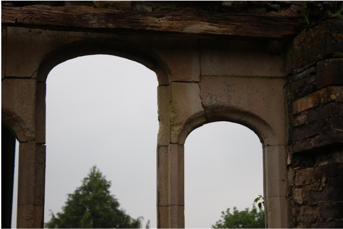
Plate 131 - AD042_WB_131 - South window interior, showing showing deteriorated sandstone window head, west.
