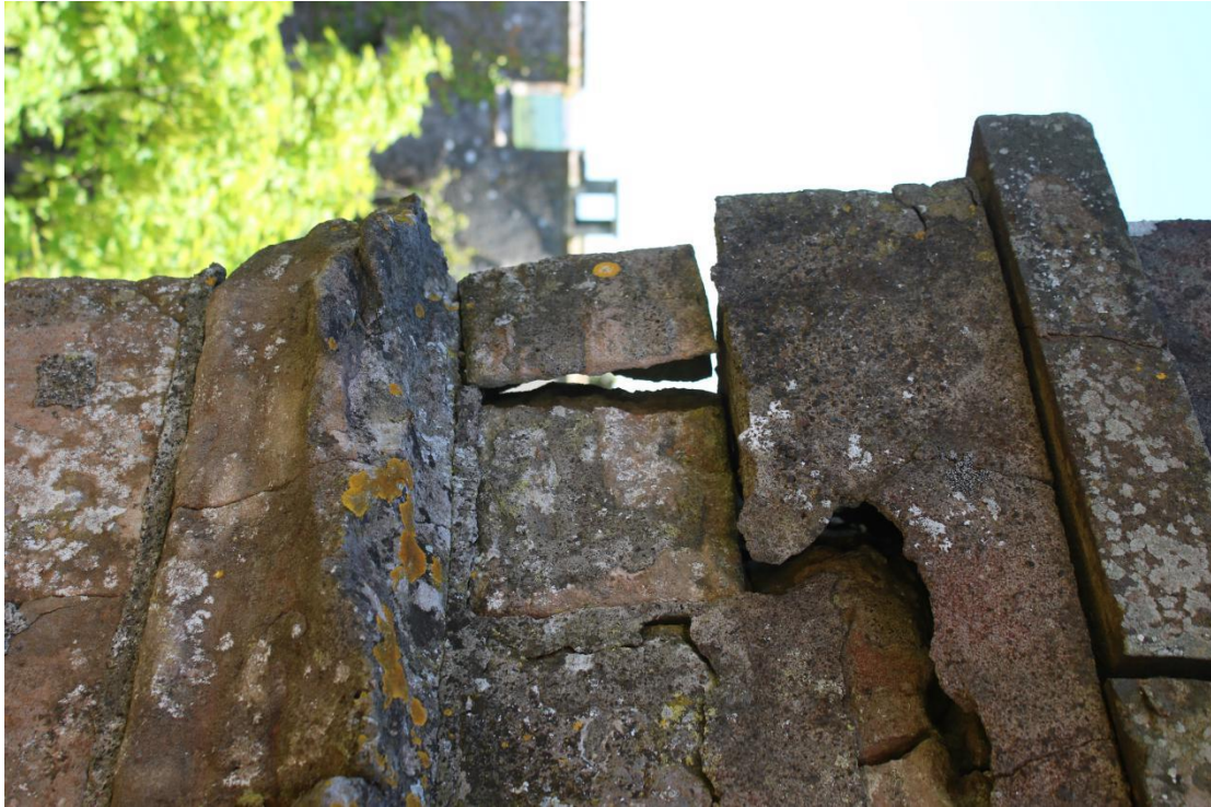
Plate 31 - AD042_WB_031 - North elevation, showing decayed sandstone ashlar with cementitious mortar above.
