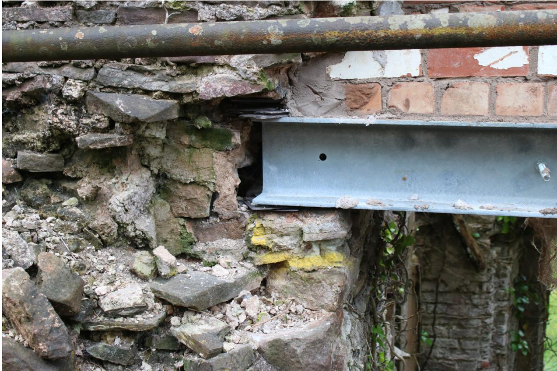
Plate 140 - AD042_WB_140 - South window, showing temporary RSJ siting and masonry to be removed.
