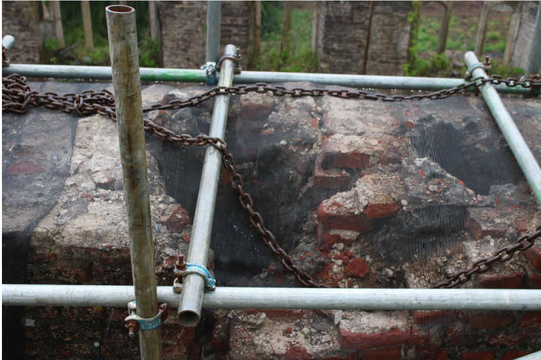
Plate 115 - AD042_WB_115 - Chimney after removal of row 8, showing flue 2 and area of lost brickwork.
