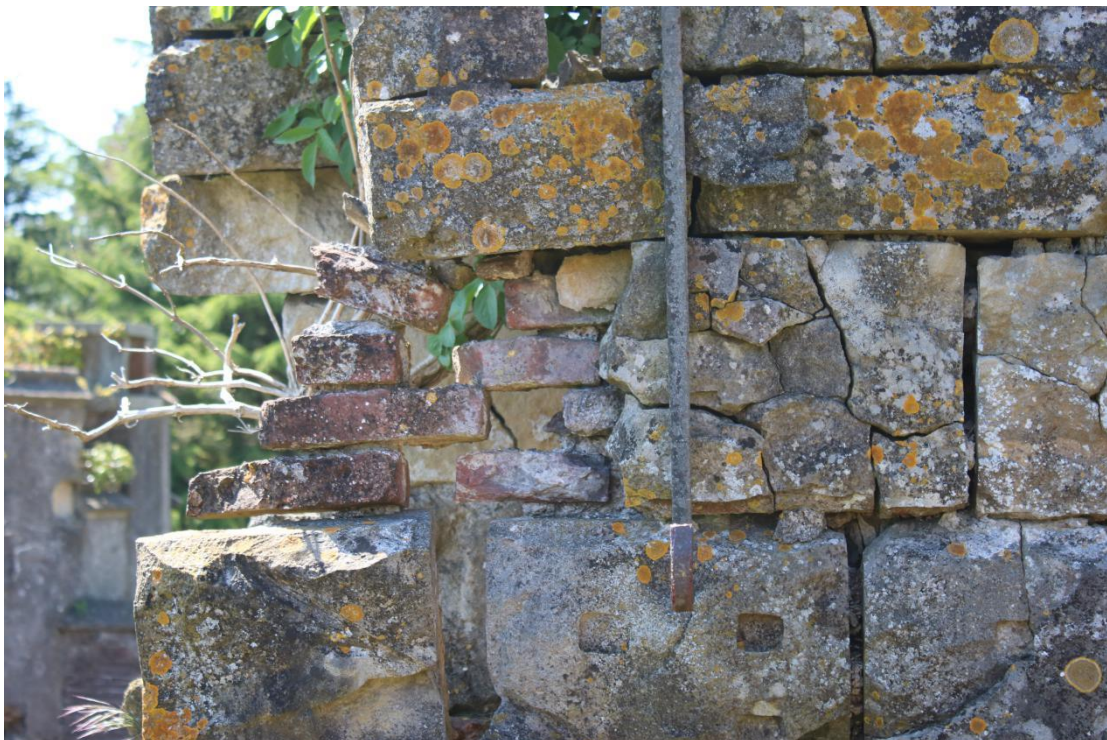
Plate 50 - AD042_WB_050 - East elevation, showing brickwork supporting upper masonry to south end of east elevation.
