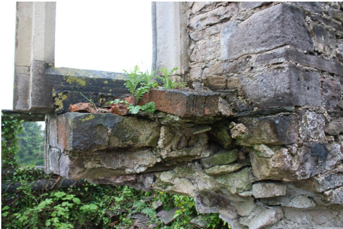
Plate 142 - AD042_WB_142 - South window interior, showing hanging masonry.
