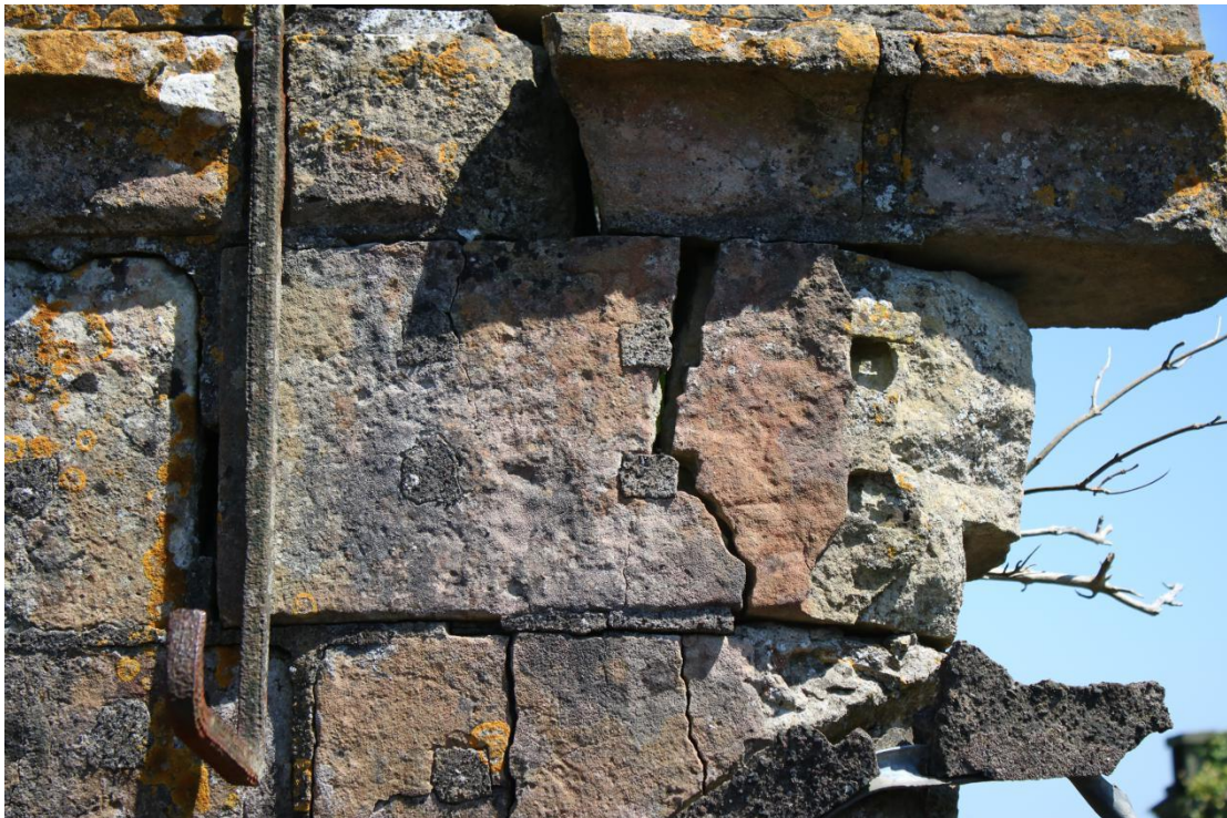
Plate 8 - AD042_WB_008 - West elevation, showing damaged sandstone ashlar.
