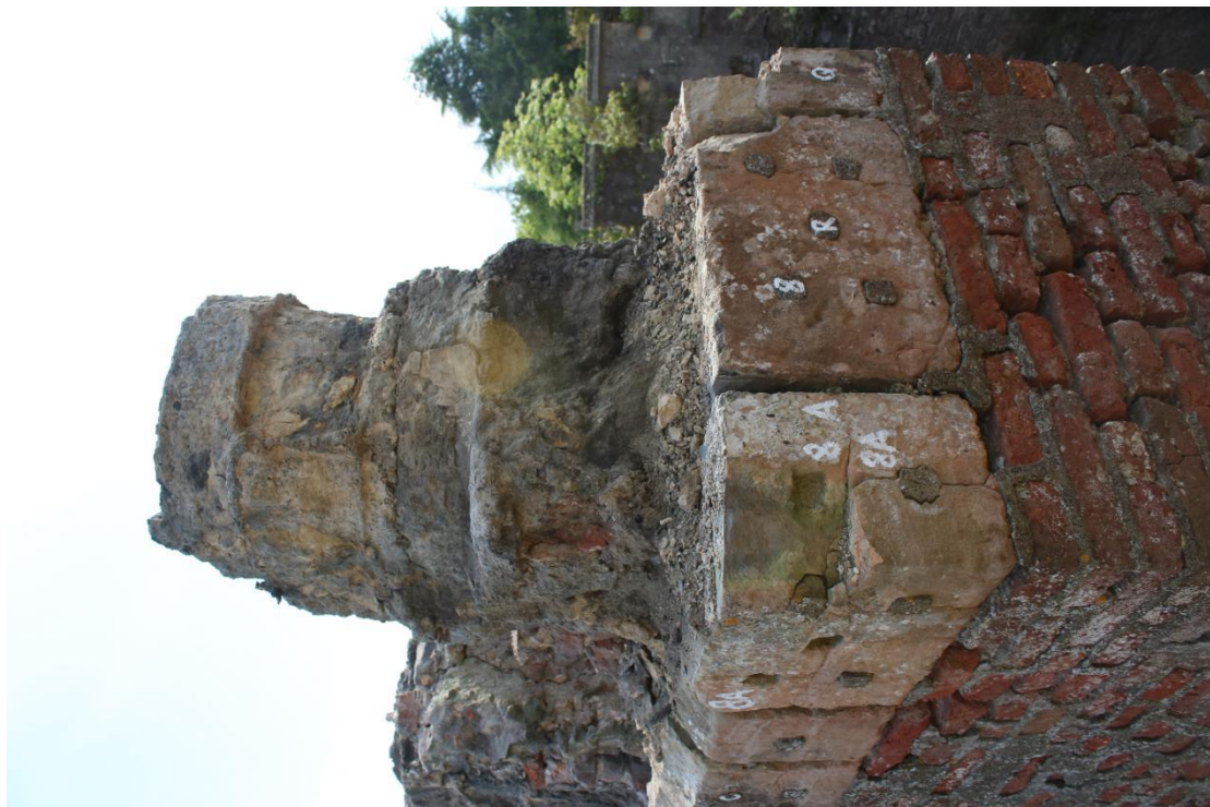
Plate 80 - AD042_WB_080 - Chimney after removal of row 7, showing north cementitious mortar lined flue 1.
