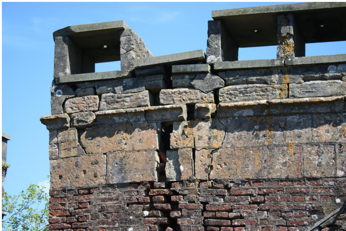
Plate 16 - AD042_WB_016 - West elevation, showing crack, caused by northern flue falling away.
