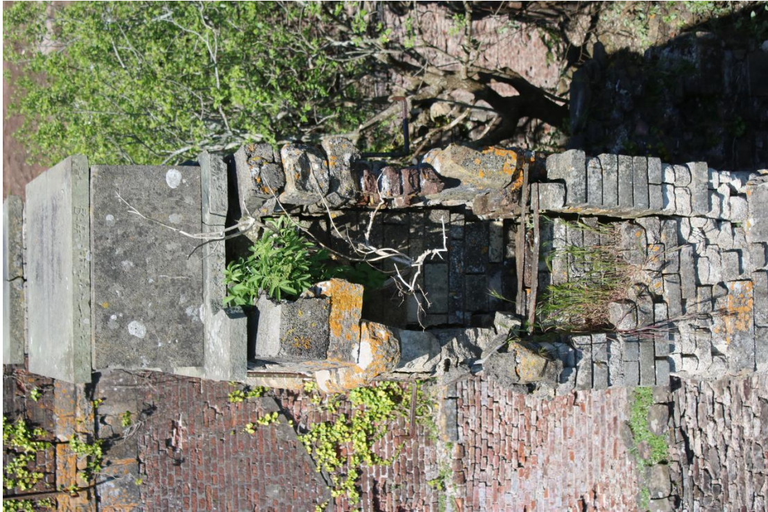
Plate 3 - AD042_WB_003 - South chimney elevation, showing top of flue, caused by partial collapse of brickwork.
