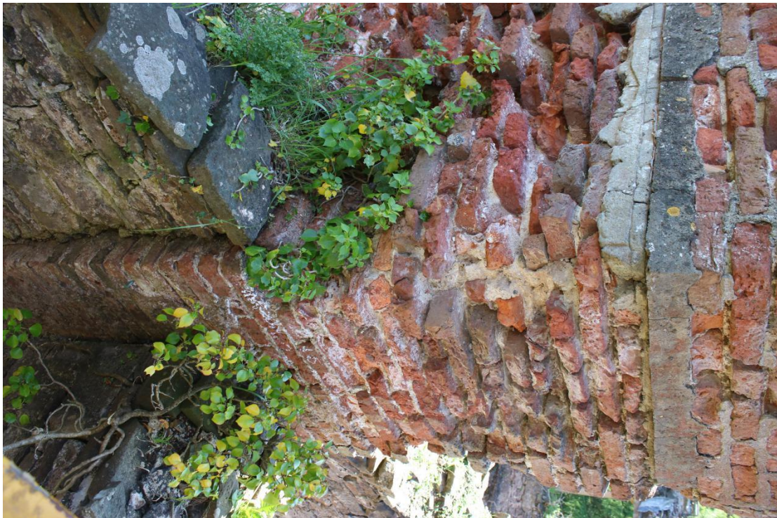
Plate 36 - AD042_WB_036 - 3/4 view of north and east elevations, showing pinch spalling and flashing line to former roof.
