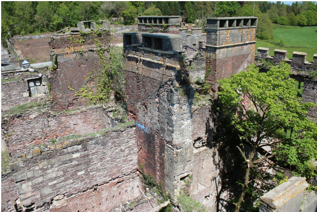
Plate 2 - AD042_WB_002 - 3/4 view showing chimney in relation to north, east and west chimneys.
