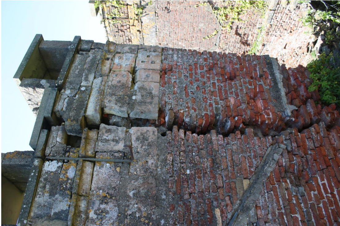
Plate 47 - AD042_WB_047 - East elevation, showing crack and flashing line to 1783 roof.
