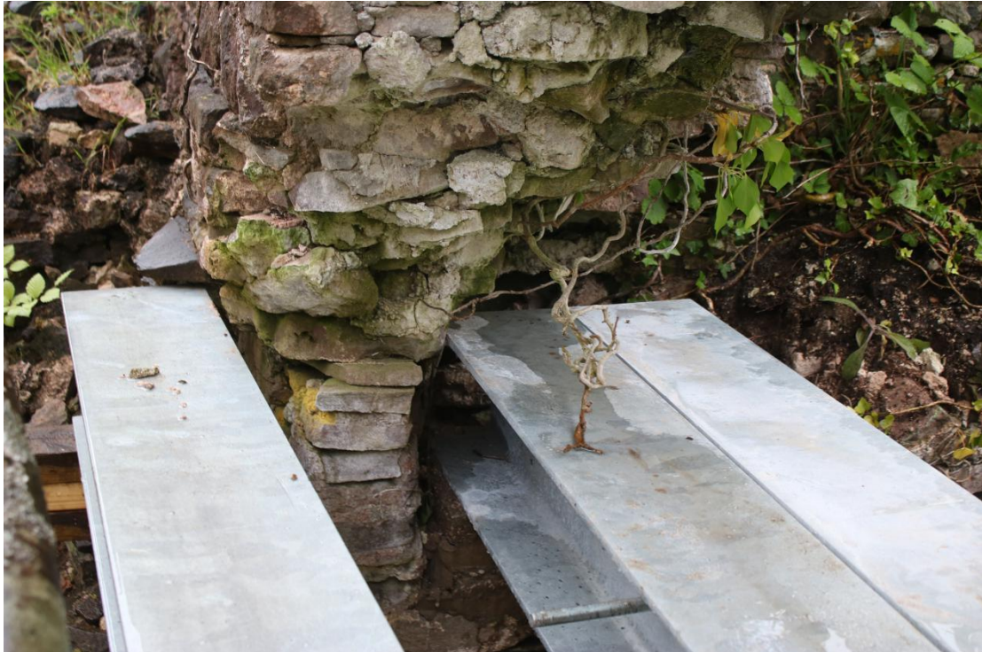
Plate 139 - AD042_WB_139 - South window, showing temporary RSJ siting and masonry to be removed.
