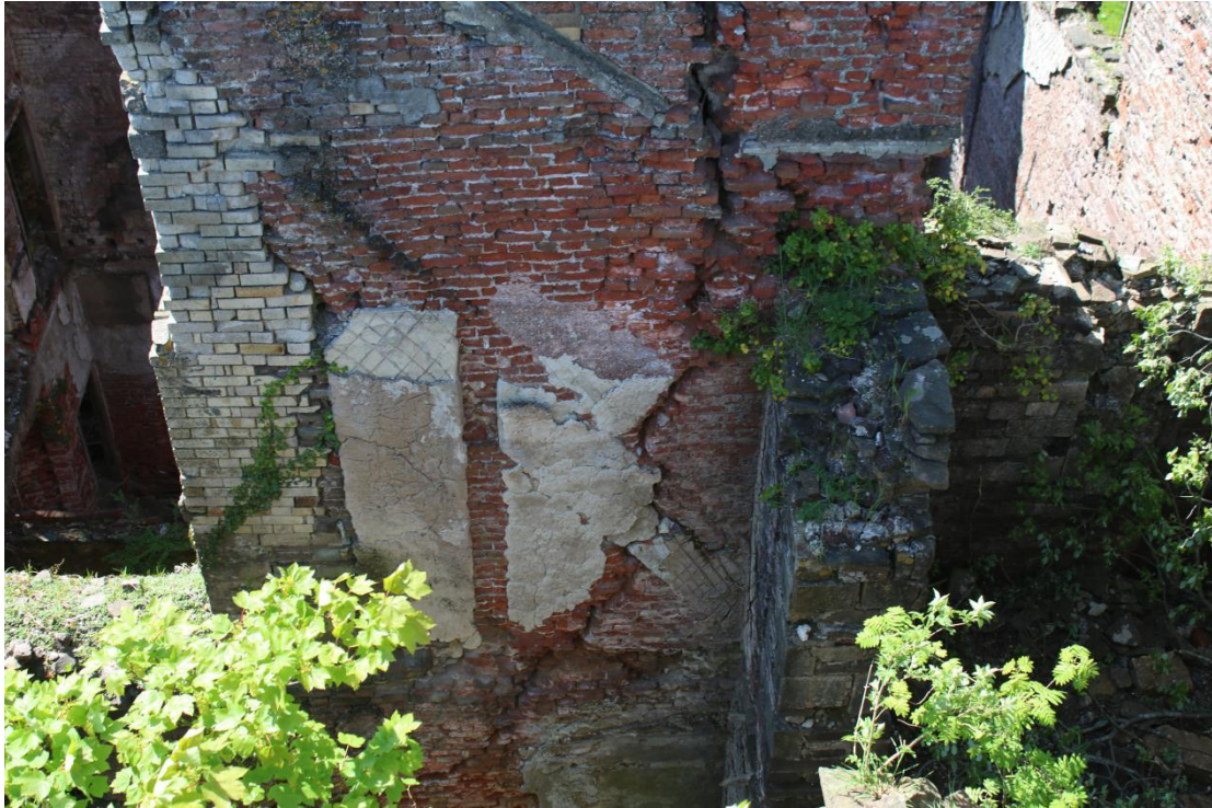
Plate 41 - AD042_WB_041 - East elevation, showing 1626 roofline, patches of lime plaster, crack and later inserted flue (white brick).
