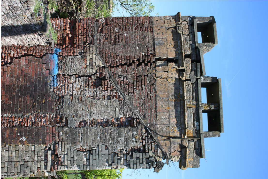
Plate 13 - AD042_WB_013 - West elevation, showing initial area to be dismantled (to blue line).
