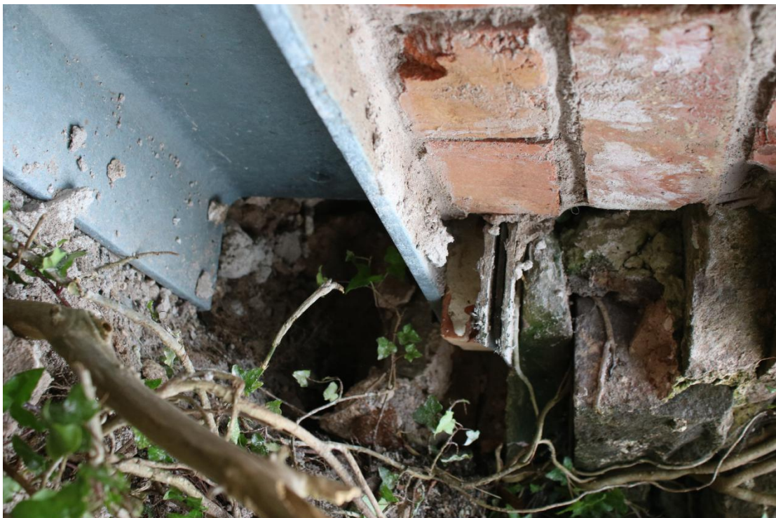
Plate 141 - AD042_WB_141 - South window, showing temporary RSJ siting and masonry to be removed.
