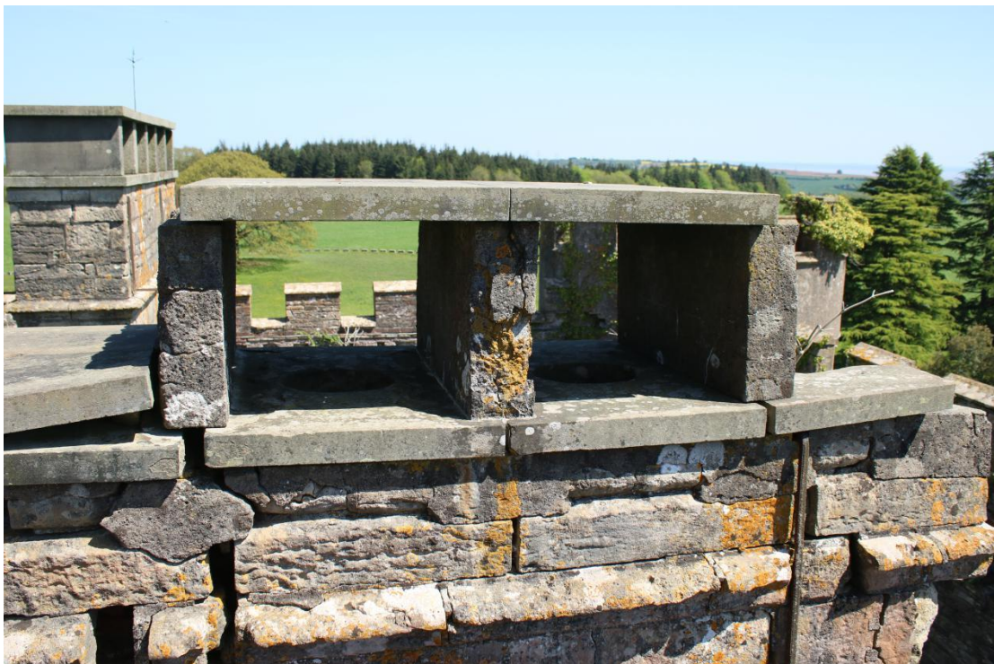
Plate 20 - AD042_WB_020 - West elevation, showing capstones and flue stones, with cast concrete uprights.
