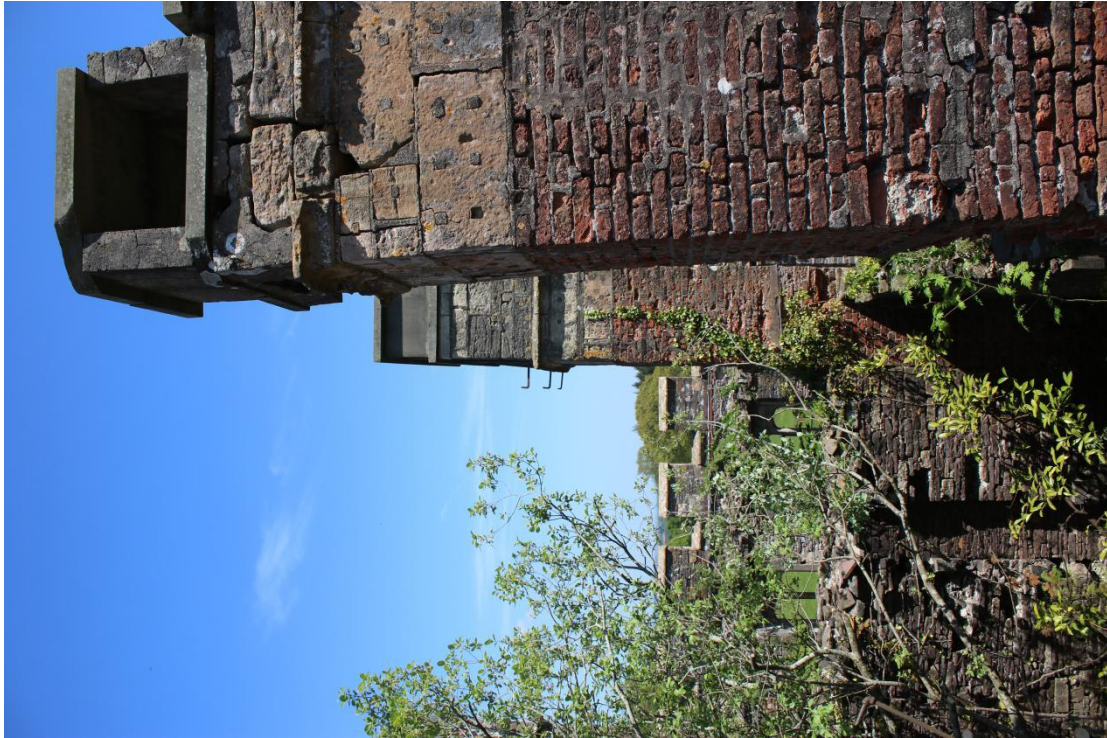
Plate 27 - AD042_WB_027 - West elevation, showing fall of the north flue from plumb.
