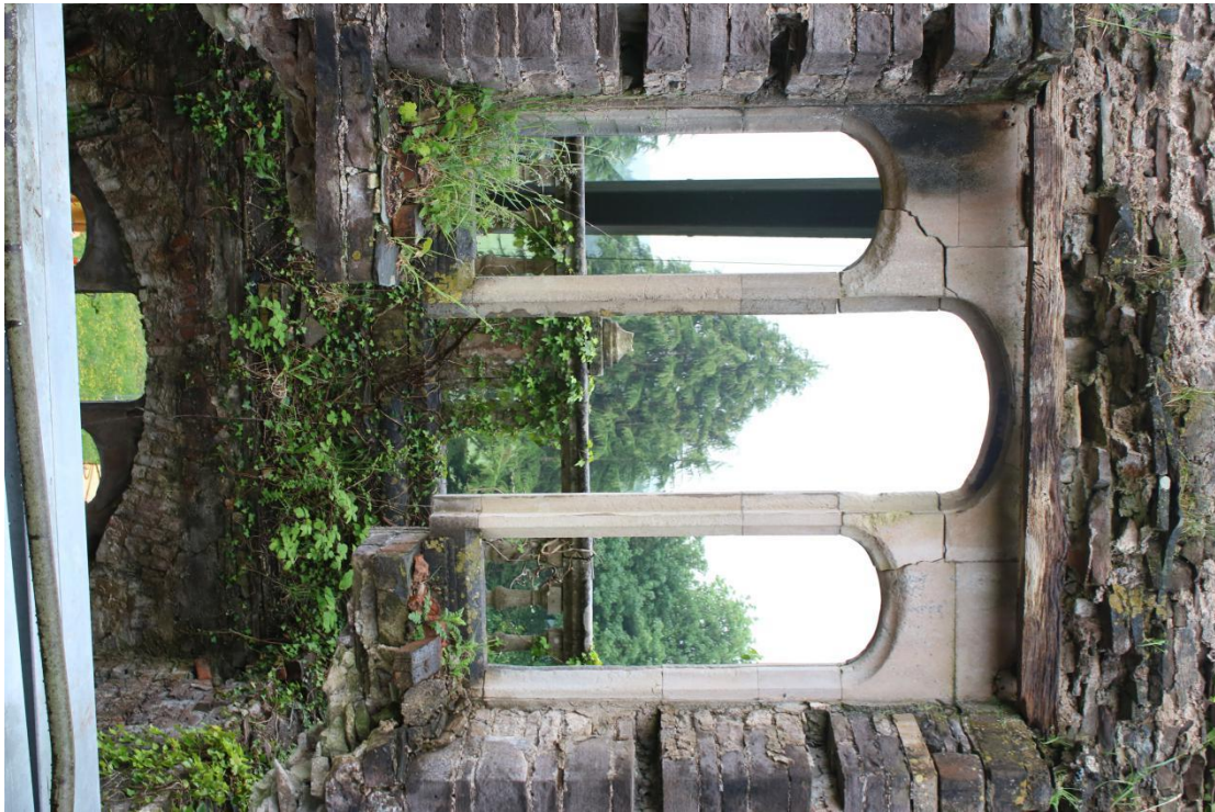
Plate 129 - AD042_WB_129 - South window interior, showing hanging masonry.
