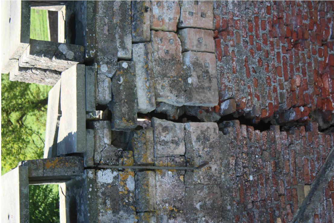
Plate 43 - AD042_WB_043 - East elevation, showing crack.
