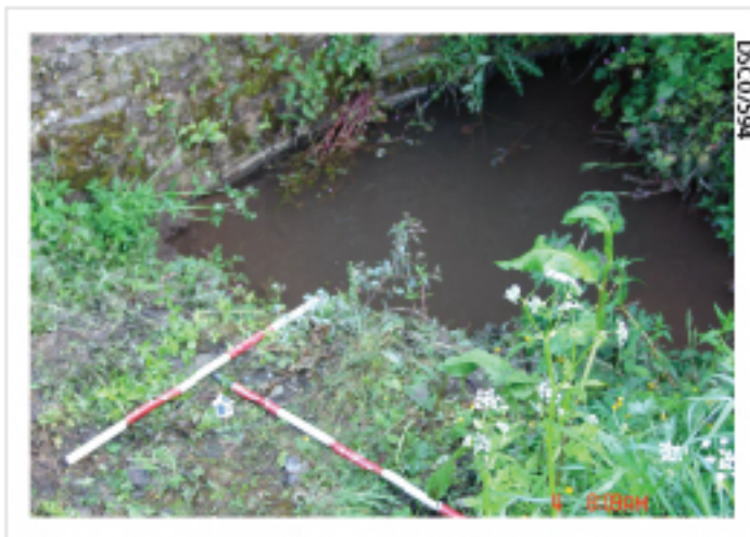
Plate 06: Culvert beside cottage showing level of water (WB/JB/10).
