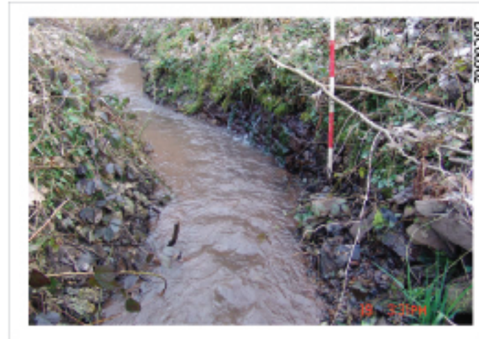
Plate 23: Curved walling of culvert, south bank and just south of stream join
