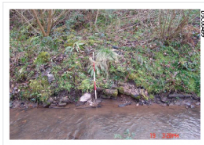
Plate 24: Culvert drystone wall with section of mortared wall above and at angle
