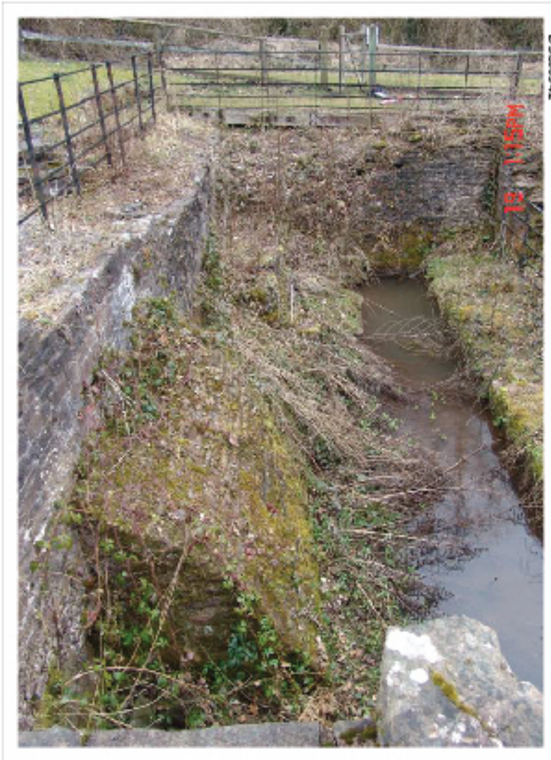
Plate 07: Wheelpit waterlevel, mid March 2010. Inflow submerged
