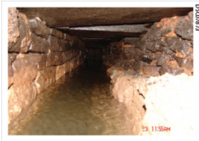
Plate 36: Beyond silt remains at the cottage outfall culvert.
