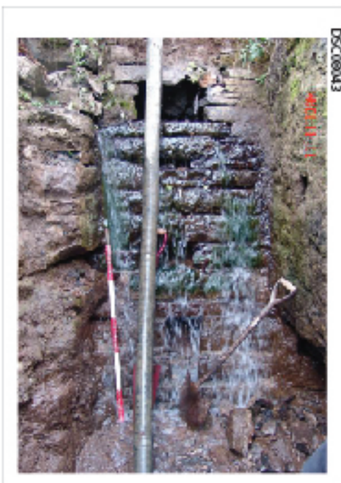
Plate 52: Stream side of wheelpit showing water ingress, river sandbagged
