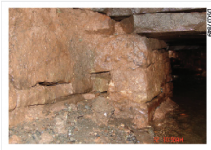
Plate 29: Close up of butt joint to south west wall of culvert, beyond the mortared arch
