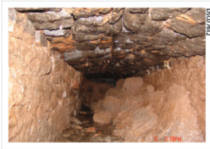
Plate 05: Culvert beside cottage showing level of silt (WB/JB/10).
