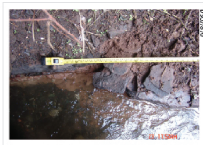
Plate 34: Upstream butt joint to culvert below outflow. Curved construction to reduce turbulent water flow and erosion.
