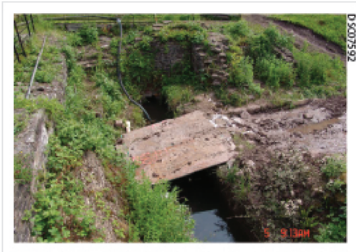
Plate 49: Silt dump at the wheel pit
