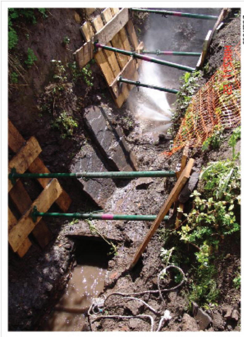
Plate 10: Further jetting attempt in Cottage outfall, culvert
