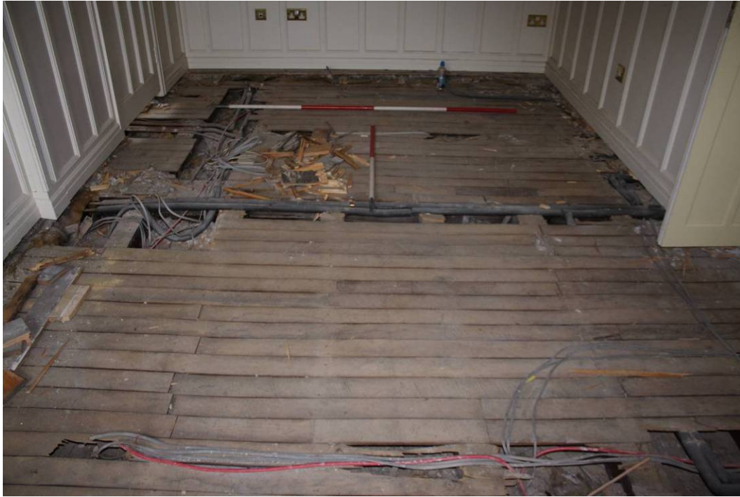
Photo 25: Room 103 looking NE following removal of floorboards and exposure of underlying wooden slats
