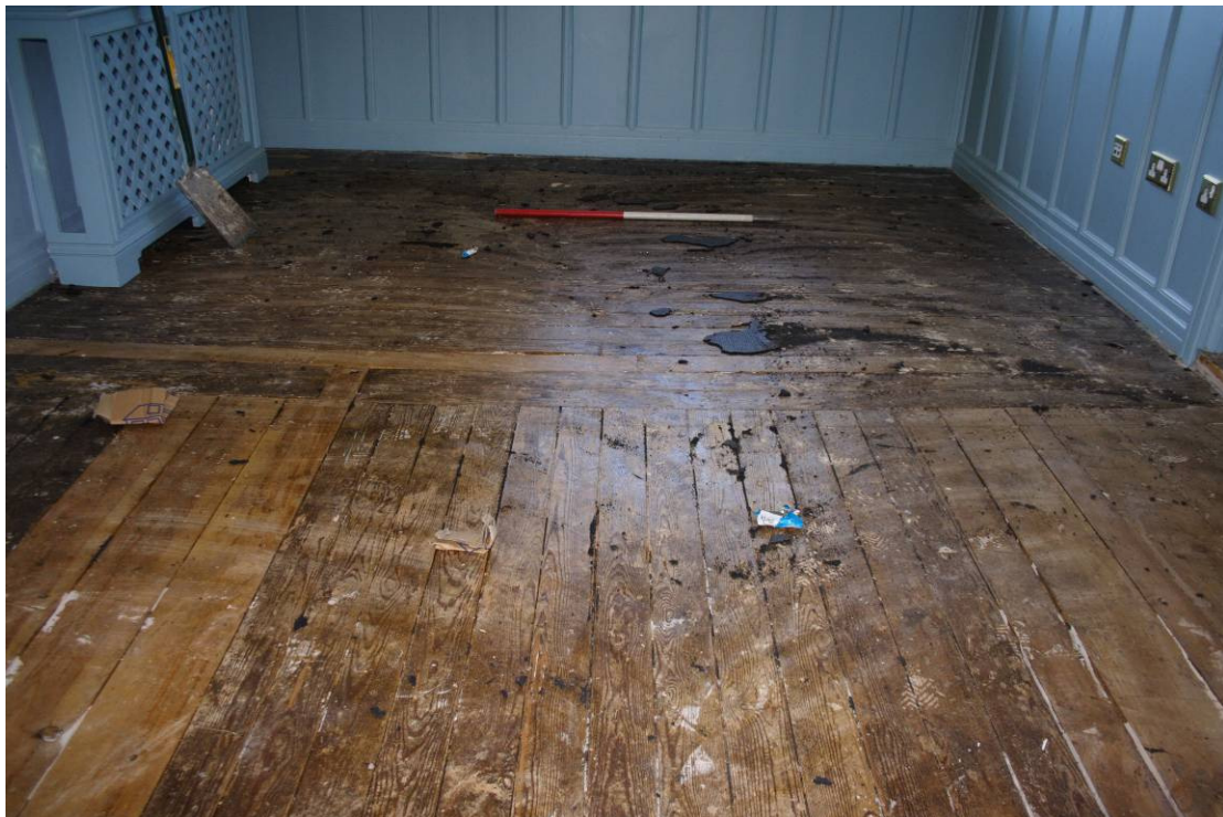
Photo 27: Room 105 viewing SW prior to removal of floorboards, showing change in floorboard direction
