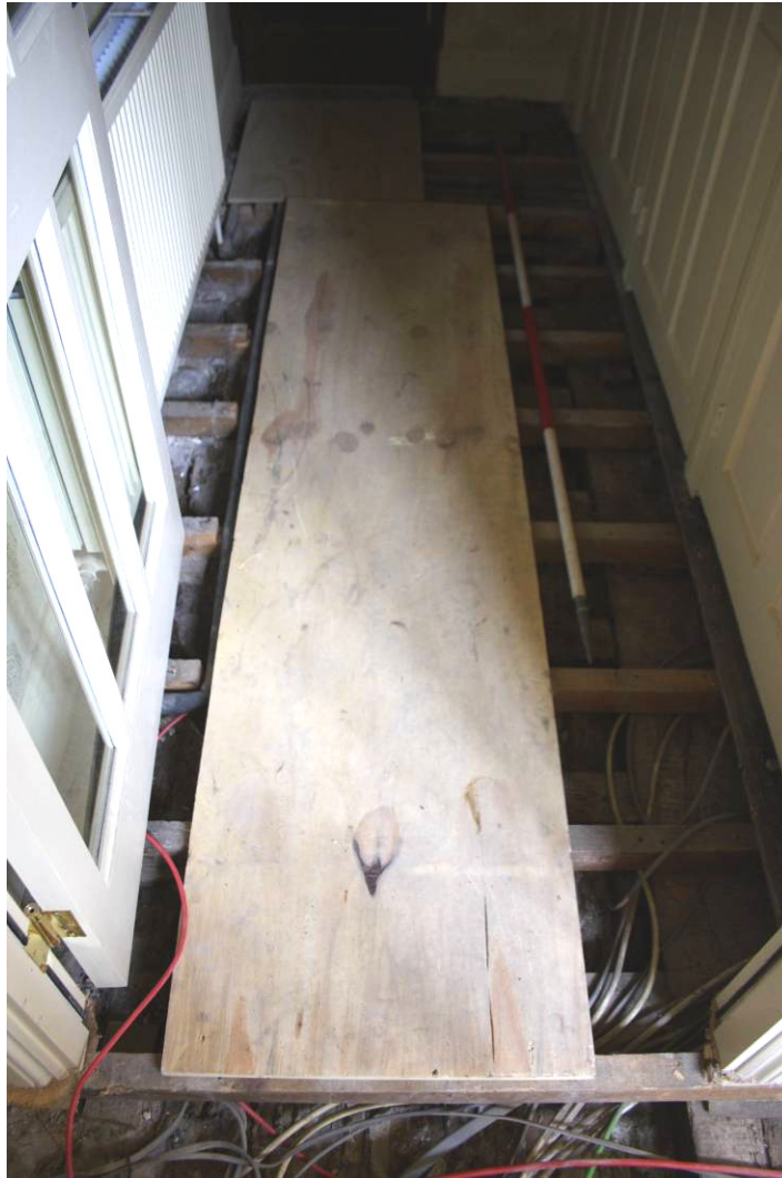
Photo 58: Corridor 113 (NE to SW section adjacent to cupboards showing beams visible running under the fixed walkway boards
