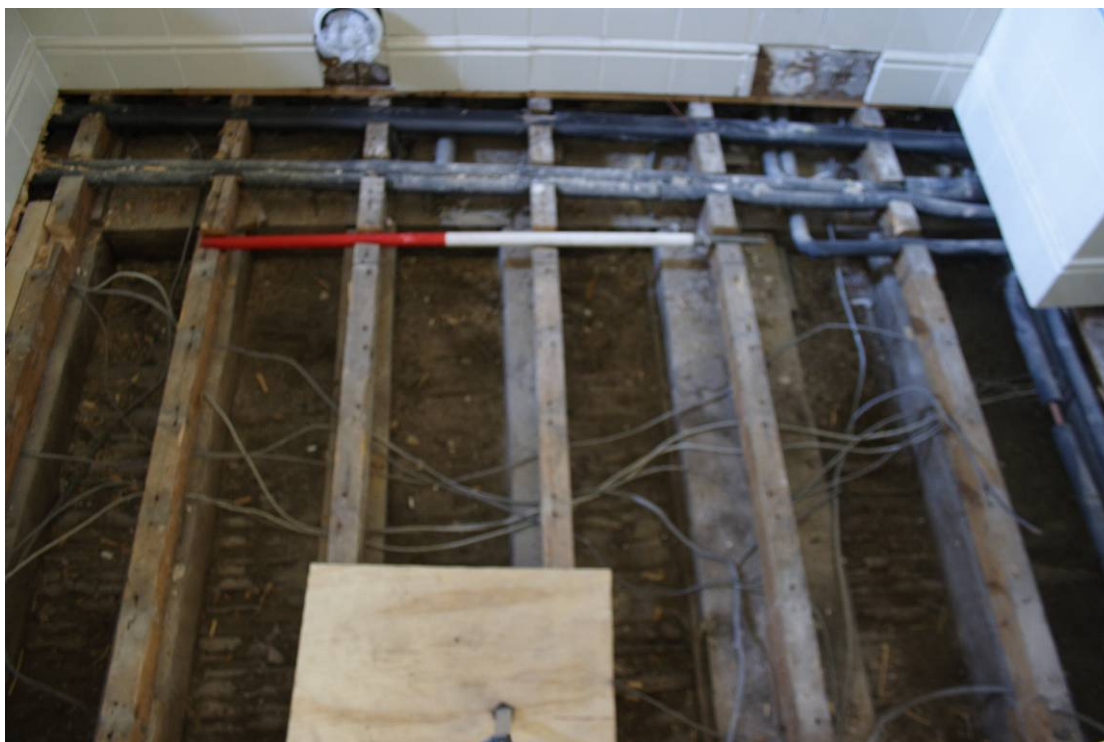
Photo 55: Bathroom 115 following removal of floorboards, viewing SE, showing underlying joists and large beams
