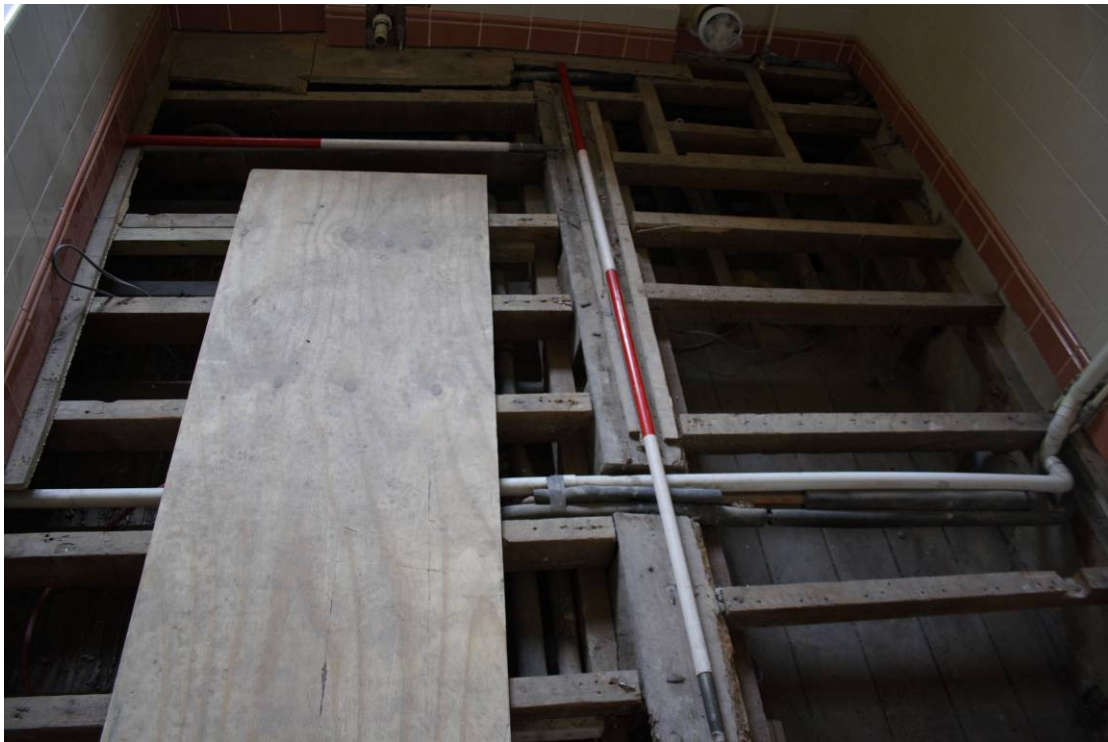
Photo 43: Bathroom 121 following removal of flooring showing joists, beam and lower area of floorboards
