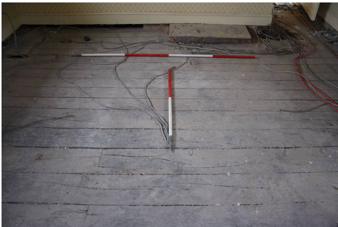
Photo 38: Northwestern end of Chapel Bedroom 122 showing earlier wide floorboards in bottom of photo with tongue and groove boards above, and brick plinth in front of presumed location of former fireplace
