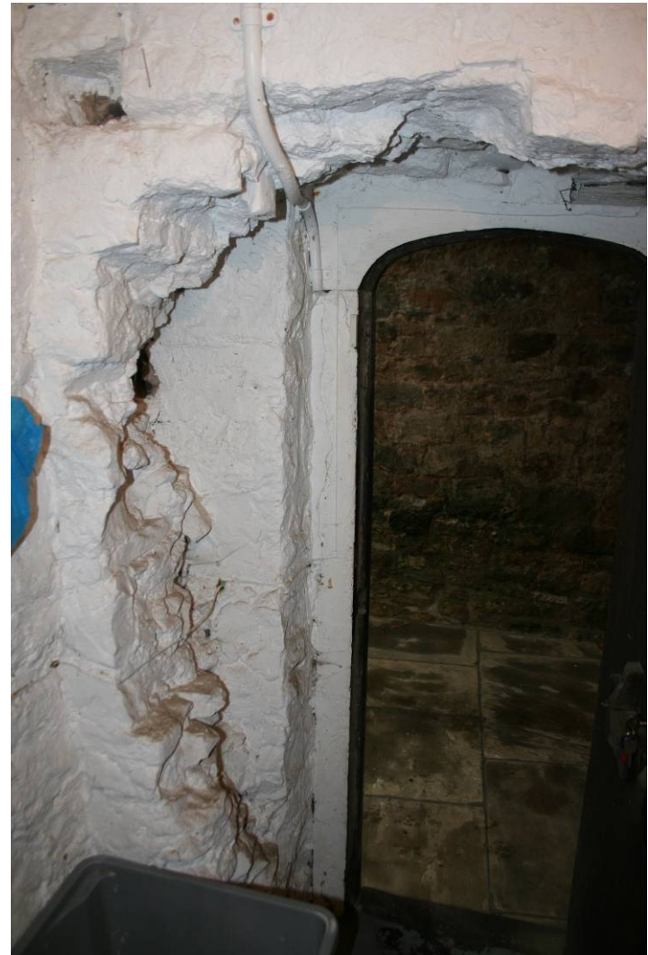
Photo 69: Inside of doorway accessing exterior passage from Room 035, showing breach in wall
