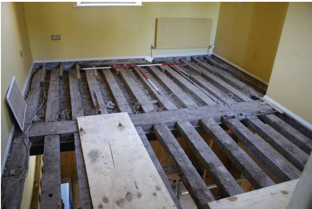
Photo 88: Floor of Bishop Morgan Bedroom 201 following removal of floorboards, with collapsed ceiling showing Bedroom 109 below
