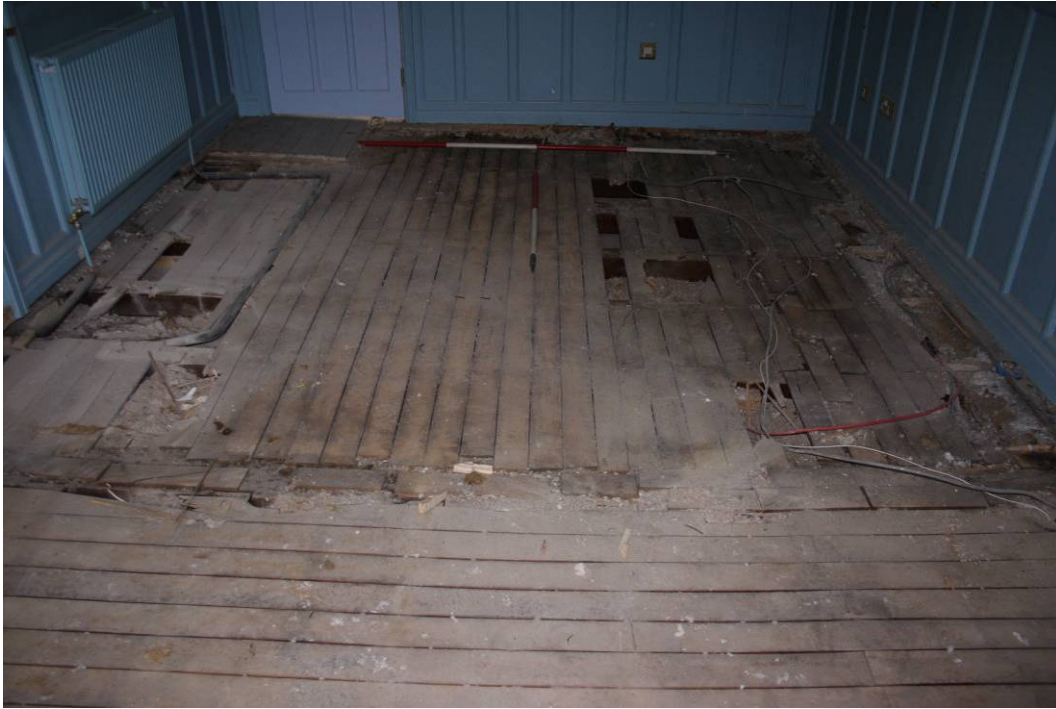
Photo 28: Room 105 viewing SW following removal of floorboards, showing change in floorboard direction and irregular slats over central beam
