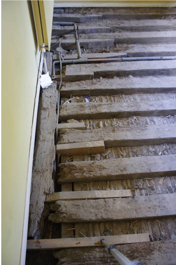
Photo 89: Wall plate along SW stone wall of Bishop Morgan Bedroom, showing decayed timbers and joists, and more recent repairs (as well as lath and plaster ceiling to Room 109 below)
