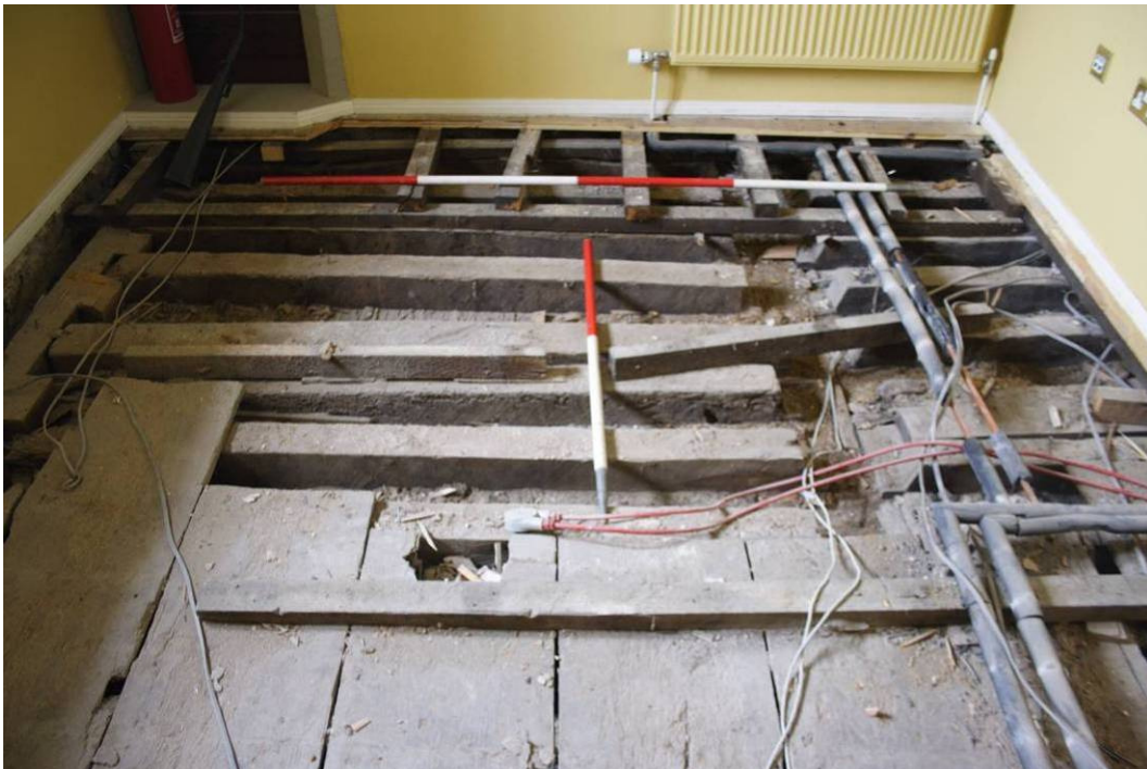
Photo 104: Bedroom 203 following removal of modern floorboards and exposure of underlying elm boards and beams and joists in NW half of room
