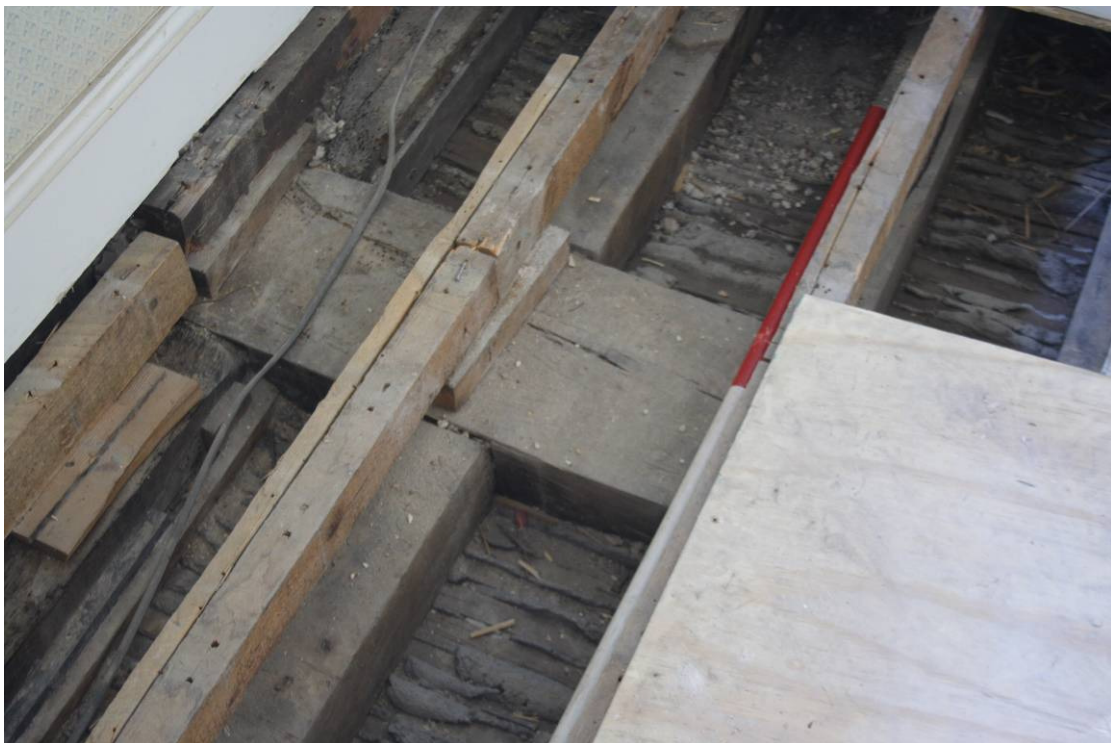
Photo 54: Bishop Miles Salley Bedroom 114 following the removal of floorboards, viewing eastern corner of room with main cross beam and wall beam
