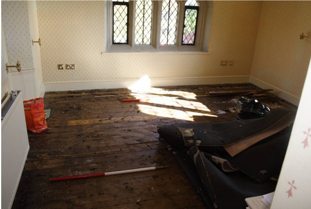
Photo 36: Chapel Bedroom 122 prior to removal of floorboards, viewing east from doorway to Room 121
