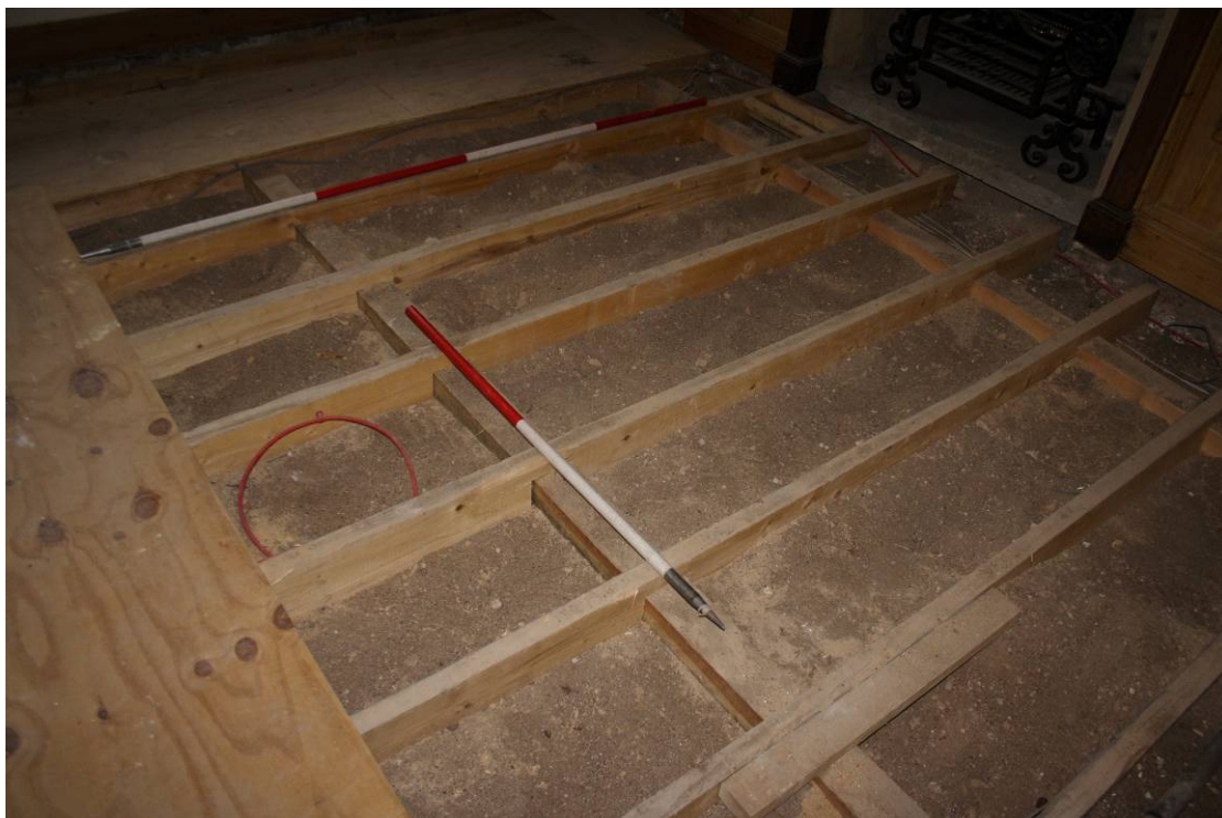
Photo 74: Bishop de La Zouche Lounge 111, following removal of ply-board sheeting, showing modern timber frame beneath sitting on sand
