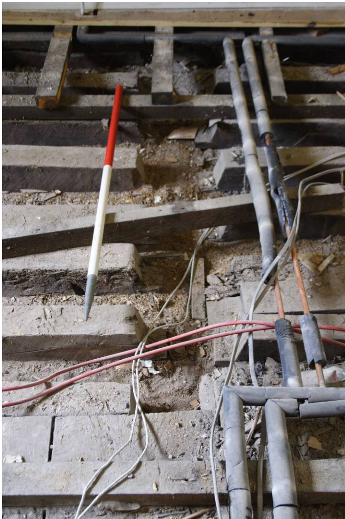
Photo 105: Decayed beam across floor of Bedroom 203 showing joists resting on top of the surviving part
