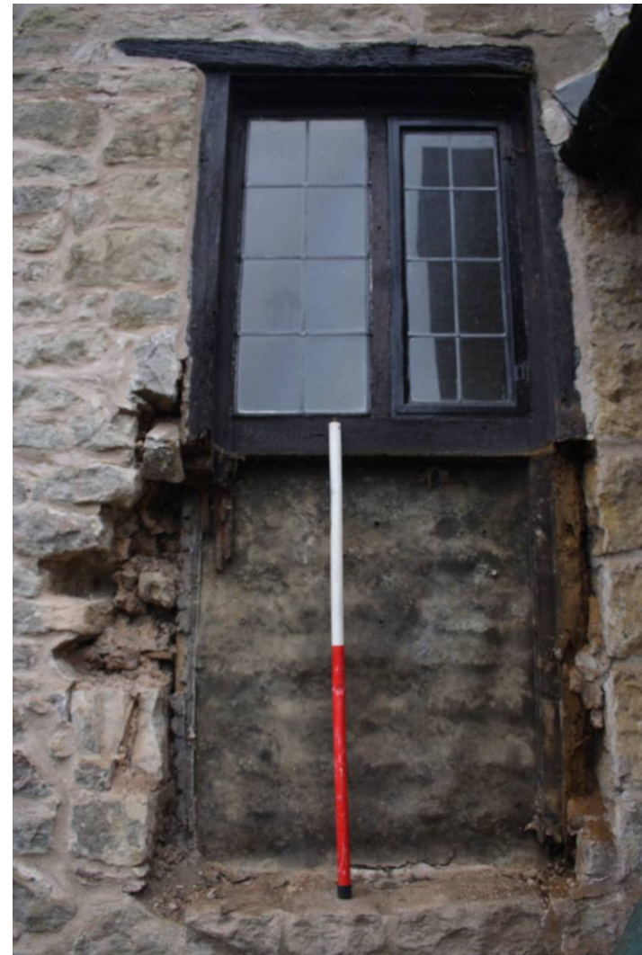
Photo 13: Detail of doorway during reopening, showing exposed remains of former timber doorframe and tar paper
