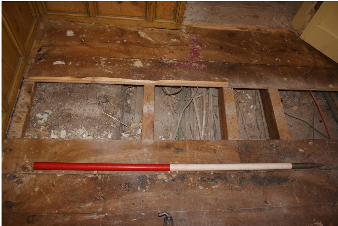
Photo 82: Bedroom 109, small opening through floorboards showing stone wall and modern joists resting on earlier joists
