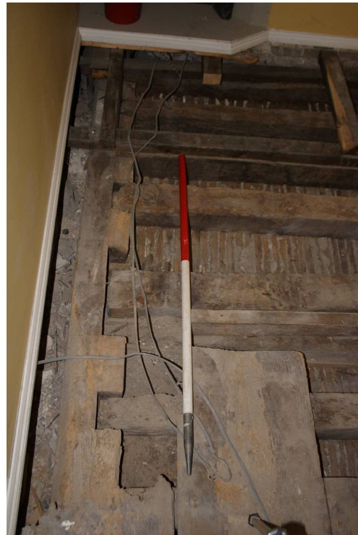
Photo 106: Wall plate beam on SW wall of room showing notches for joists
