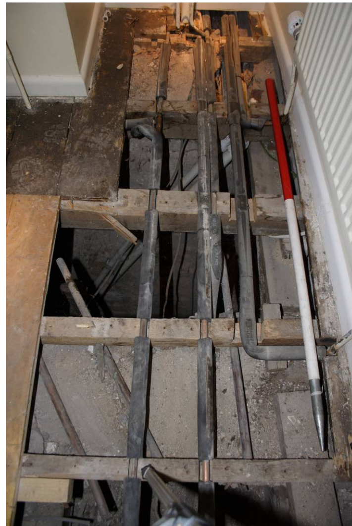
Photo 96: Bathroom 202 following removal of most of the modern floorboards showing underlying stonewalls and probable garderobe chute
