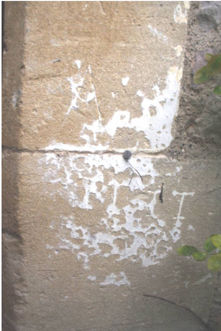
Photo 17: Graffiti on right hand side of doorway
