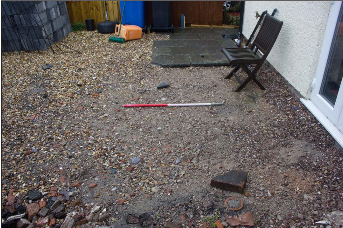
Plate 01: Pre excavation shot of site area to rear of Longton, Parliament Street, Rhuddlan, Denbighshire - from the southeast - 1.00m scale
