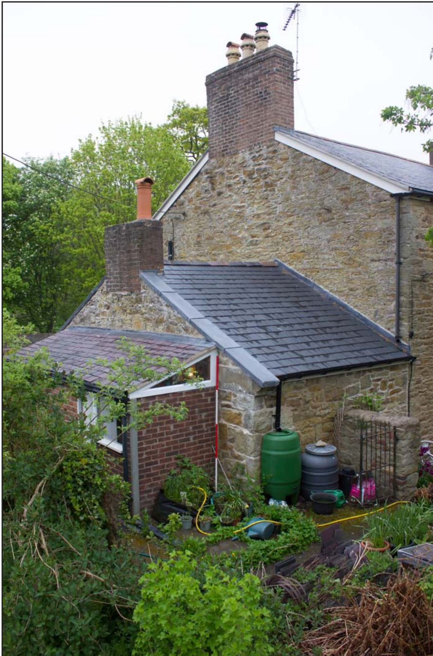
Plate 08: Oblique shot of northwest elevation of Ty Carreg, Northop, Mold, Flintshire - from the southwest - 2.00m scale
