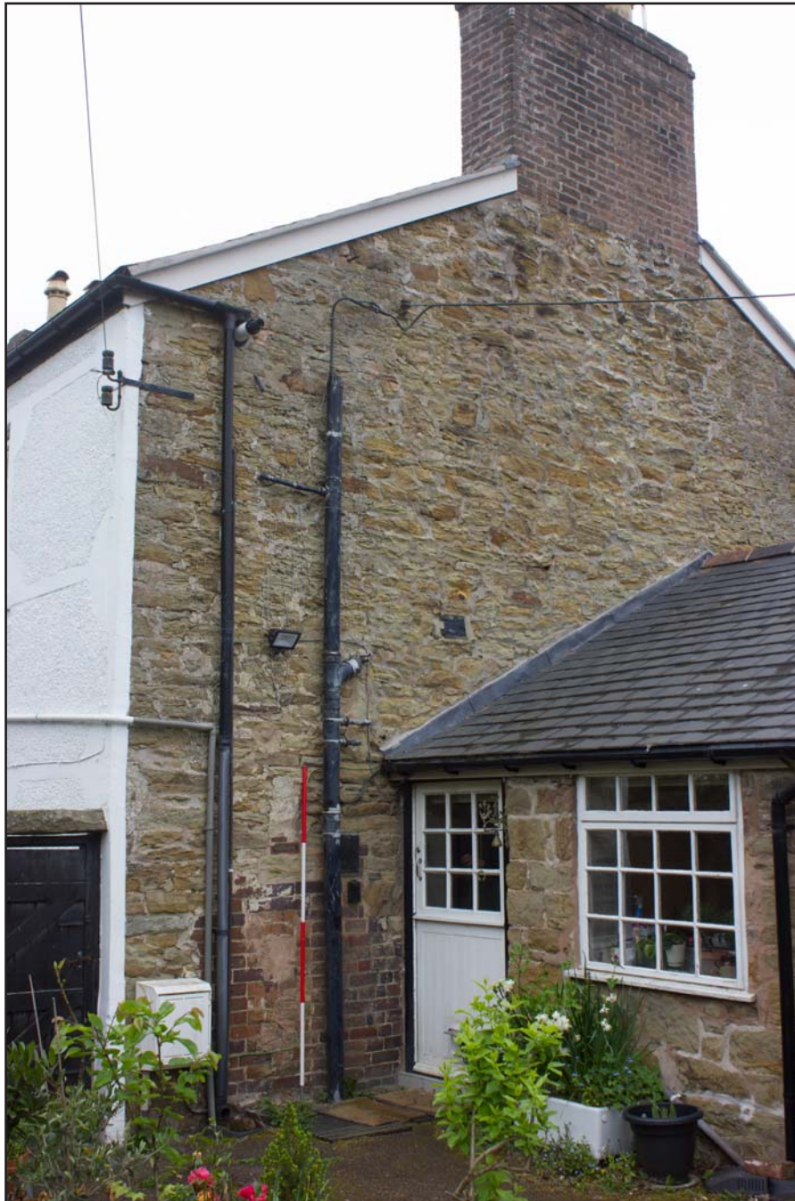
Plate 11: Focus shot on northwest gable elevation of Ty Carreg, Northop, Mold, Flintshire - from the northwest - 2.00m scale
