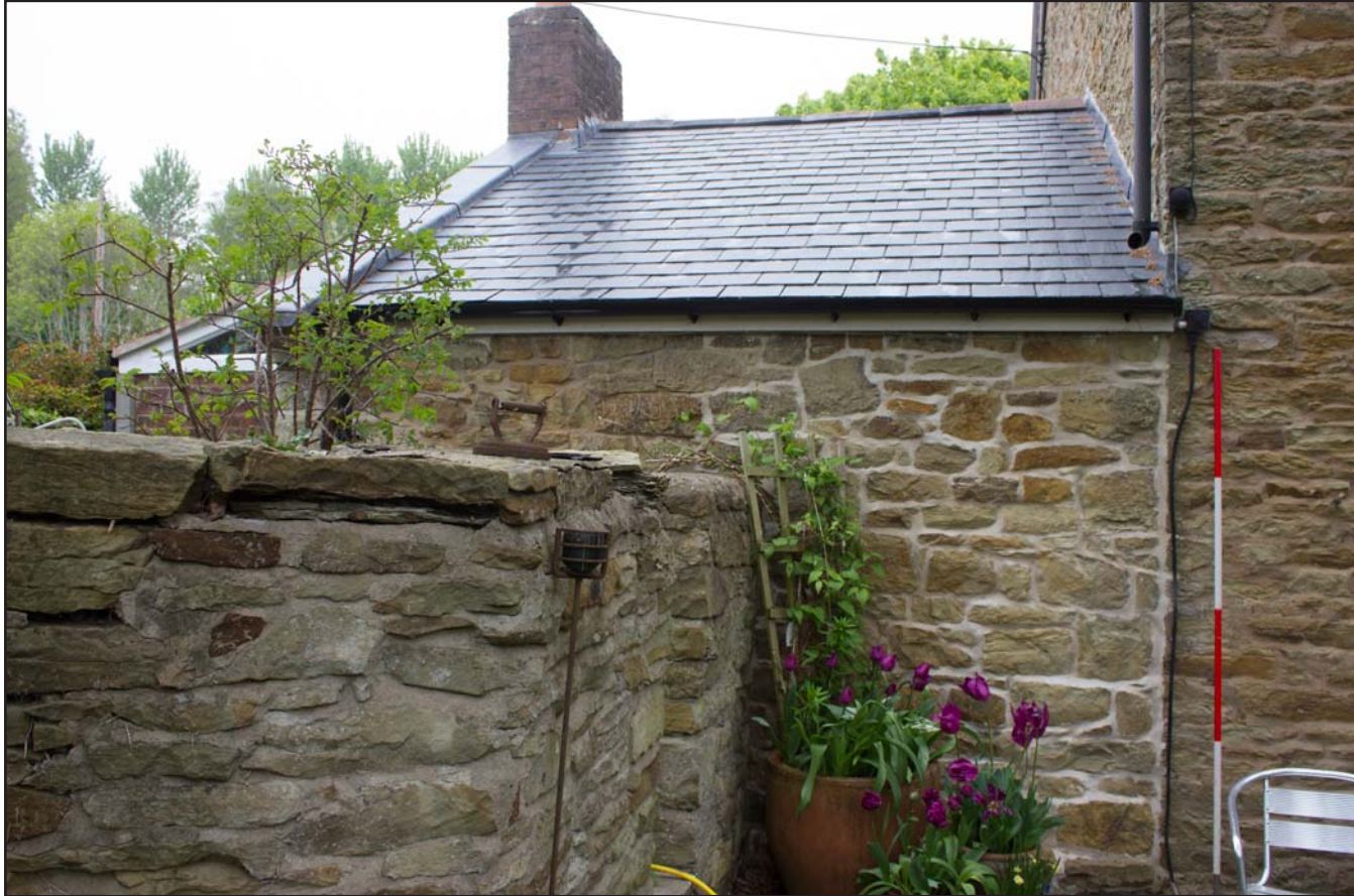
Plate 06: Southwest elevation (left) shot of Ty Carreg, Northop, Mold, Flintshire - from the southwest - 2.00m scale
