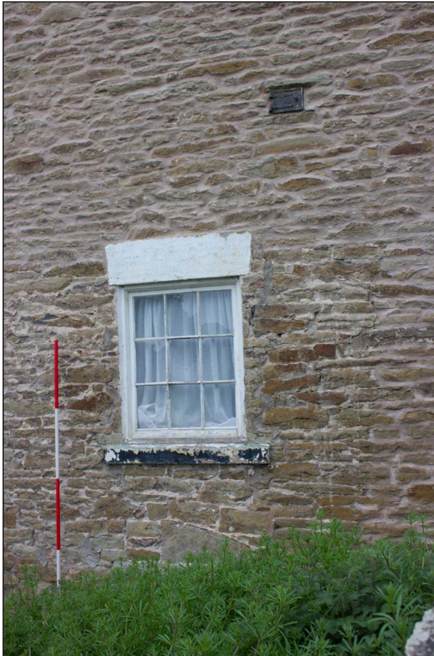
Plate 04: Window and fire hatch on southeast elevation shot of Ty Carreg, Northop, Mold, Flintshire - from the southeast - 2.00m scale
