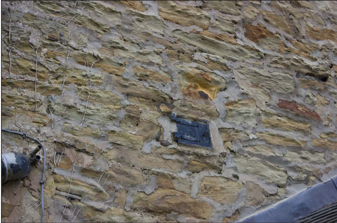
Plate 12: Cast Iron fire hatch on northwest gable elevation of Ty Carreg, Northop, Mold, Flintshire - from the northwest - no scale
