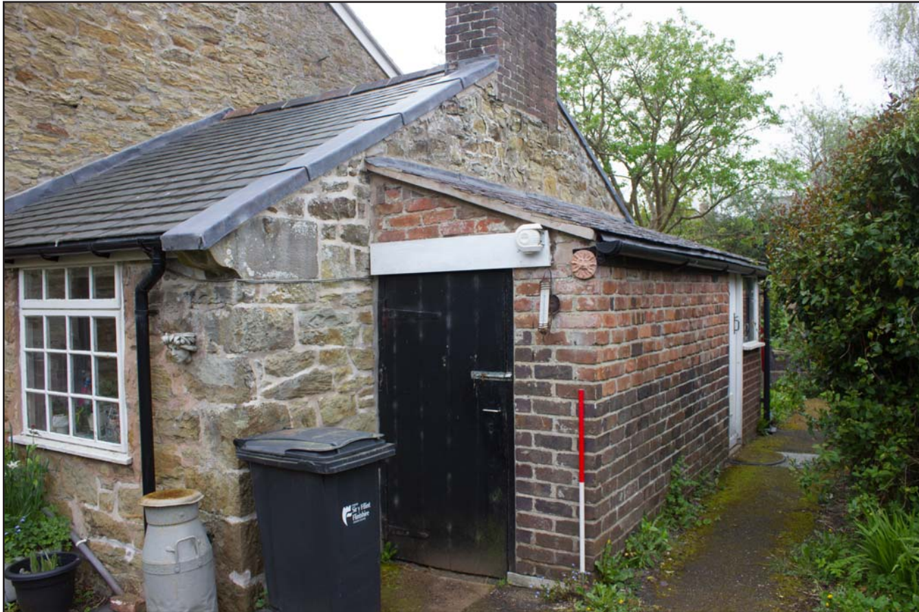
Plate 19: External shot of brick out building at Ty Carreg, Northop, Mold, Flintshire - from the northwest - 1.00m scale
