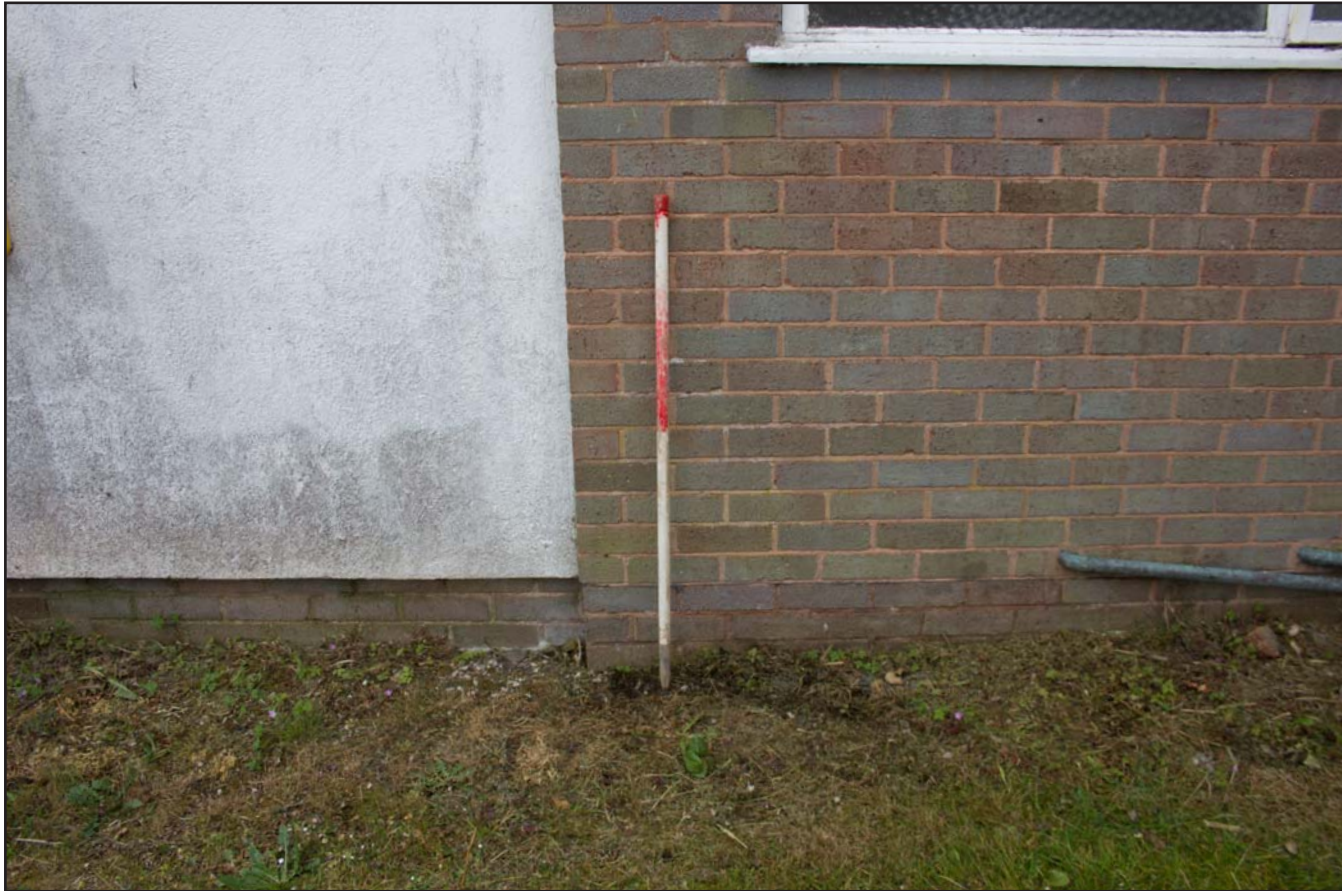
Plate 06: Pre excavation shot of foundation reveal pit (C) at Llanefydd Village Hall, Godre'r Graig, Llanefydd - from the northeast - scale 1m
