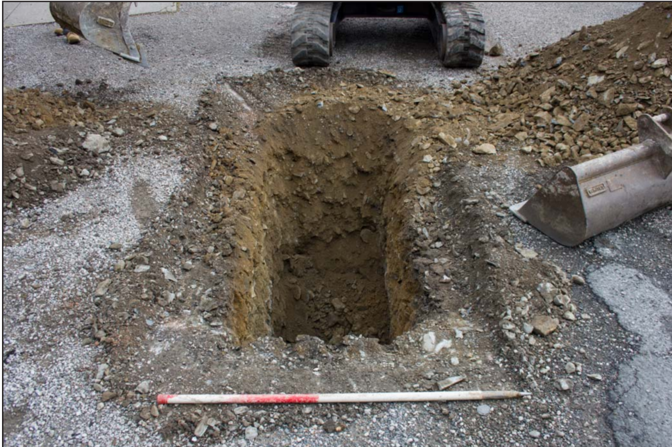
Plate 03: Post excavation plan shot of Percolation Pit (A) at Llanefydd Village Hall, Godre'r Graig, Llanefydd - from the southeast - scale 1m
