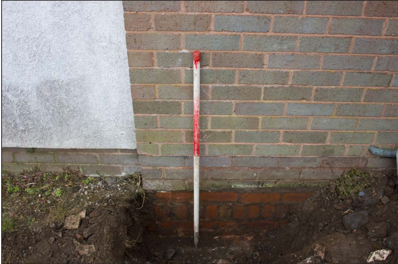
Plate 07: Post excavation shot of foundation reveal pit (C) at Llanefydd Village Hall, Godre'r Graig, Llanefydd - from the northwest - scale 1m
