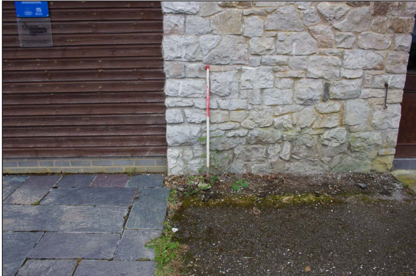
Plate 04: Pre excavation shot of foundation reveal pit (B) at Llanefydd Village Hall, Godre'r Graig, Llanefydd - from the northeast - scale 1m
