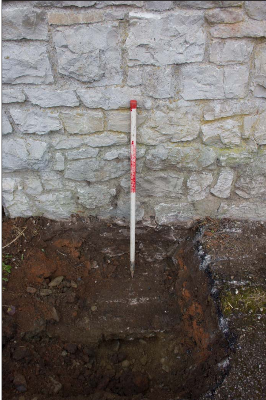
Plate 05: Post excavation shot of foundation reveal pit (B) at Llanefydd Village Hall, Godre'r Graig, Llanefydd - from the northwest - scale 1m
