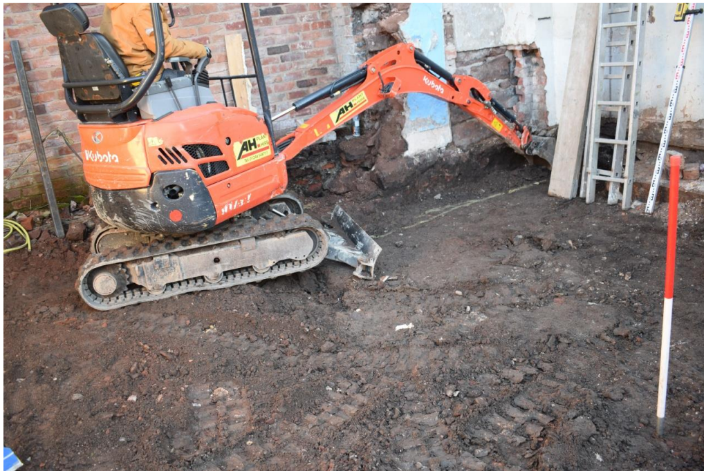
Figure 5 Initial excavation beginning at the north part of the site. Viewed from south west. CPAT photo 4961-0002
