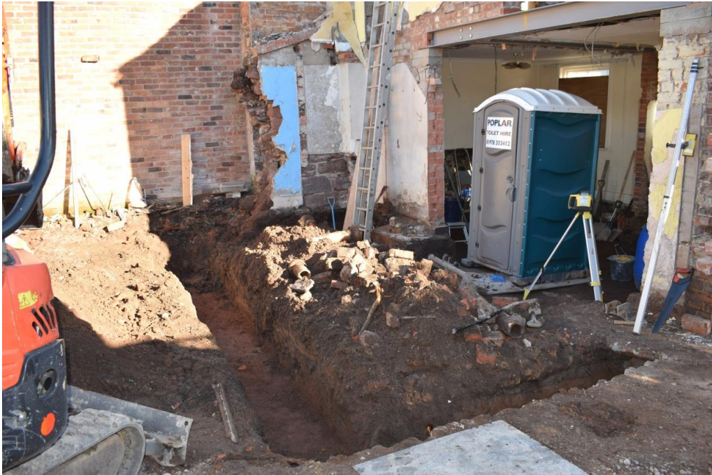
Figure 8 The excavated trench as it appeared at the conclusion of the first stage. Viewed from the south-west. CPAT photo 4961-0015
