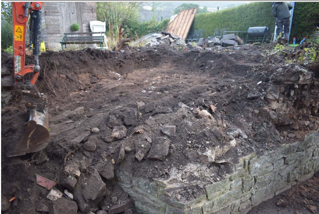
Fig. 6 Stripped topsoil showing concreted material behind revetment and imported soil. CPAT photo 4945-0007
