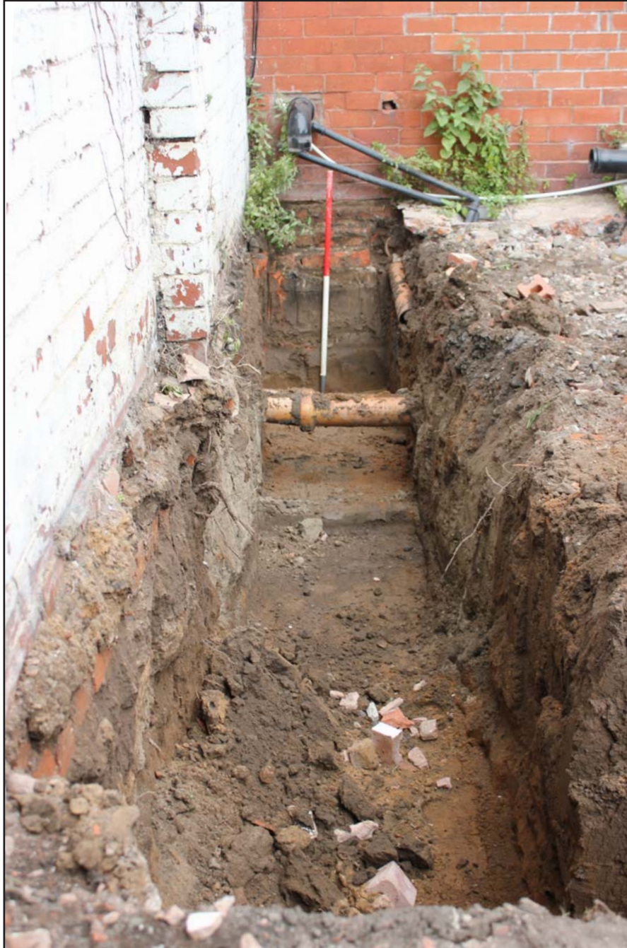
Plate 02: Trench A (showing section collapse) at Plas Llewelyn, Hylas Lane, Rhuddlan, Denbighshire - from the south - scale 1m
