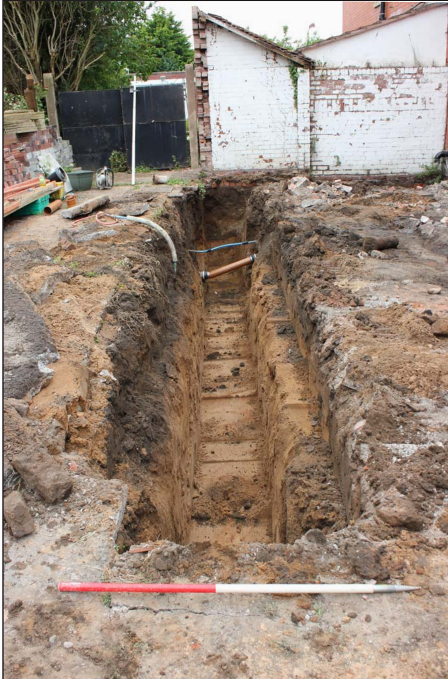
Plate 03: Trench B at Plas Llewelyn, Hylas Lane, Rhuddlan, Denbighshire - from the east - scale 1m
