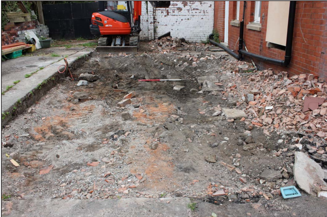
Plate 01: Pre excavation shot of extension area at Plas Llewelyn, Hylas Lane, Rhuddlan, Denbighshire - from the east - scale 1m
