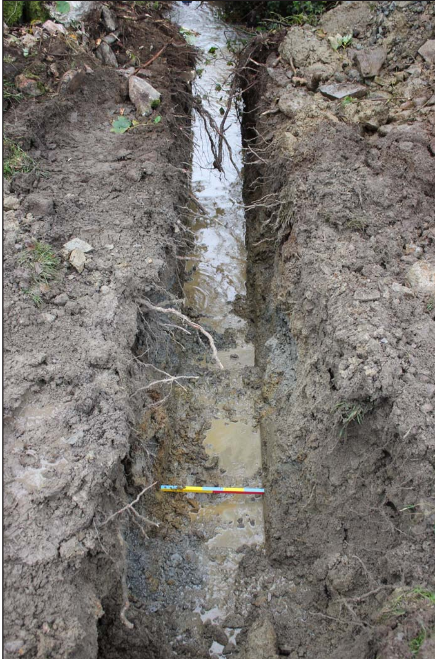
Plate 81: Pipe trench within Field L north of Nânt y lâr - from the south - scale 0.5m
