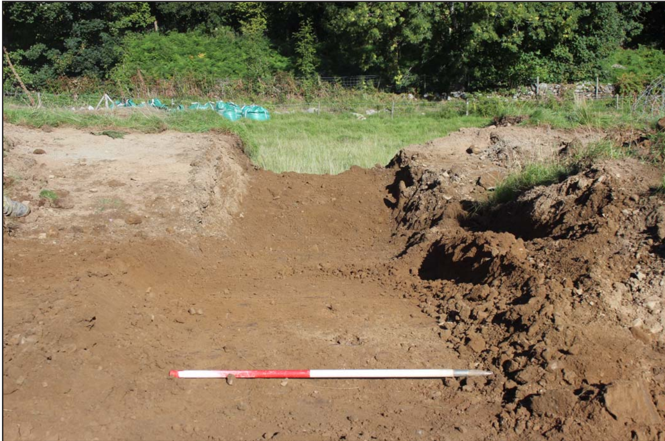
Plate 12: Pipe trench in Field C/D boundary looking downslope to Valley Road - from the south- scale 1m
