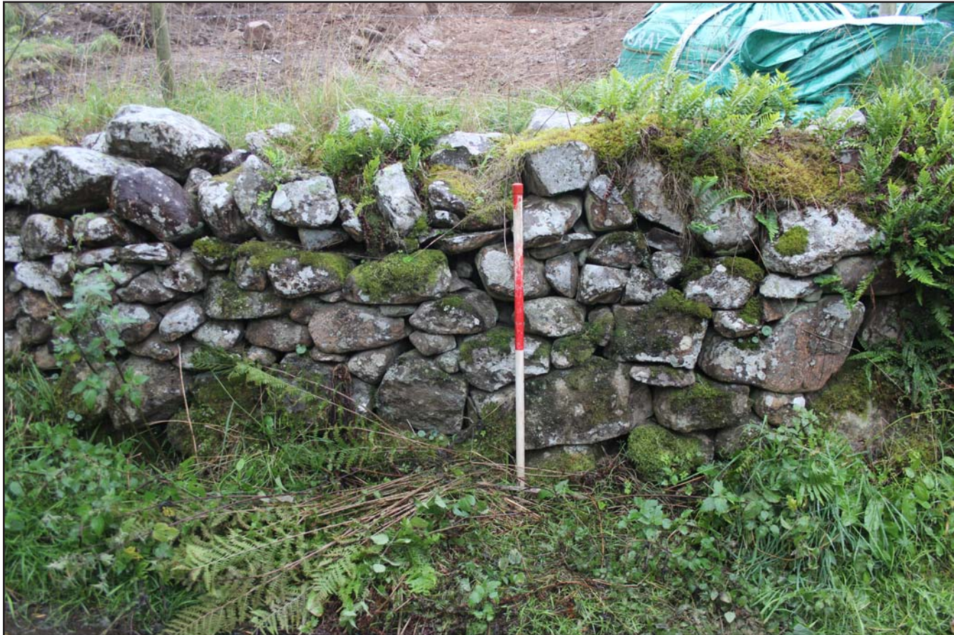
Plate 16: Pre breach of field wall south of Valley Road (Field D) - from the north - scale 0.05m
