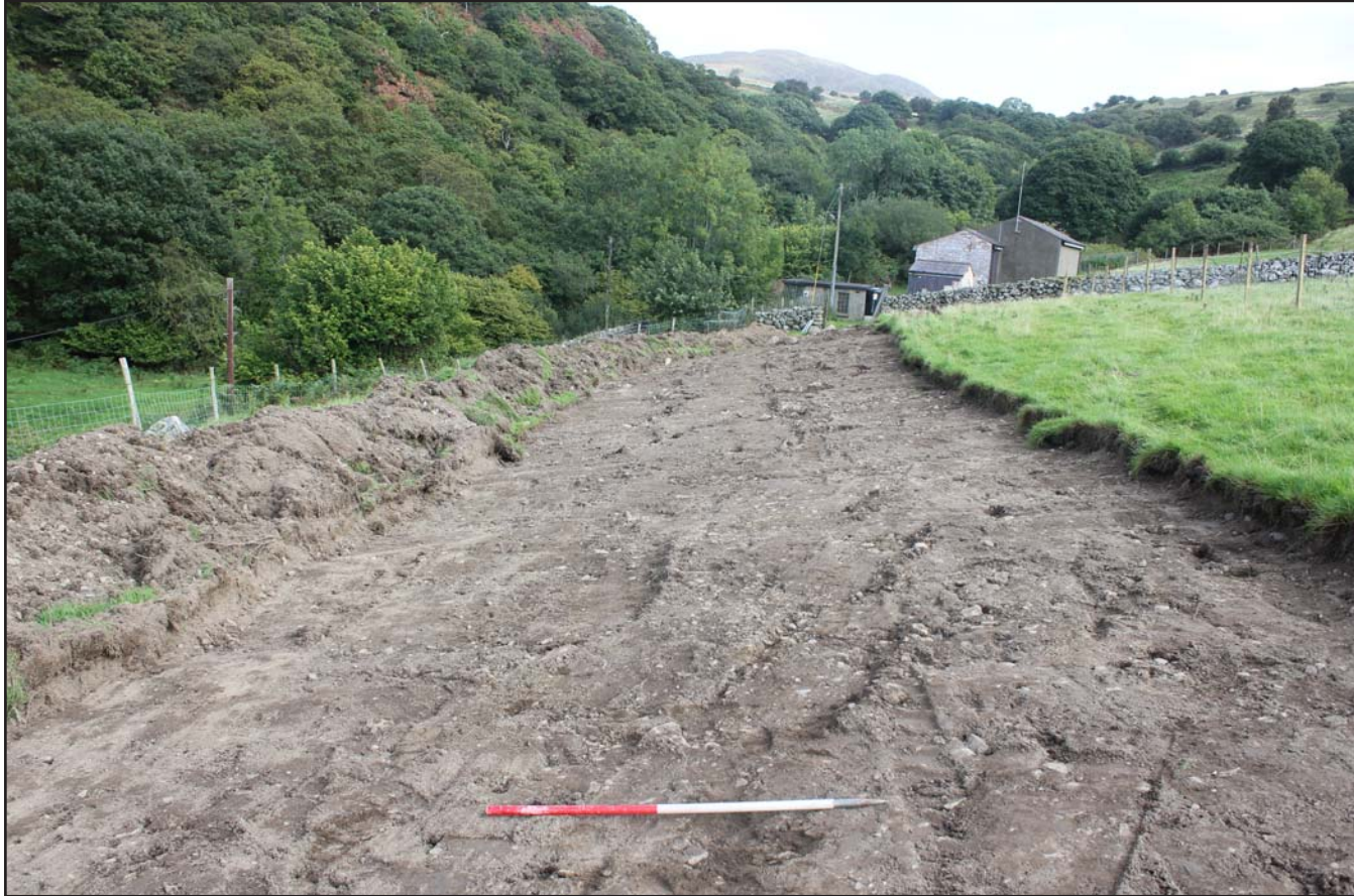
Plate 03: Topsoil Strip shot looking southeast towards pumping station - from the northeast - scale 1m
