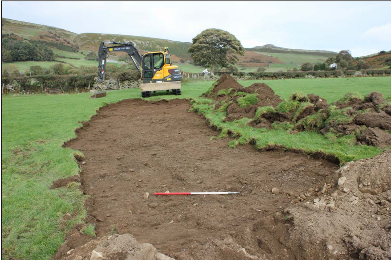
Plate 61: Topsoil strip within Field H to 1st launch pit - from the south - scale 1m
