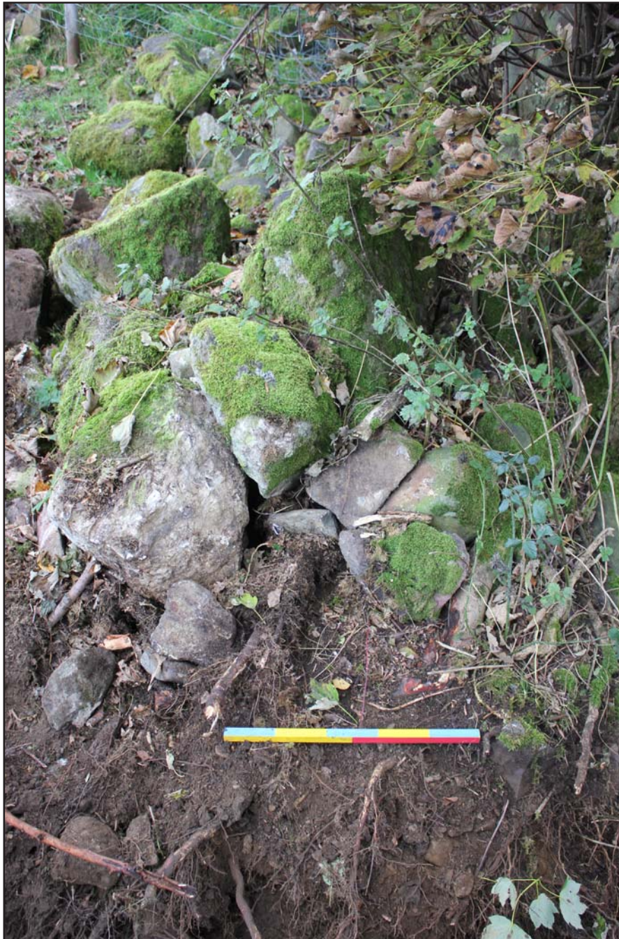
Plate 80: Section of breached wall south of Nânt y lâr within Field L - from the south - scale 0.5m
