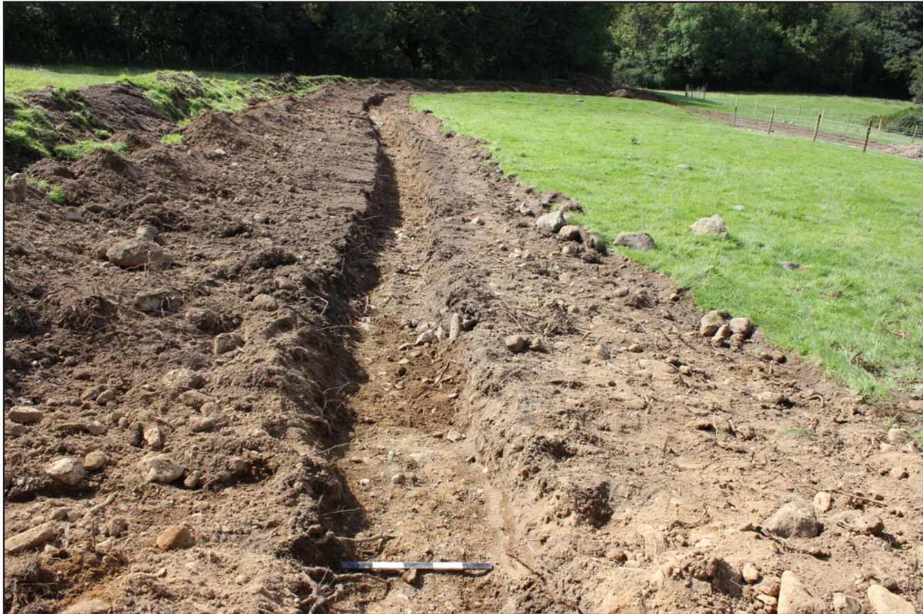
Plate 55: Pipe trench base of Field F (top of field) - Route 2 - from the north - scale 0.5m
