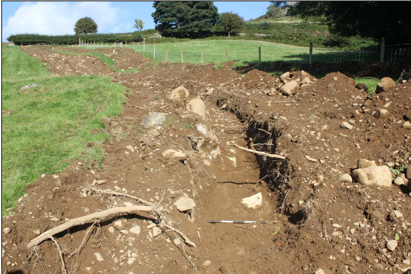
Plate 31: Pipe trench within Field F (from the base of slope) - Route 1 - from the southwest - scale 0.5m
