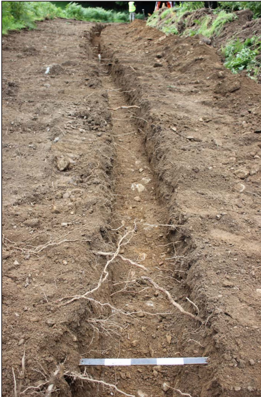
Plate 20: Pipe trench within Field E looking west - from the east - scale 0.5m
