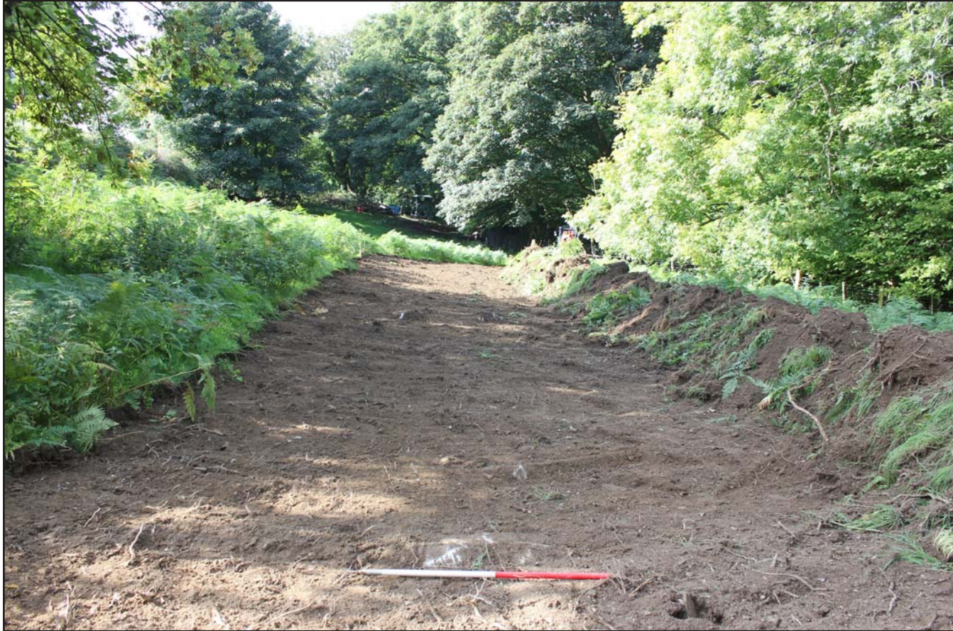
Plate 18: Topsoil Strip in Field E looking west- from the east - scale 1m
