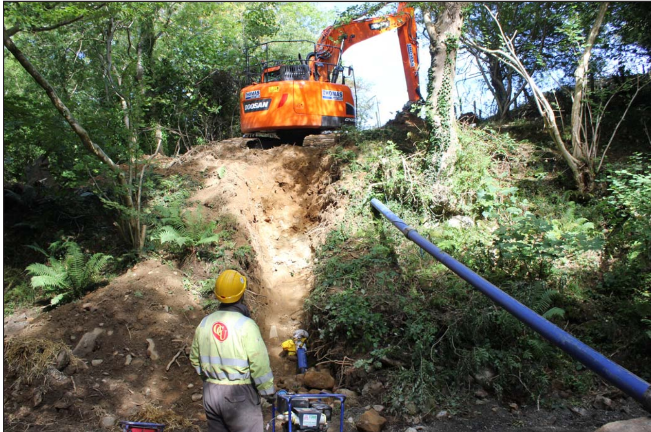
Plate 26: Pipe trench in northern bank of Afon Llanfairfechan - from the south - scale n/a
