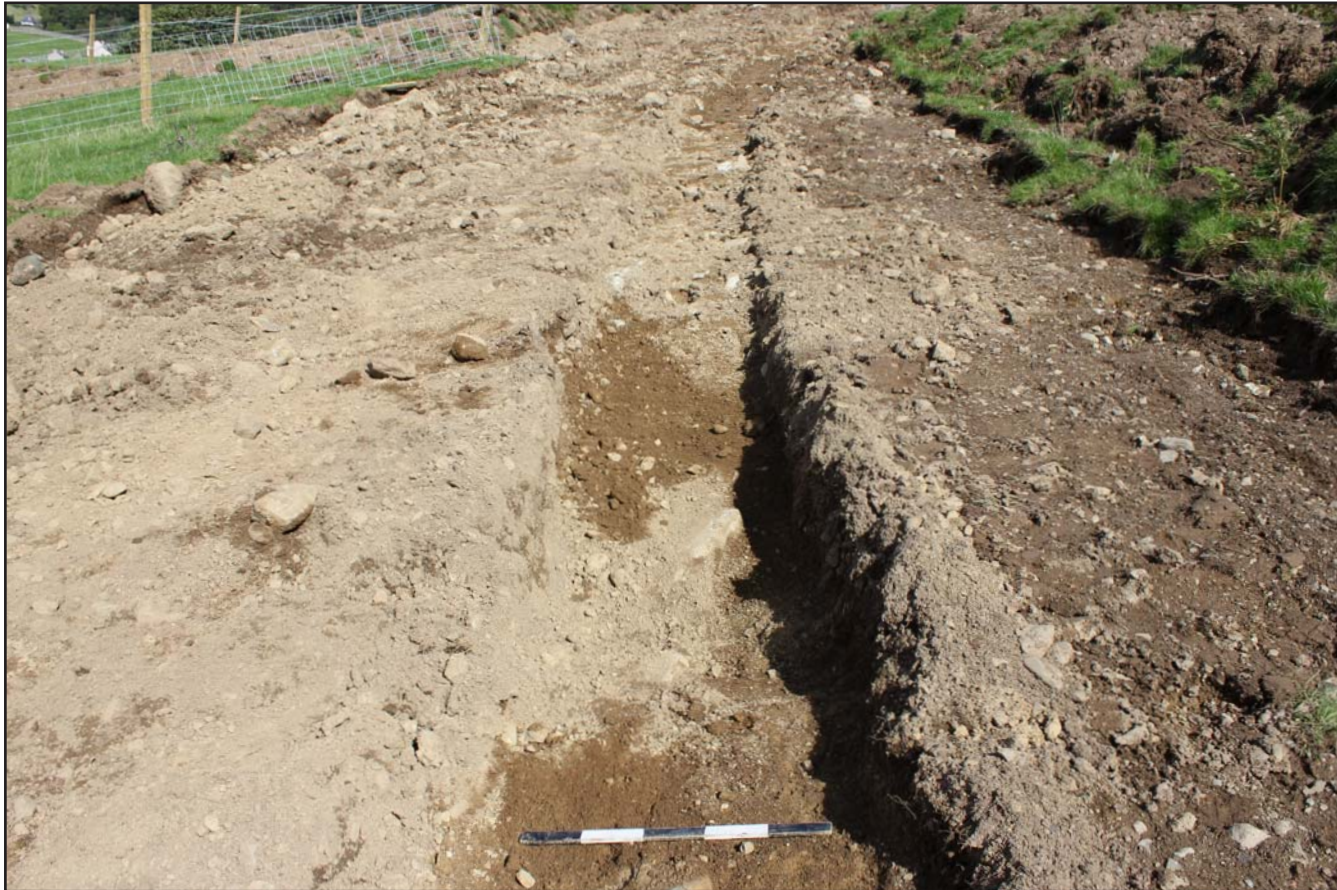
Plate 56: Pipe trench base of Field G (base of field) - Route 2 - from the north - scale 0.5m
