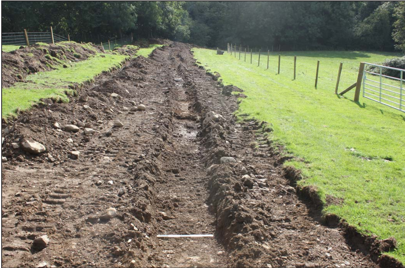
Plate 32: Pipe trench within Field F (looking downslope) - Route 1 - from the northeast - scale 0.5m
