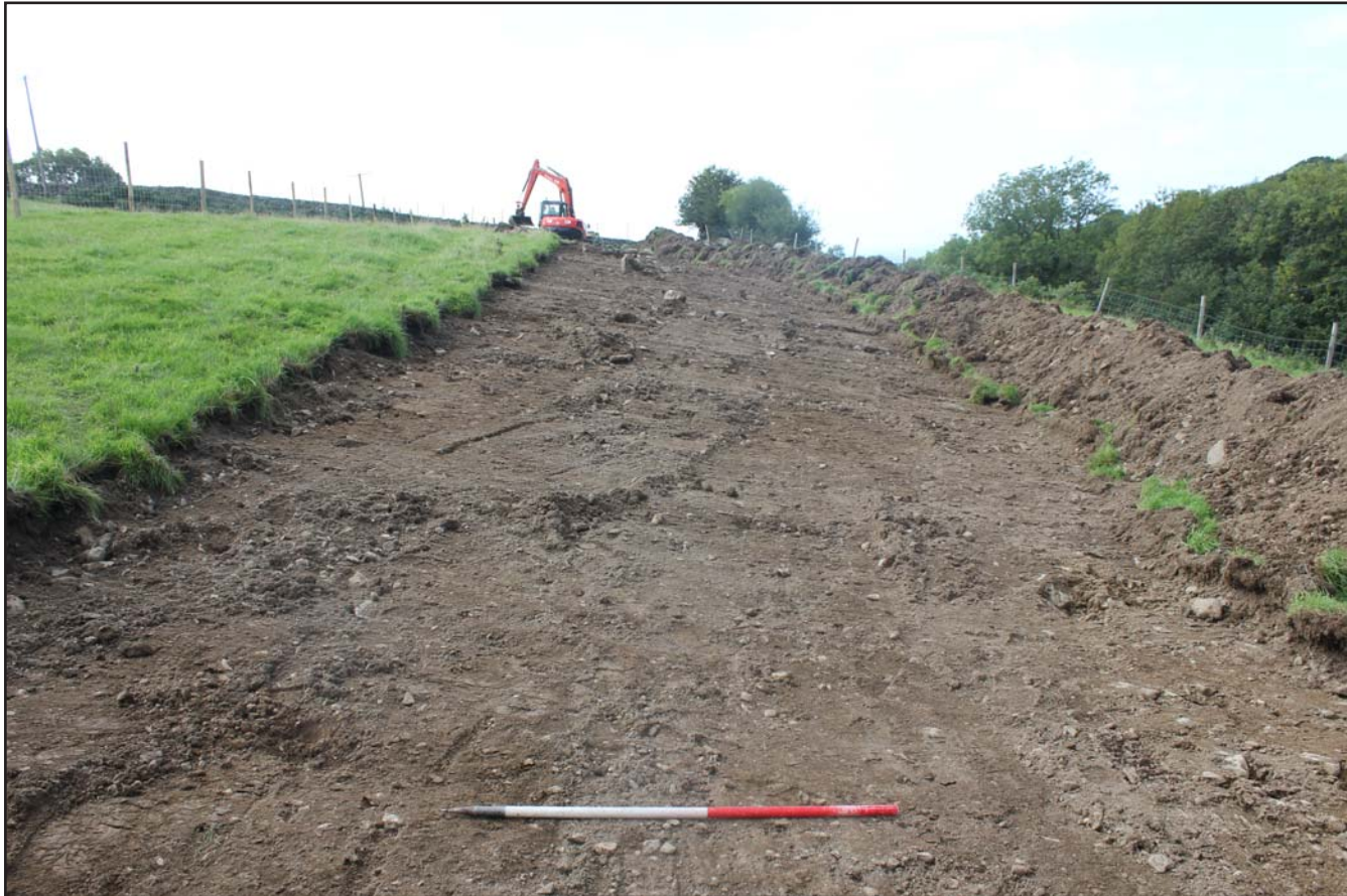
Plate 02: Topsoil Strip shot looking northwest away from pumping station - from the southwest - scale 1m
