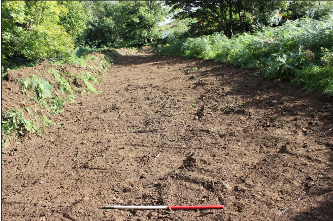
Plate 19: Topsoil Strip in Field E looking east- from the west - scale 1m
