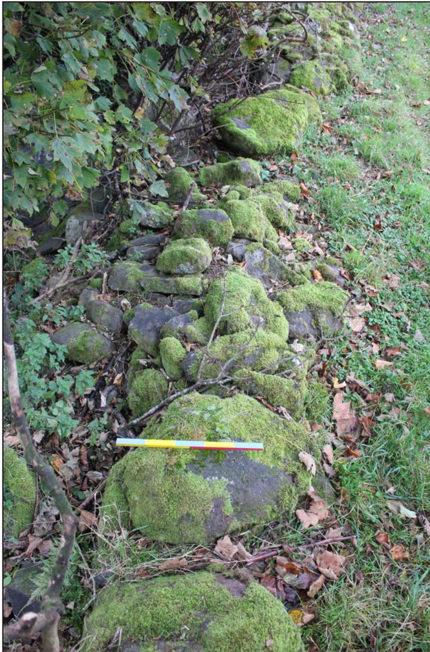
Plate 79: Wall south of Nânt y Iâr within Field L - from the southwest - scale 0.5m
