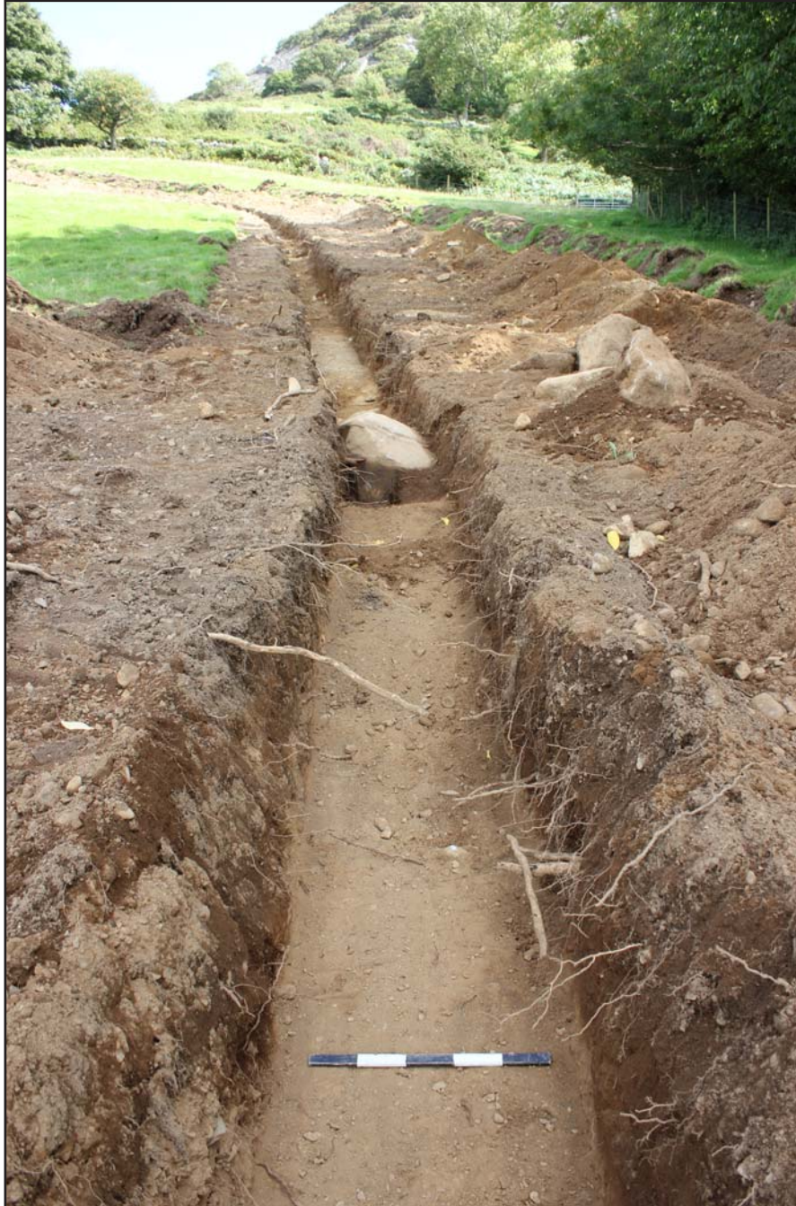
Plate 54: Pipe trench base of Field F (base of field) - Route 2 - from the southwest - scale 0.5m
