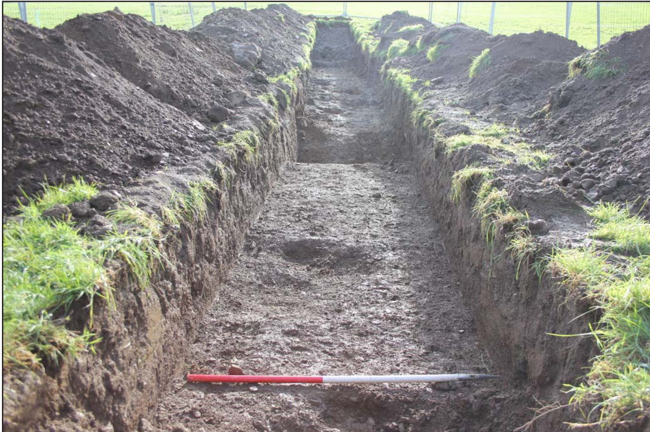
Plate 59: Test pit within Field H to locate water main - from the southwest - scale 1m
