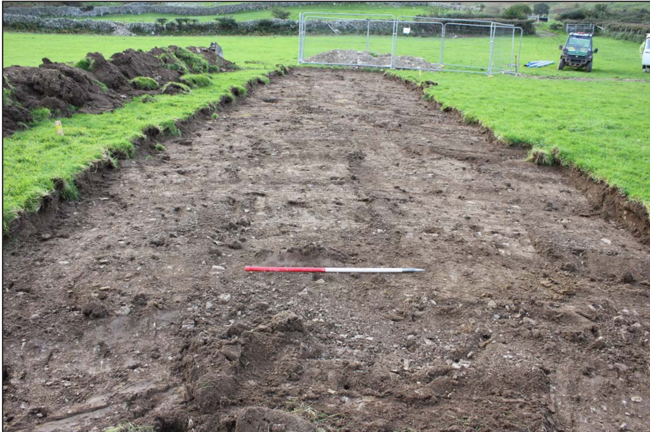
Plate 60: Topsoil strip in Field H to 1st launch pit - from the northeast - scale 1m
