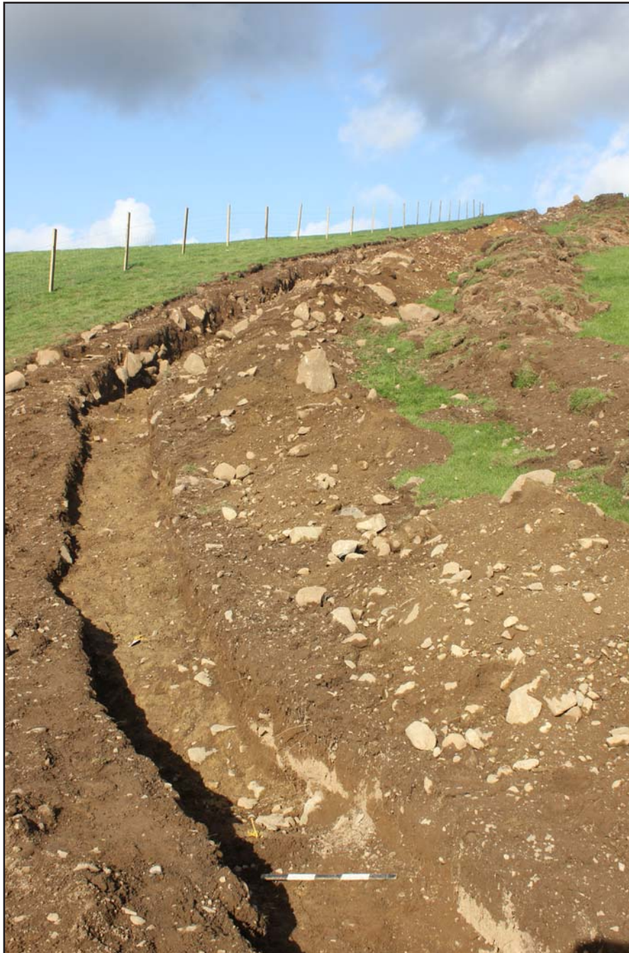
Plate 33: Pipe trench within Field G (looking upslope) - Route 1 - from the south - scale 0.5m
