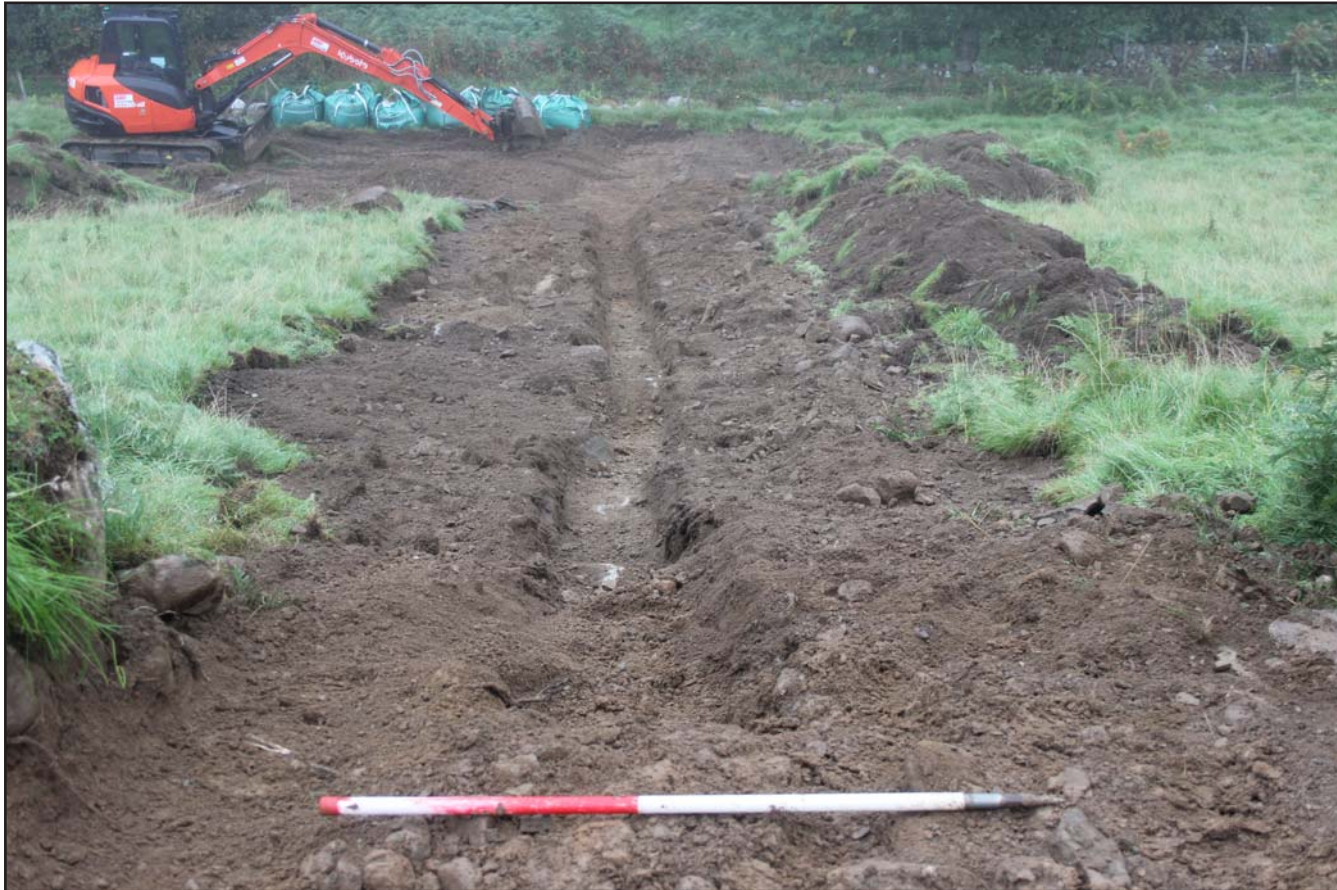
Plate 15: Pipe trench within Field D looking downslope - from the south - scale 0.5m
