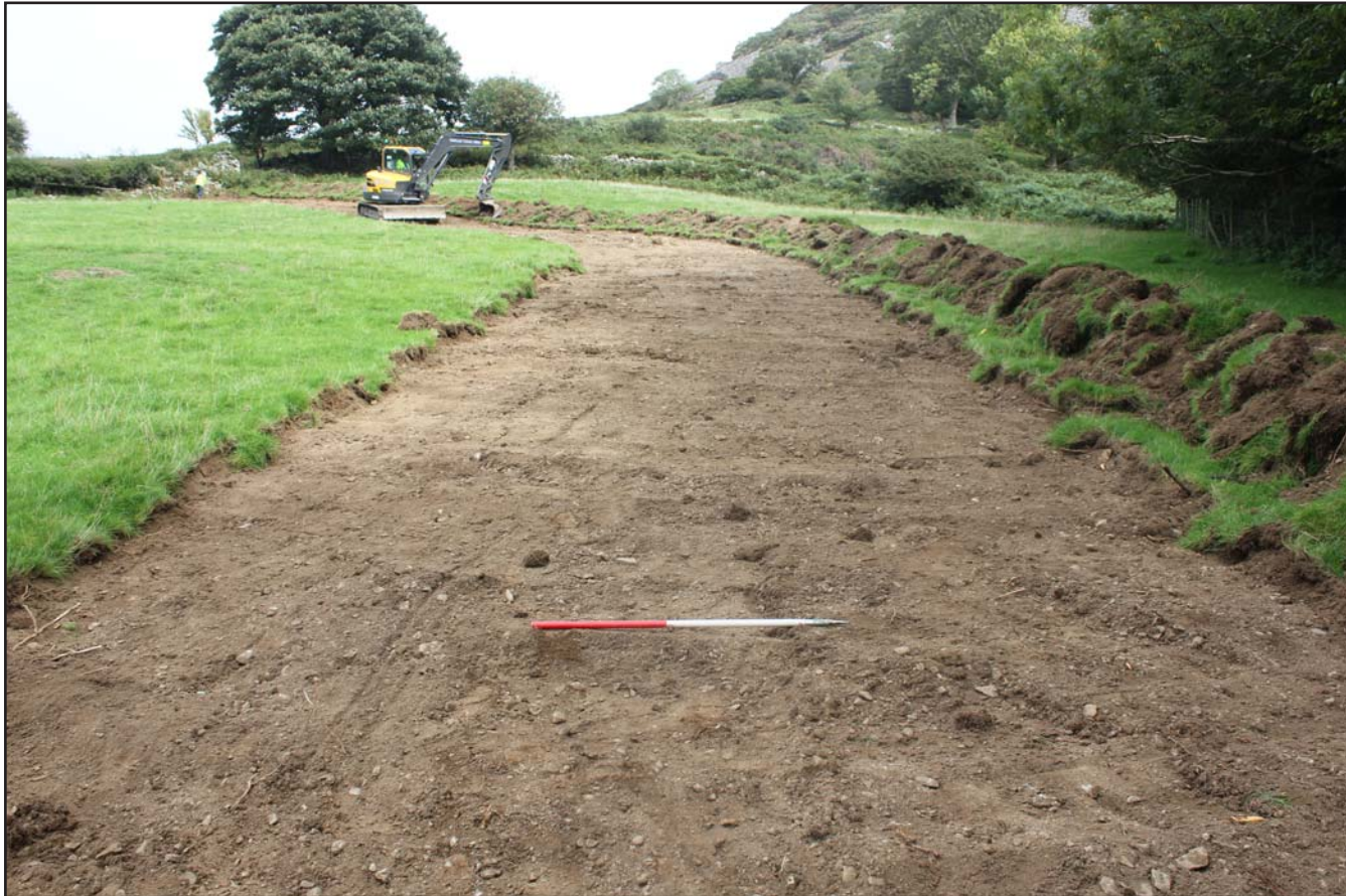
Plate 48: Topsoil strip within Field F (from the base of the slope) - Route 2 - from the southwest - scale 1m
