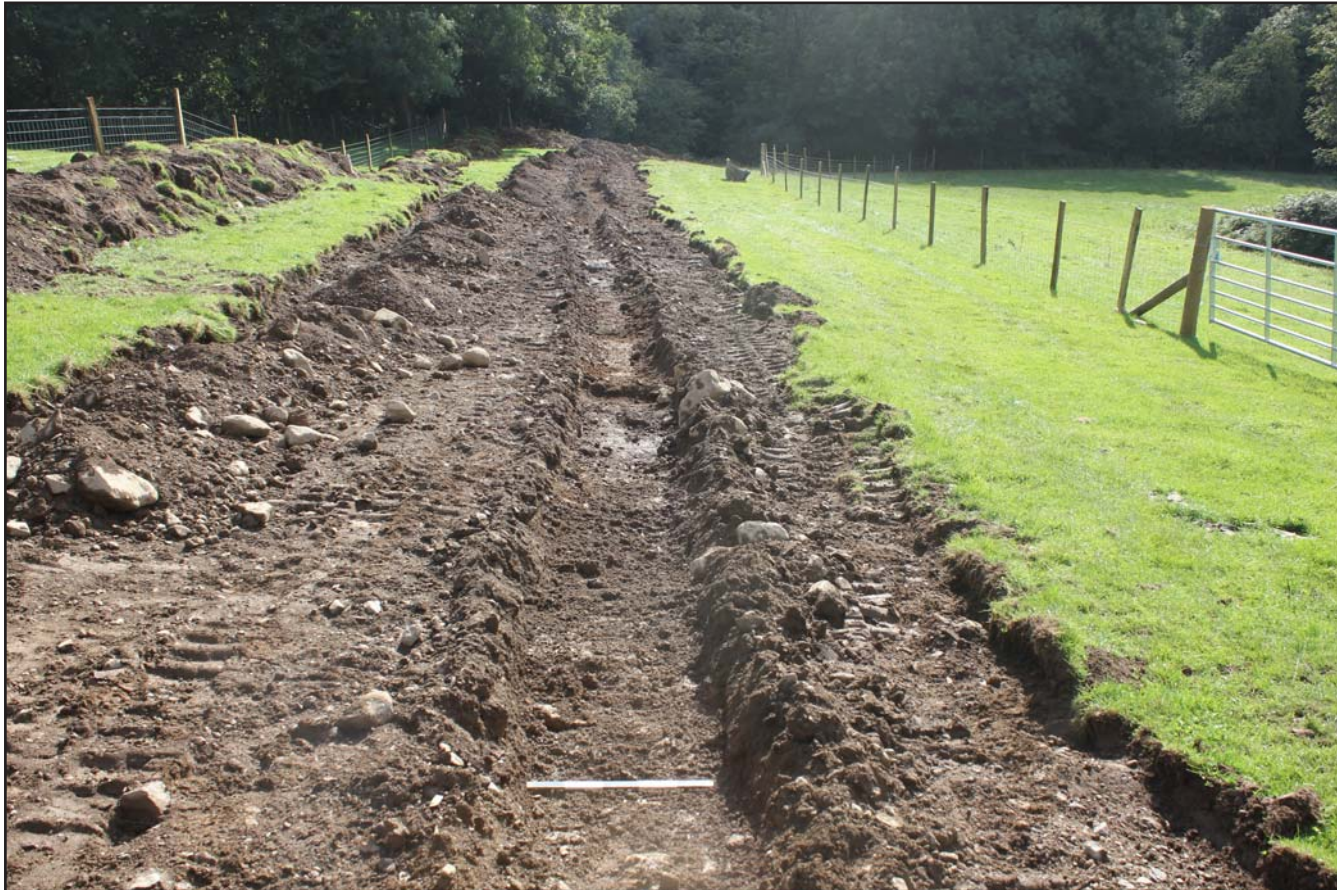
Plate 34: Pipe trench within Field G (top of slope) - Route 1 - from the north - scale 0.5m
