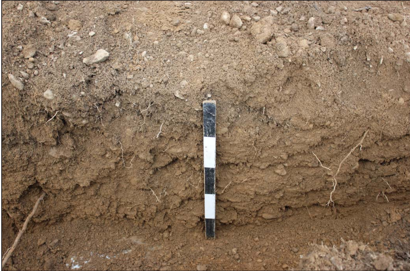
Plate 22: Section of pipe trench within Field E - from the north - scale 0.5m
