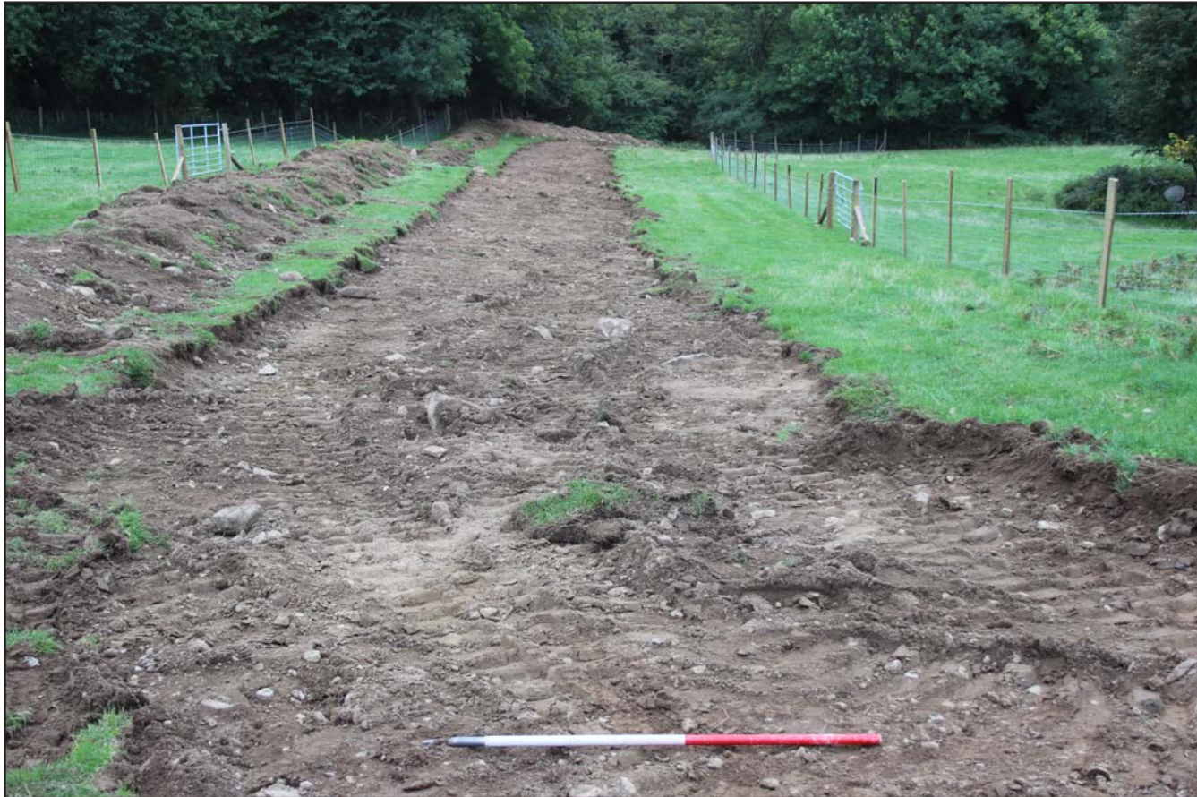
Plate 30: Topsoil strip within Field F (downslope) - Route 1 - from the northeast - scale 1m
