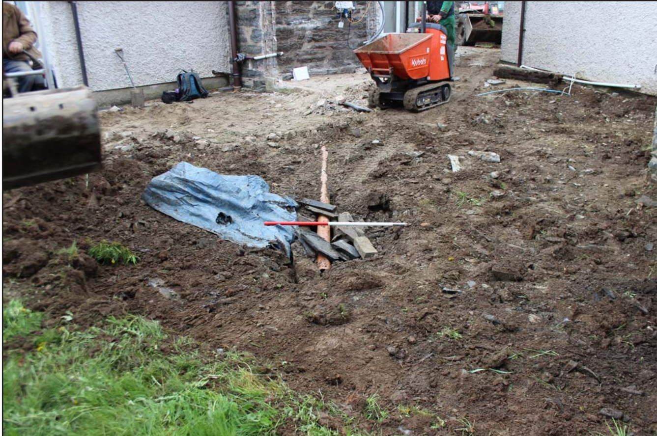
Plate 03: Working shot showing modern soakaway cut into (103) - from the north - scale 1.00m
