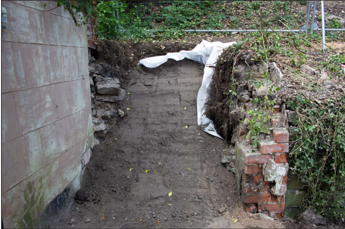
Plate 26: Test Pit 4 closed down and backfilled following archaeological work, Bailey Hill, Mold, Flintshire - from the southeast - no scale
