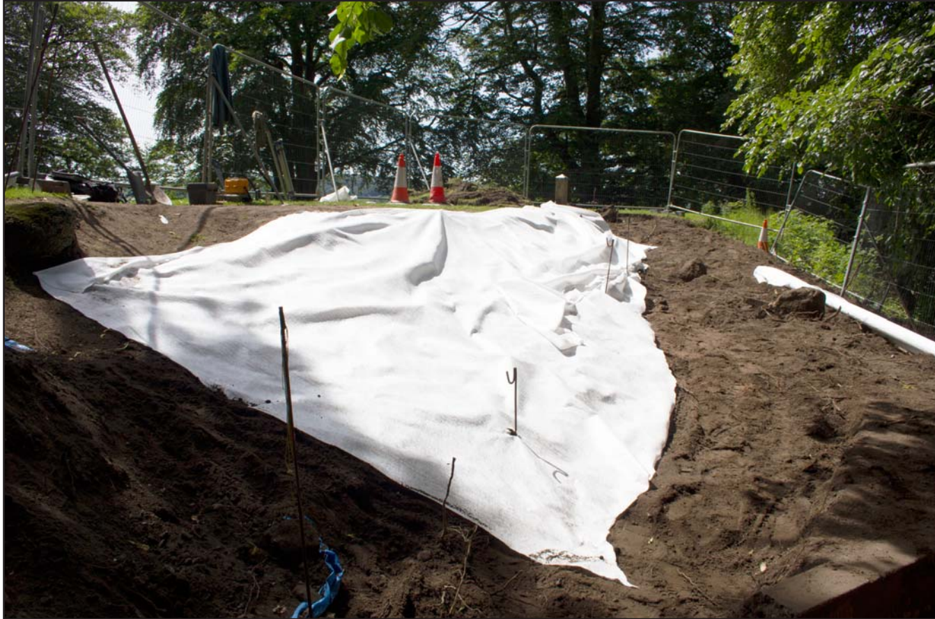
Plate 41: Terram placement and closing down shot on slope (western part) of Outer Bailey access ramp excavation - Bailey Hill, Mold, Flintshire - from the west - scale 1m
