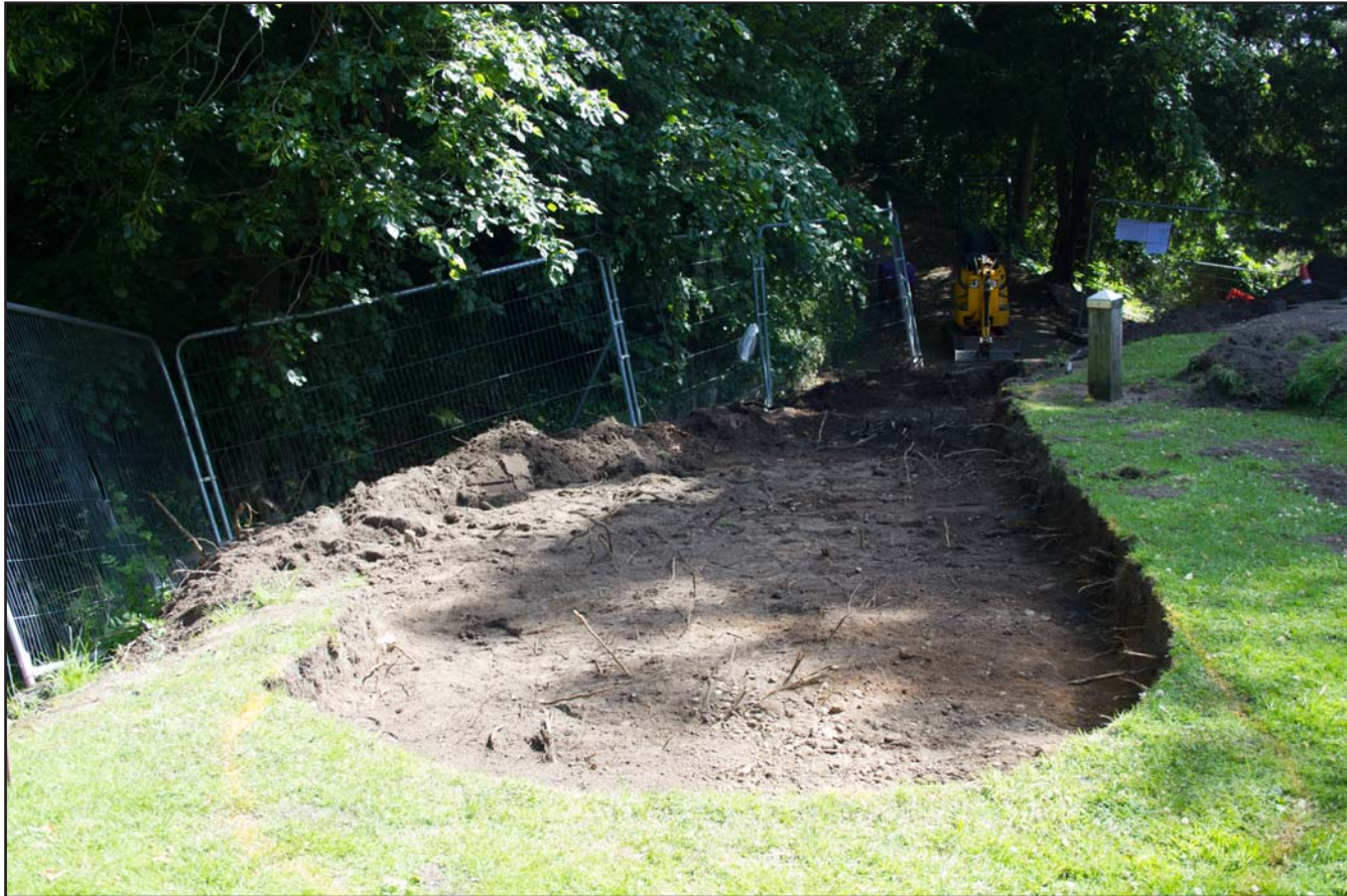
Plate 33: Post excavation of the upper portion (eastern) of the Outer Bailey access ramp excavation - Bailey Hill, Mold, Flintshire - from the east - scale 1m
