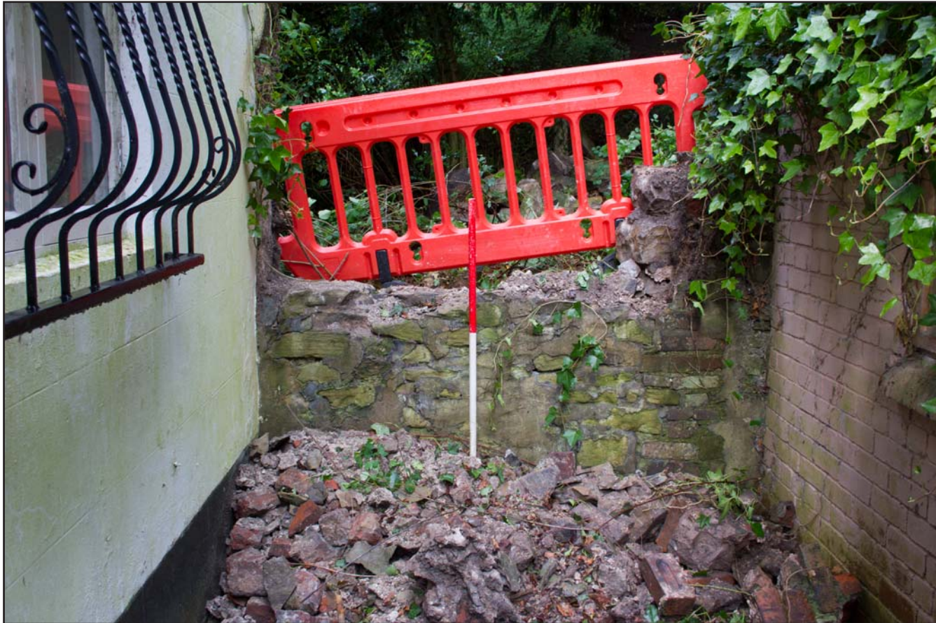
Plate 17: Pre excavation shot of Test Pit 6, Bailey Hill, Mold, Flintshire - from the northeast - scale 1m
