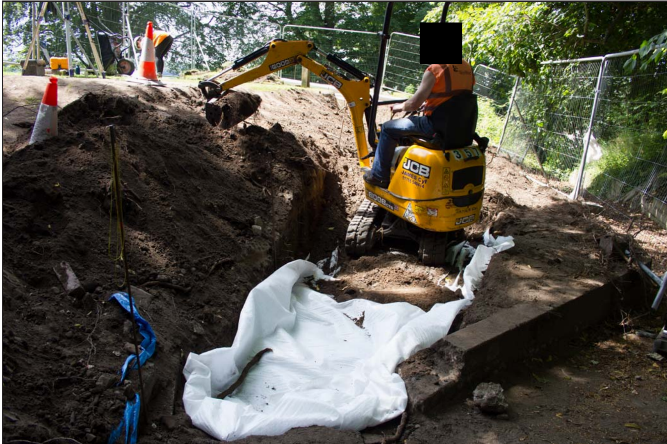
Plate 40: Terram placement and closing down shot on ramp incline of Outer Bailey access ramp excavation - Bailey Hill, Mold, Flintshire - from the west - scale 1m
