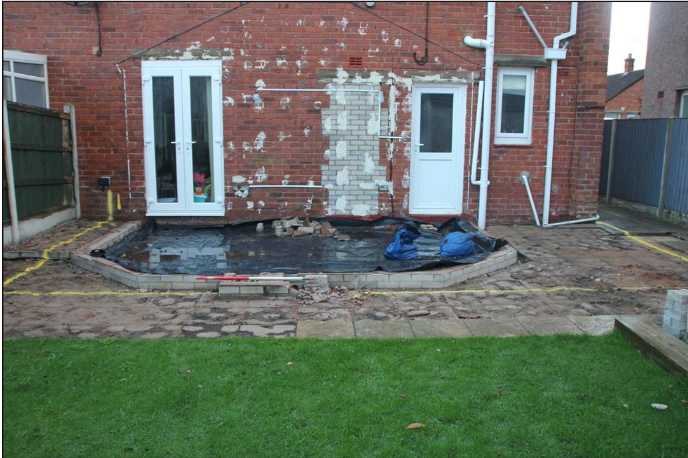
Plate 02: Pre-excitation photograph of site of proposed extension at 15 Harding Avenue, Rhuddlan, from the south. Scale 1.0m.
