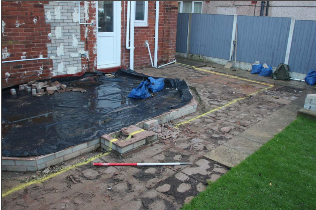
Plate 03: Pre-excitation photograph of site of proposed extension at 15 Harding Avenue, Rhuddlan, from the southwest. Scale 1.0m.
