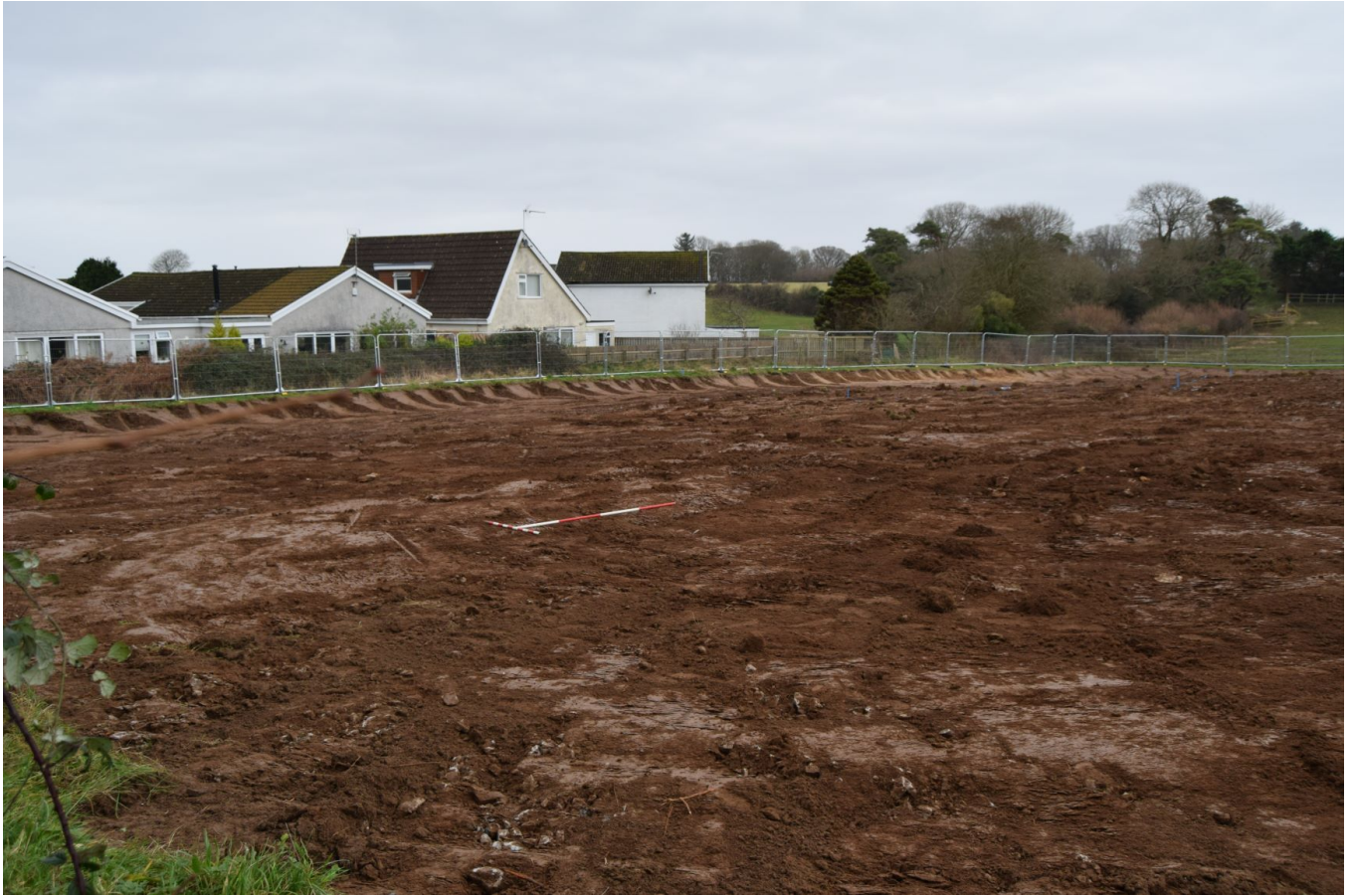
Plate 11. Topsoil (1000) removed from northern area of site, facing north-east, 1m & 2m scale.
