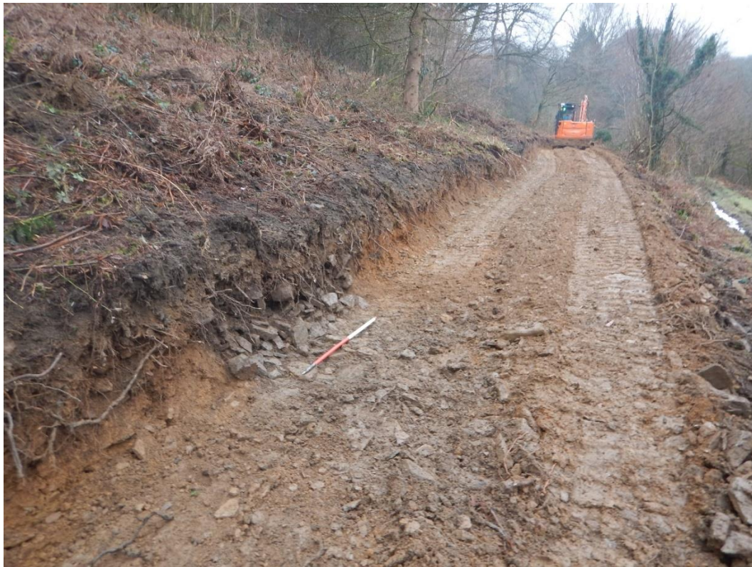
Photo 4: View west along the Phase 1 cabling route, with feature [004] visible. 1m scale.
