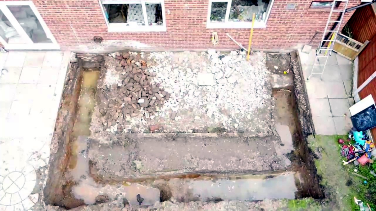
Aerial shot of the trenches. (North is to the left). Alan Wilmhurst
