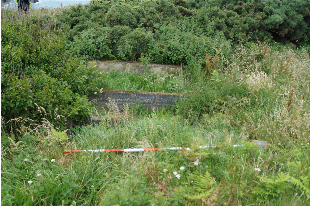
Plate 11: PEN2020_111. A view of the concrete base of an old shed or greenhouse in the garden of Pencastell cottage. It is located in the ditch of the promontory fort. Looking west.
