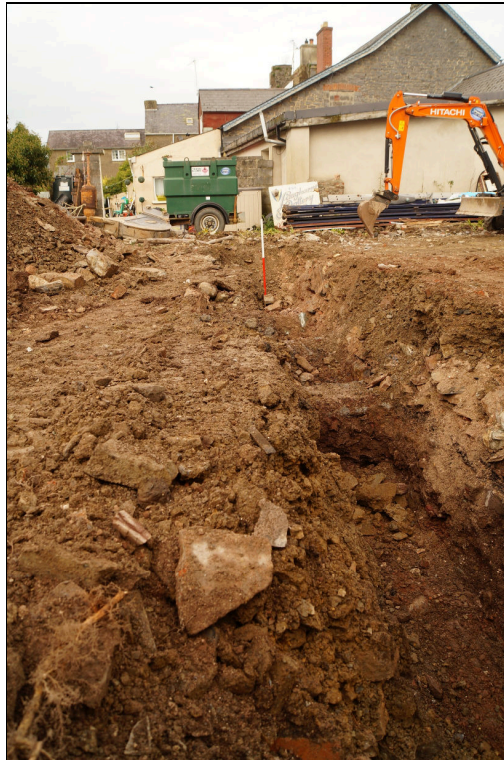
Plate 15: OPL2019_115, (003) Trench C showing concrete strips (003), and (006) below and in base of section, looking north.
