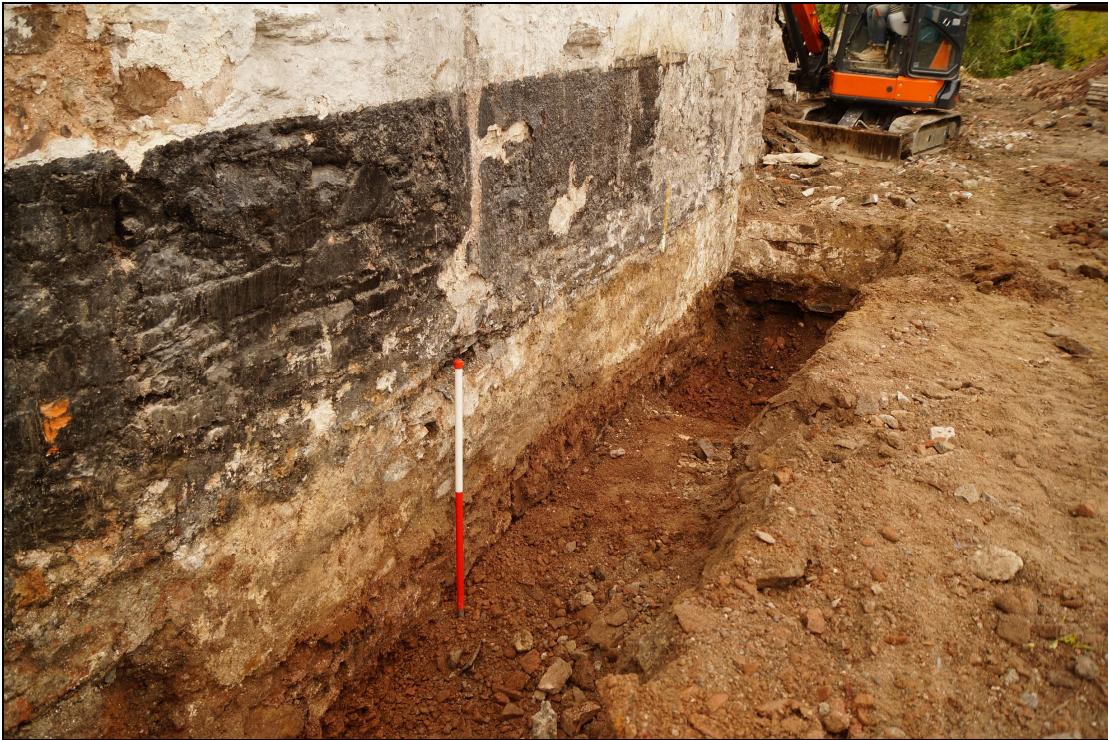
Plate 5: OPL2019_105, Trench A excavated alongside the adjoining wall of The Pelican to the south, looking west-southwest. Wall (008) can be seen across the far end of the trench abutting the north gable wall of The Pelican.
