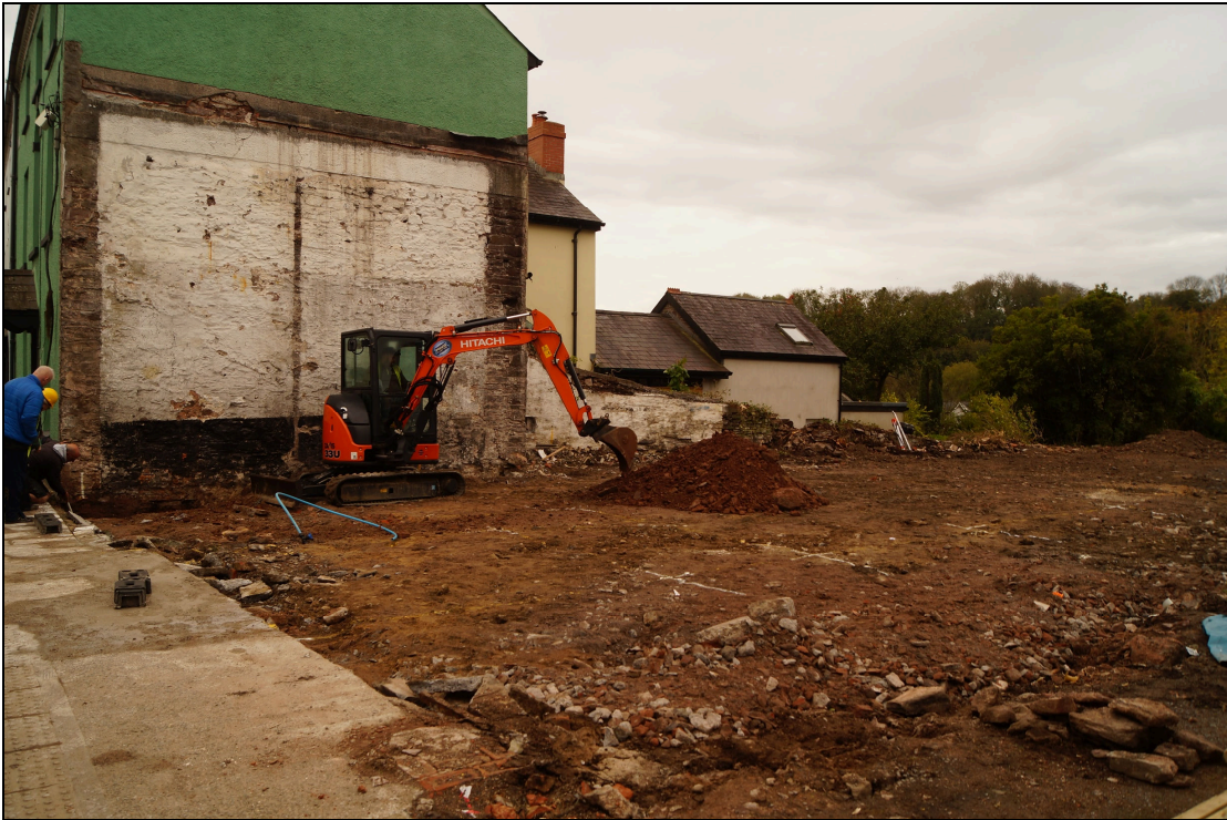
Plate 1: OPL2019_101, General view of the area where Unit 1 will be located. The former bus depot/pottery had previously been demolished and the area levelled with some of the debris, looking south-southwest.
