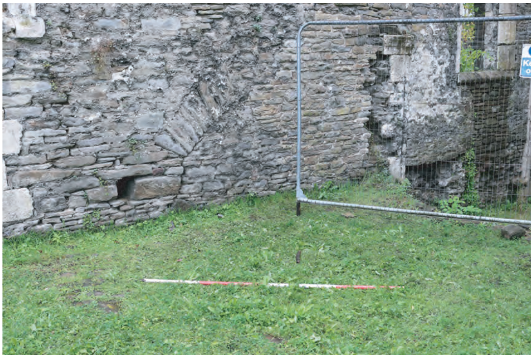
Plate 04. Area 1 - Detail of blocked opening in north end of west facing external elevation of Reredorter (Latrine Range). Looking southeast.
