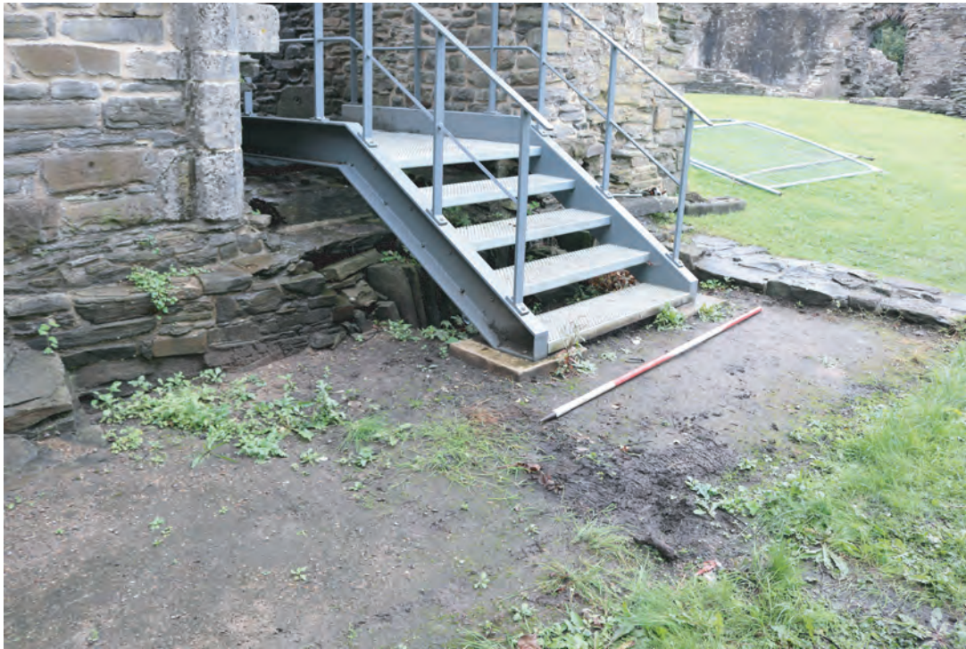
Plate 03. Area 1 - Oblique view of modern steel steps covering former opening to cell or basement area below slype passage at northern end of Dorter / Undercroft. Looking northwest.
