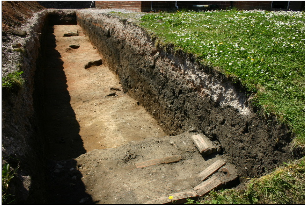
Fig. 6. Trench 1, viewed from the east, with the electricity cables in the foreground. Photo CPAT 3460-0046
