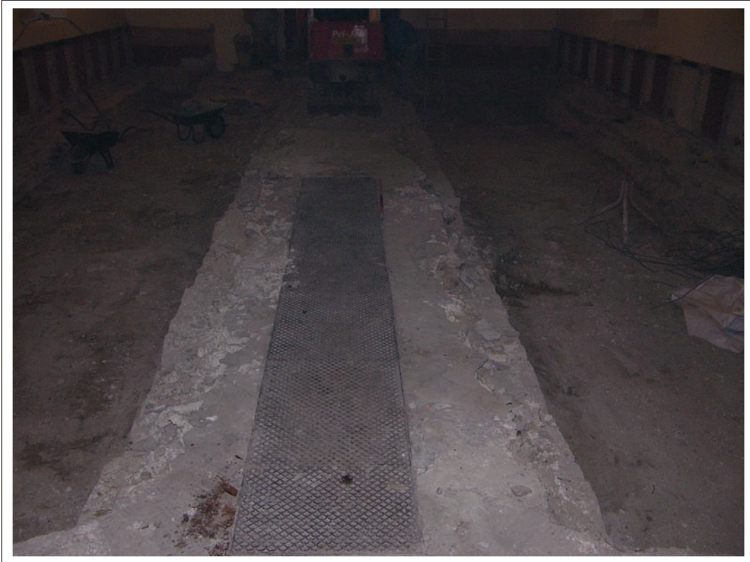
Plate 1: View of hollow areas (cavities) in nave located either side of the central aisle. Note heating grills in foreground located directly above flu in central aisle. Scale 1x1m
