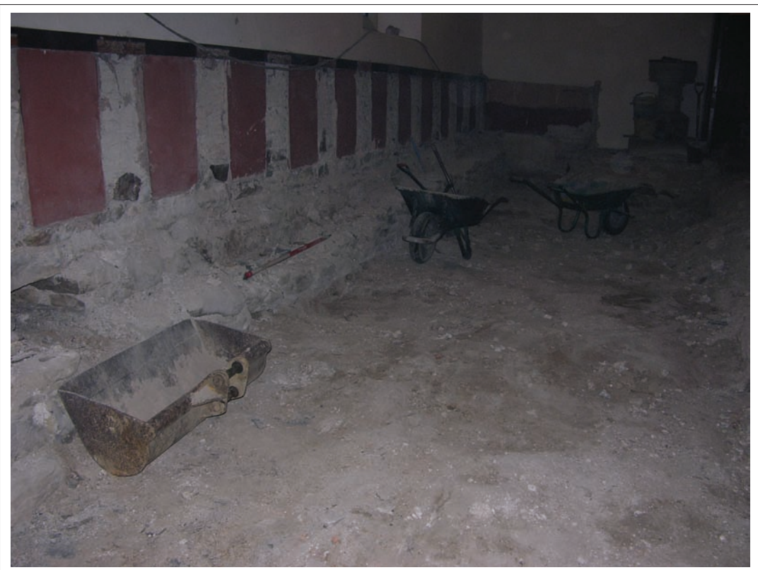
Plate 2: View of church wall foundation level, exposed after removal of floorboards, joists and rubble fill from hollow area. Scale 1x1m
