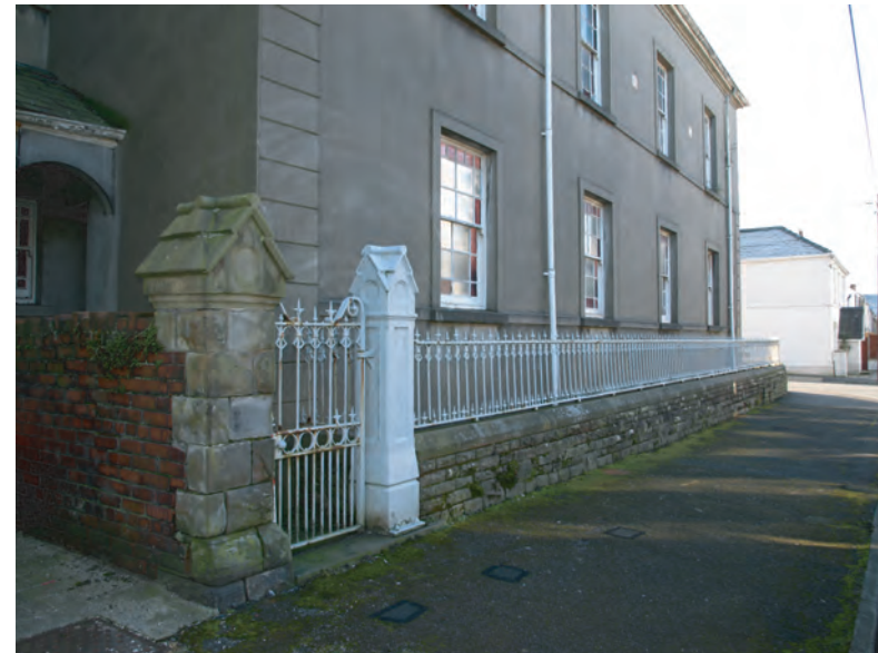
Plate 8. Siloh Chapel (1910). Detail of railings surrounding chapel on western side. Looking south.
