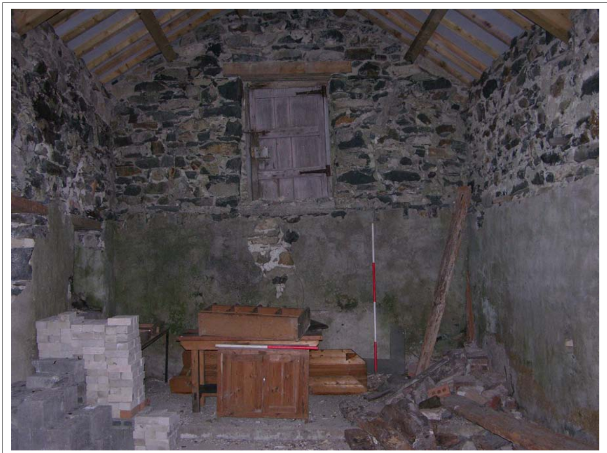
Plate 27: Internal view of Building two, note doorway leading to stairs in wall, Scales 1x1m & 1x2m
