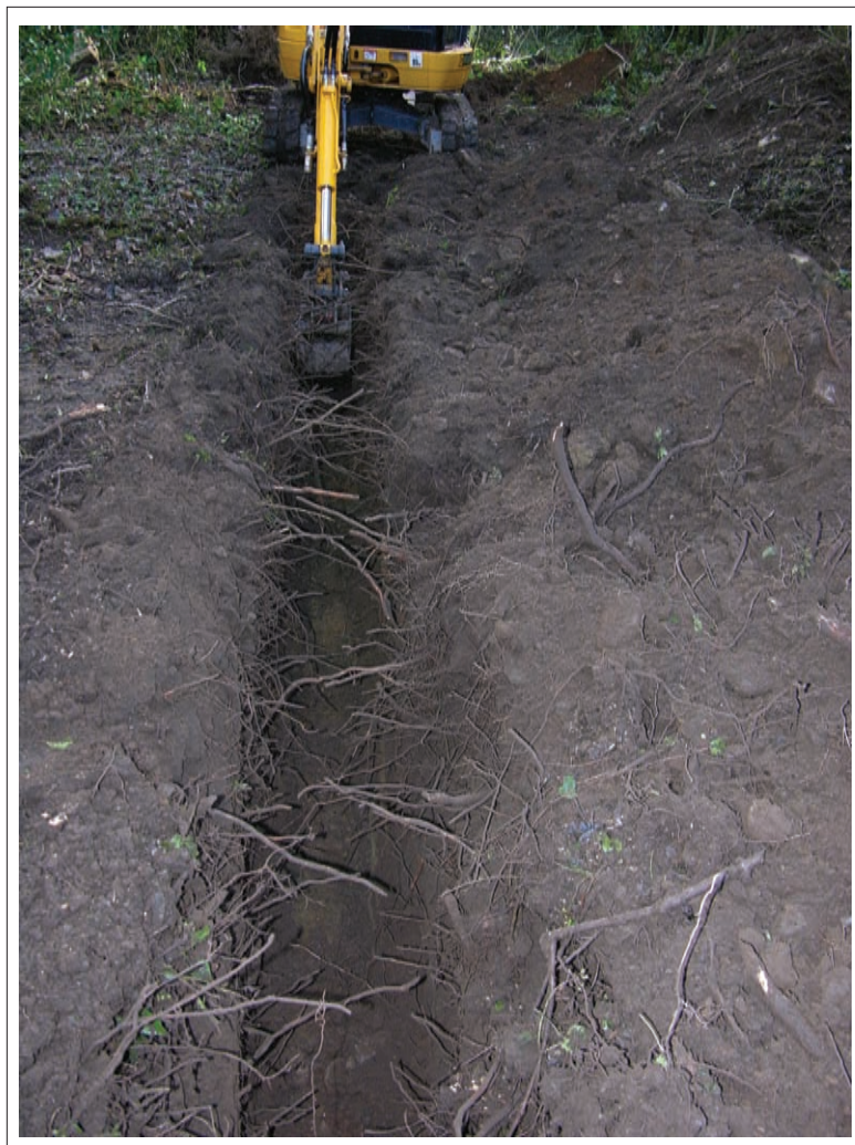
Plate 3: View of drain run into biodisc soakaway. Natural levels observed at similar depth
