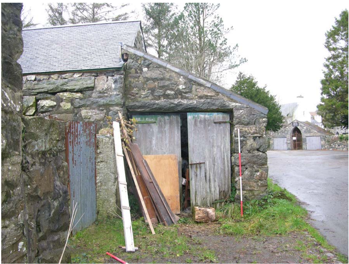
Plate 17: External view of further additional structure, note butt joint, Scale 1x2m
