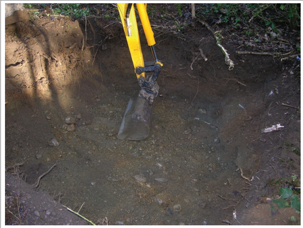
Plate 2: View of biodisc soakaway area, showing natural at a depth of approximately 0.5m
