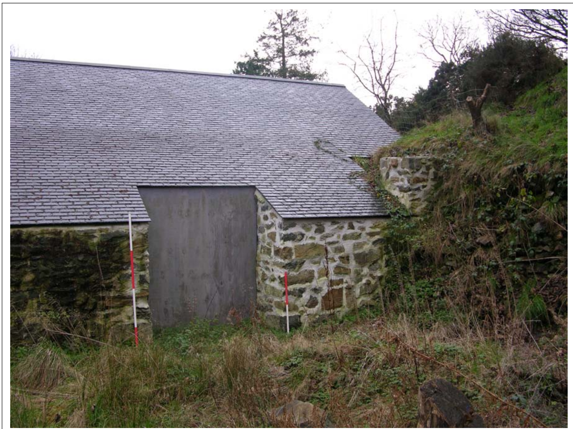
Plate 21: External view of rear of additional structure, Building one, showing where building butts against the motte, Scale 1x1m & 1x2m
