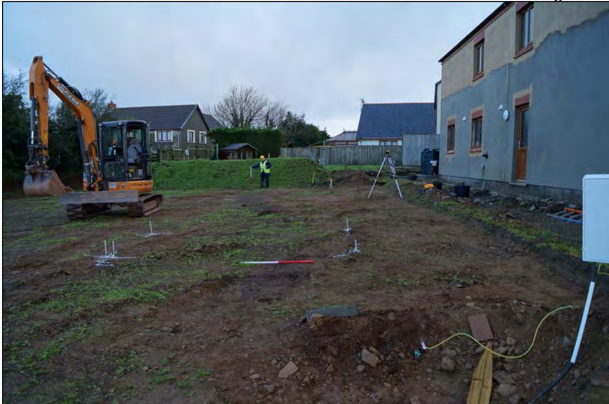
Plate 3: HMN2015_103, Site cleared of topsoil, with ditch HMN2015_003 clearly visible, taken from south end of the plot, looking north northeast.
