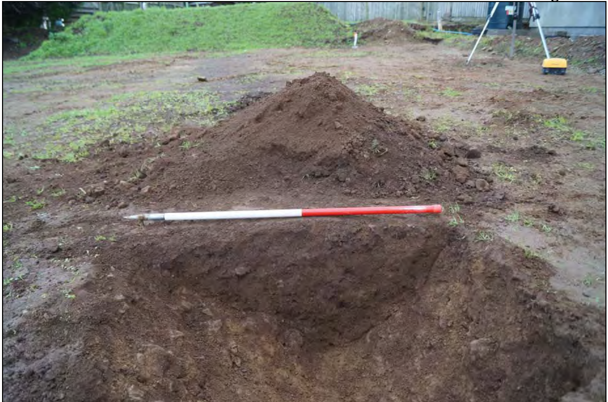
Plate 5: HMN2015_105, section across ditch where the northeasternmost wall foundation was to be placed, looking north northeast.
