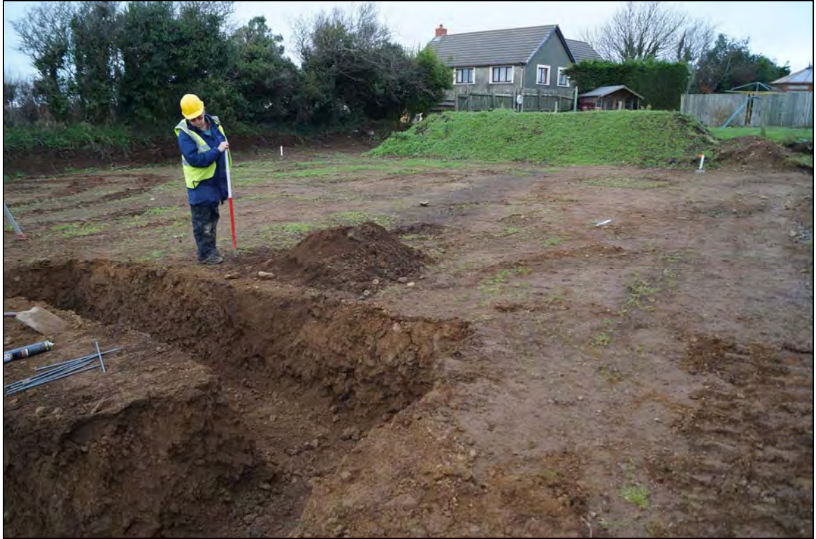
Plate 11: HMN2015_111, part of HMN2015_003, previously excavated by hand by Trydor, see Plates 5, 6 & 7, showing in section after mechanical excavation of wall foundations, looking northwest.
