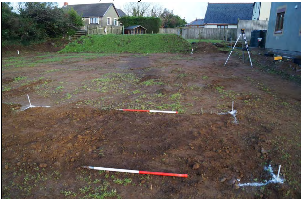
Plate 4: HMN2015_104, Site cleared of topsoil, with ditch HMN2015_003 clearly visible, taken from south end of the plot, section of ditch through which house foundations were be cut cleaned, looking north northeast.
