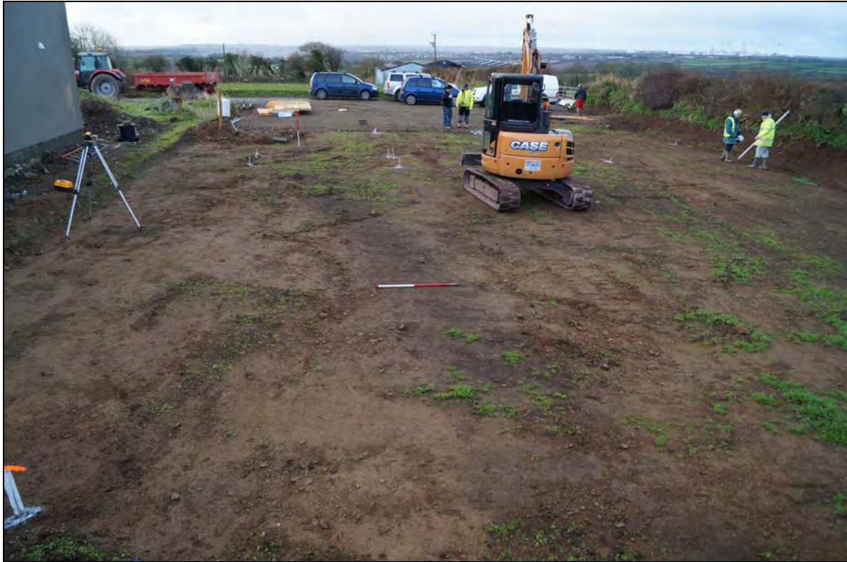
Plate 1: HMN2015_101, Site cleared of topsoil, with ditch HMN2015_003 clearly visible, taken from a pile of topsoil at the north end of the plot, looking south.
