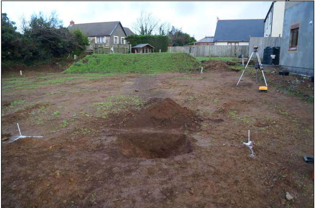
Plate 7: HMN2015_107, the excavated section of the ditch, without scales, looking north northeast.
