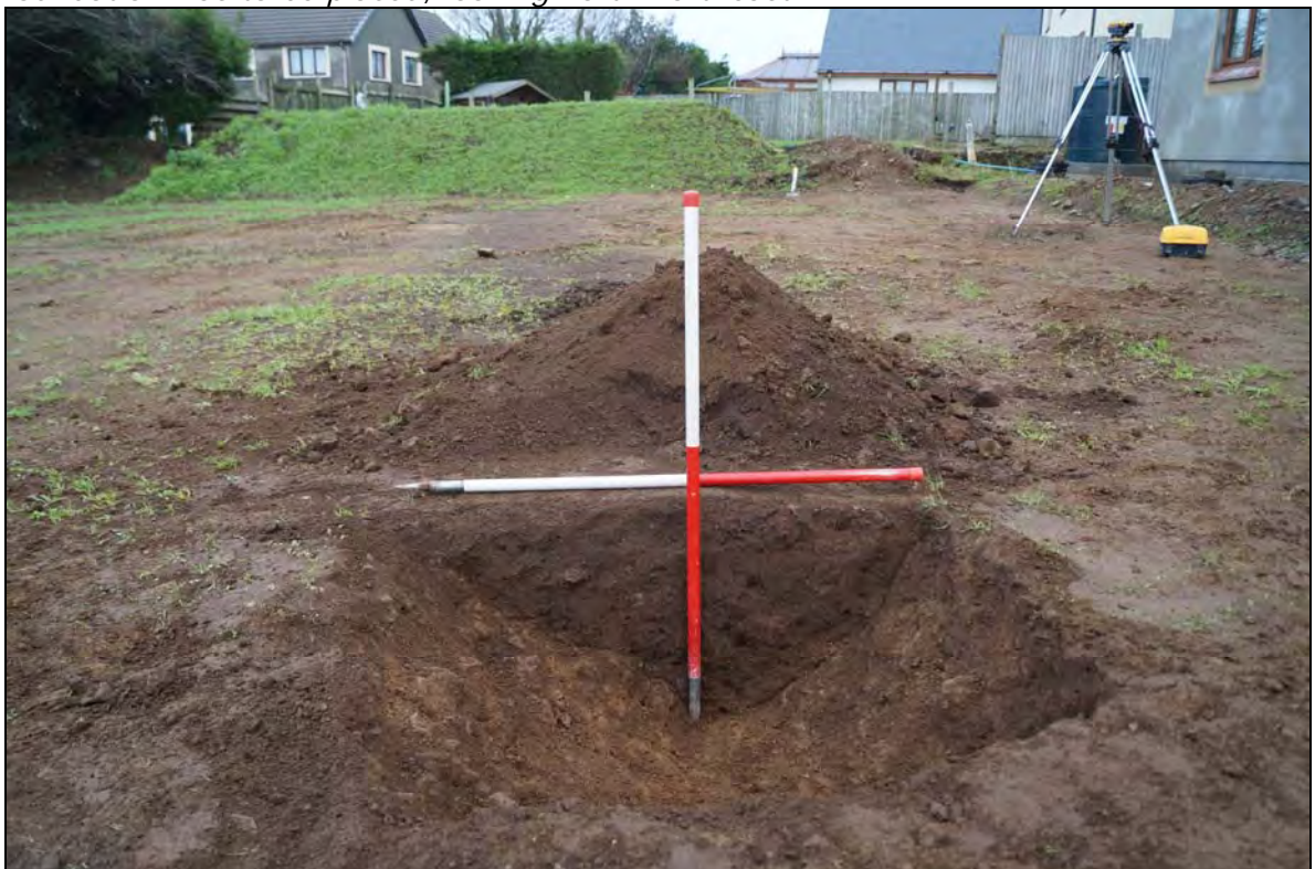
Plate 6: HMN2015_106, section across ditch where the northeasternmost wall foundation was to be placed, looking north northeast.
