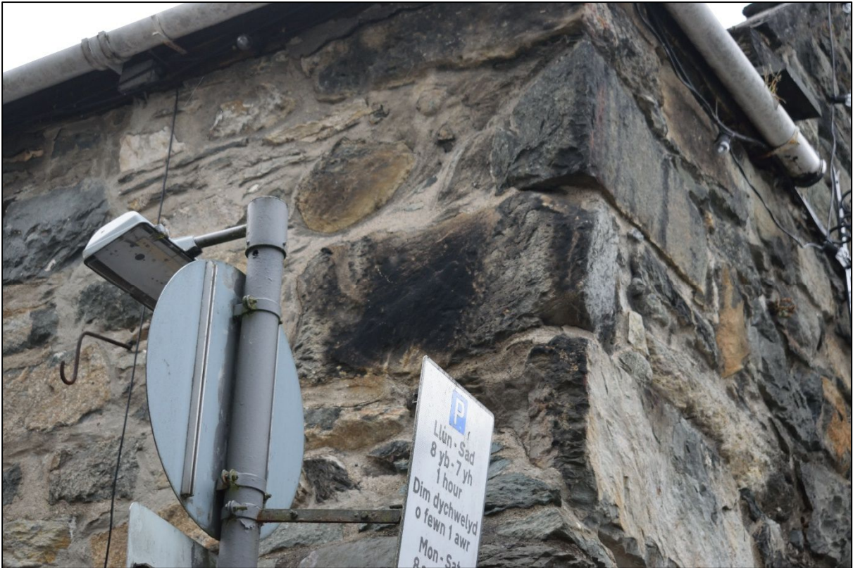
Plate 7: Sooting on the eastern end of the southern elevation
