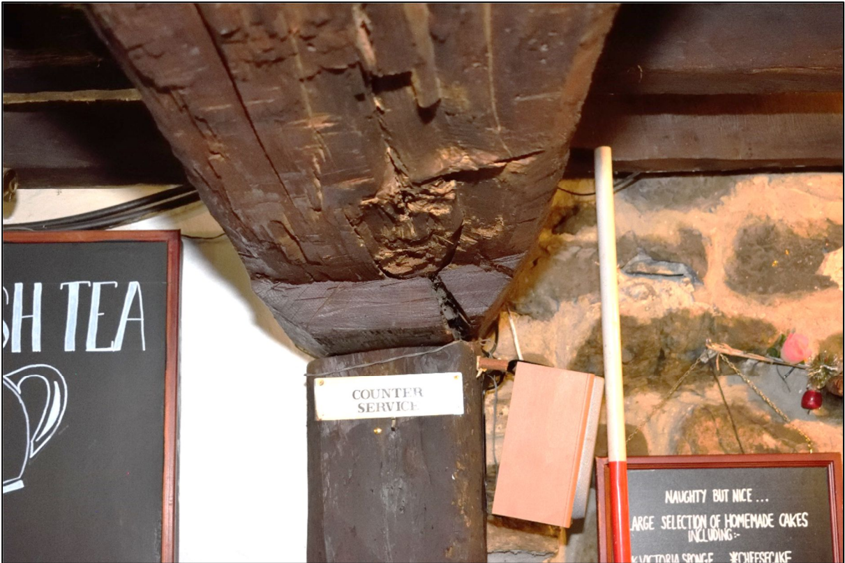
Plate 21: Underside of one of the ceiling beams in the tearoom, showing the thinning
