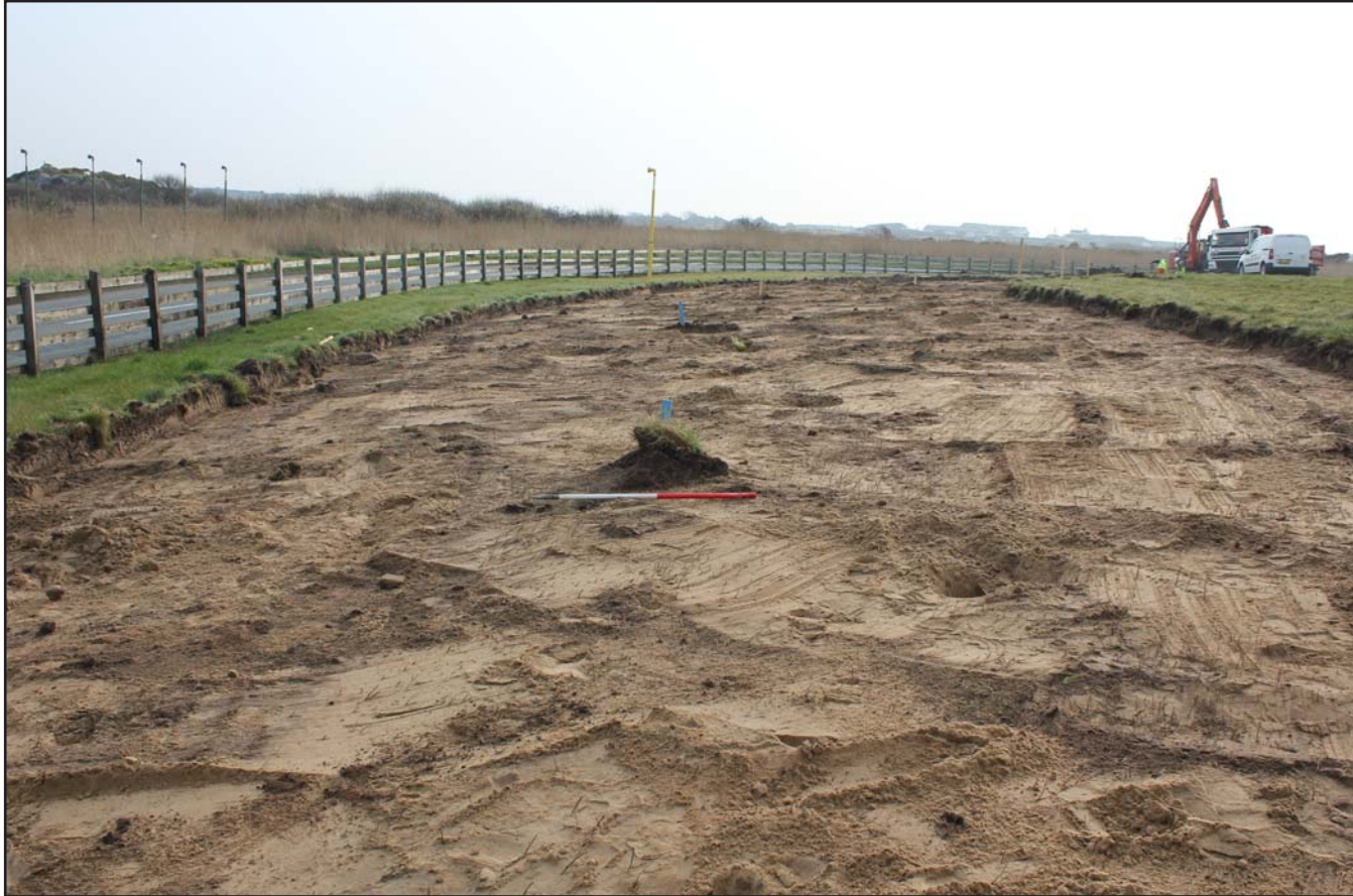
Plate 26: Perimeter road topsoil strip to north of Runway 19 (200.0m to 250.0m) - from the west - 1m scale
