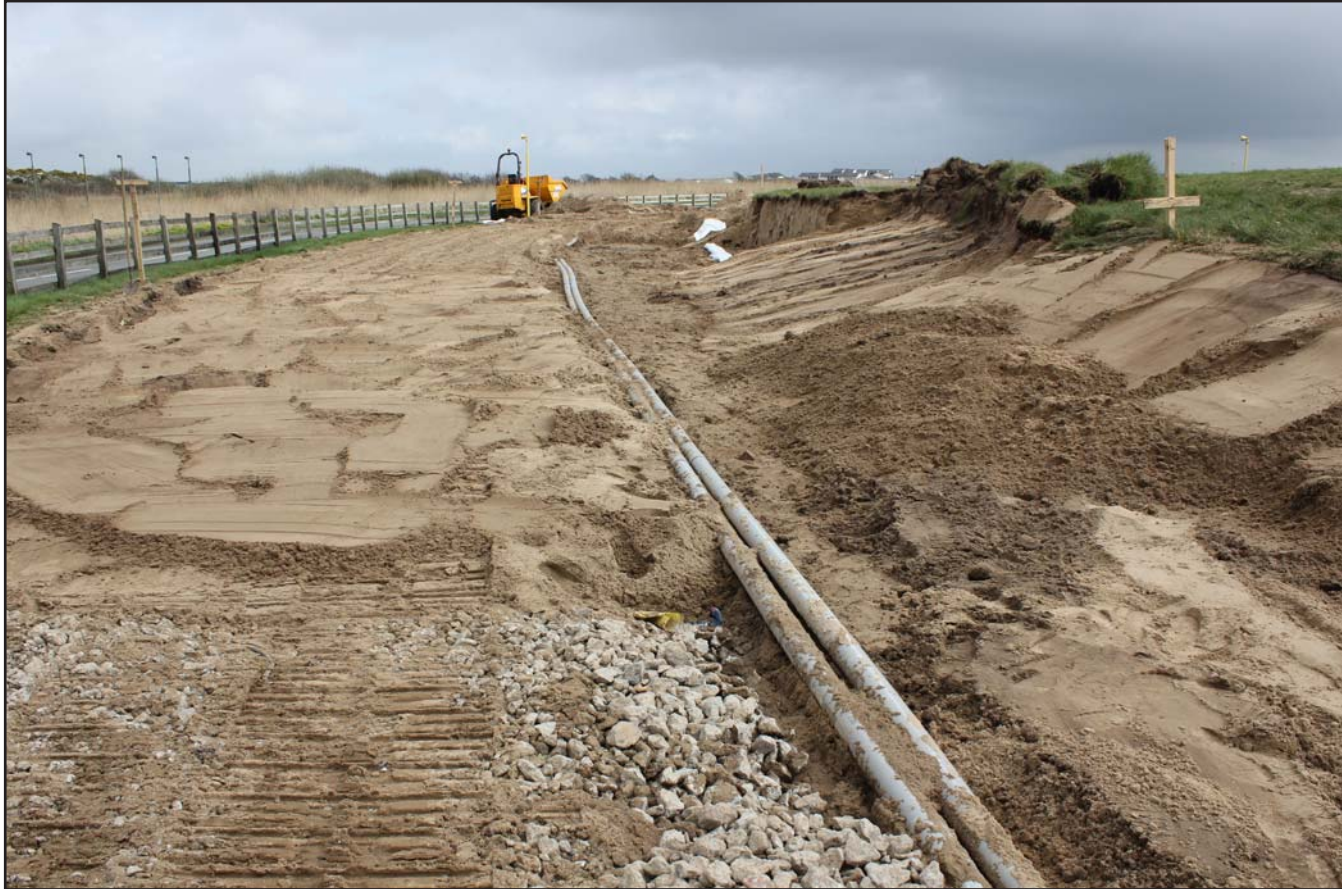
Plate 28: Batter ahead of temporary shut down ahead of reopening of Runway 19 (lowered services also shown) - from the west - no scale
