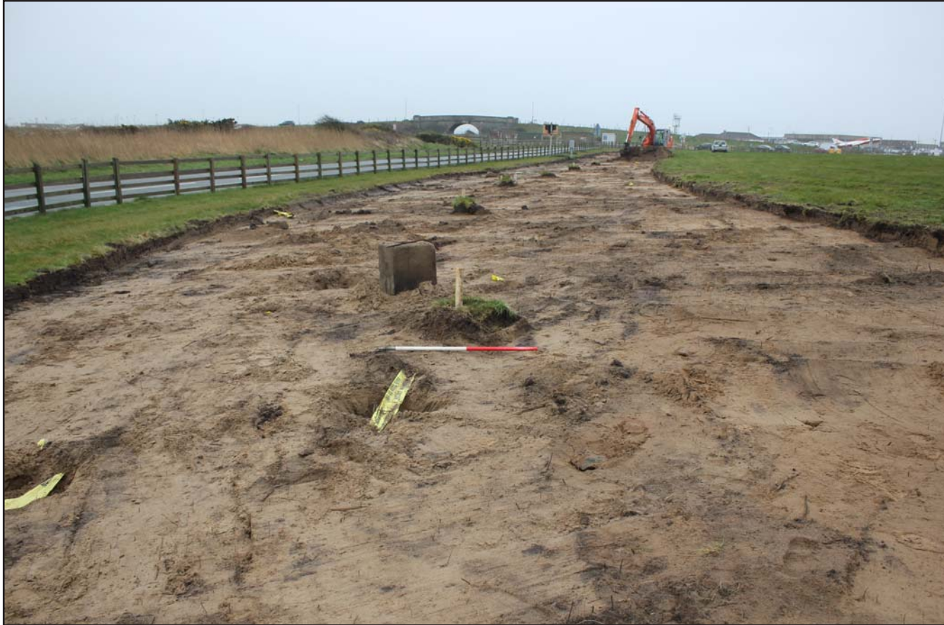
Plate 29: Perimeter road topsoil strip to north of Runway 19 (350.0m to 450.0m) - from the northwest - 1m scale
