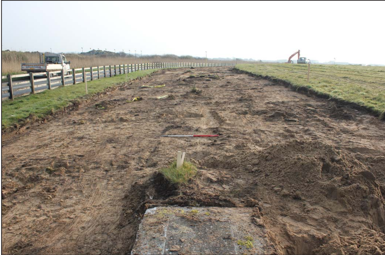
Plate 25: Perimeter road topsoil strip to north of Runway 19 (130.0m to 200.0m) - from the west - 1m scale
