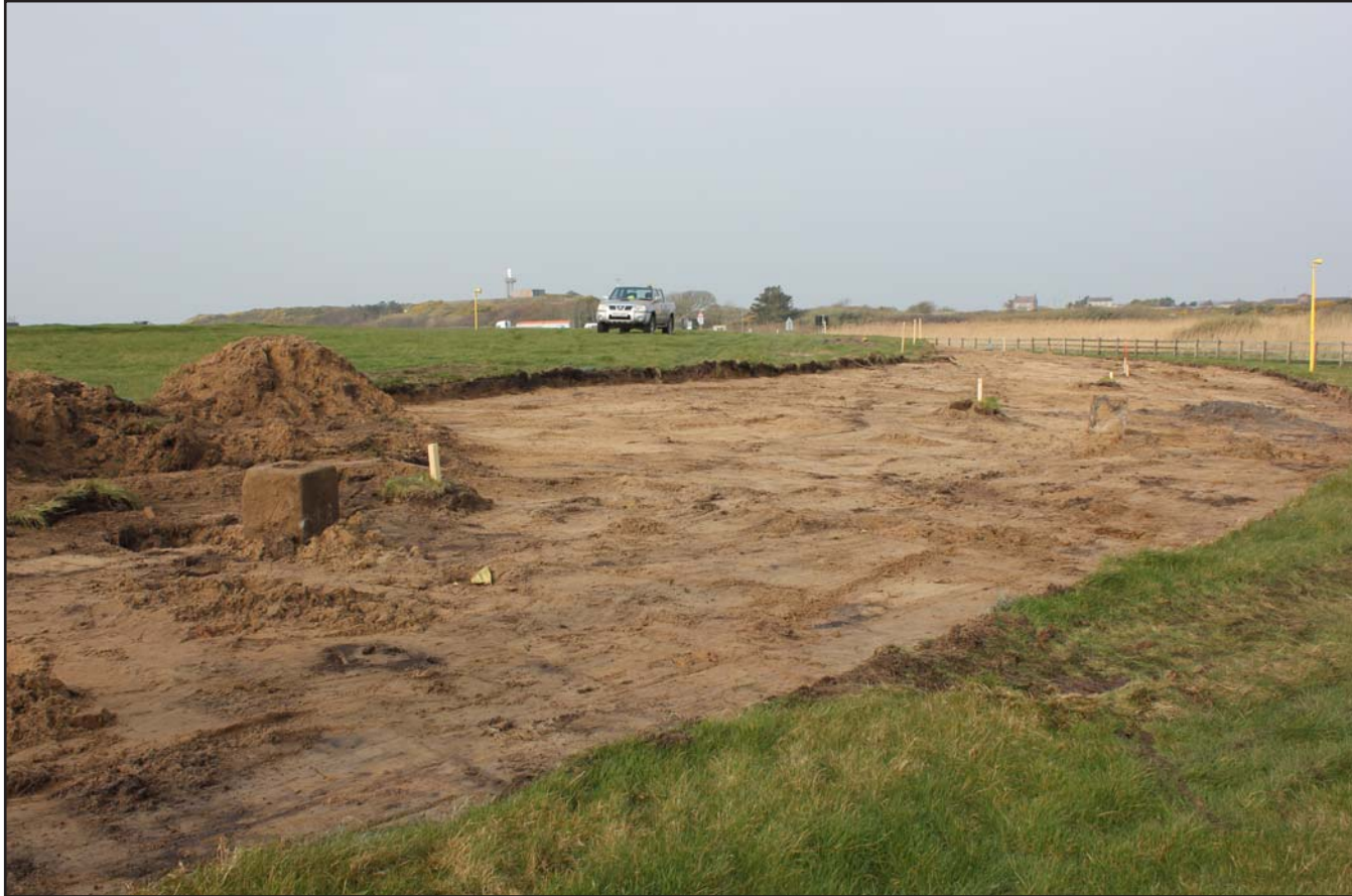
Plate 27: Perimeter road topsoil strip to north of Runway 19 (Oblique shot -250.0m to 200.0m) - from the east - 1m scale
