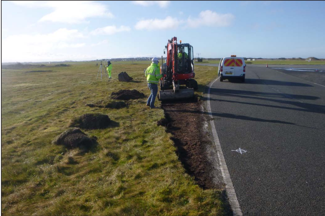
Plate 01: Commencement of Cycle path North (towards taxiway Alpha) - from the northeast - no scale
