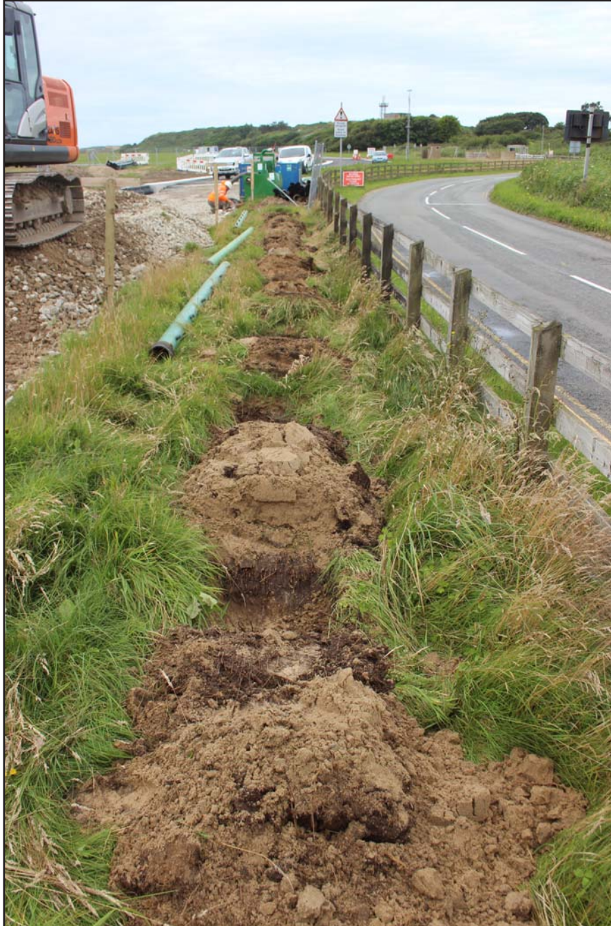
Plate 38: Test pits along northern edge of perimeter road - from the west- 1m scale
