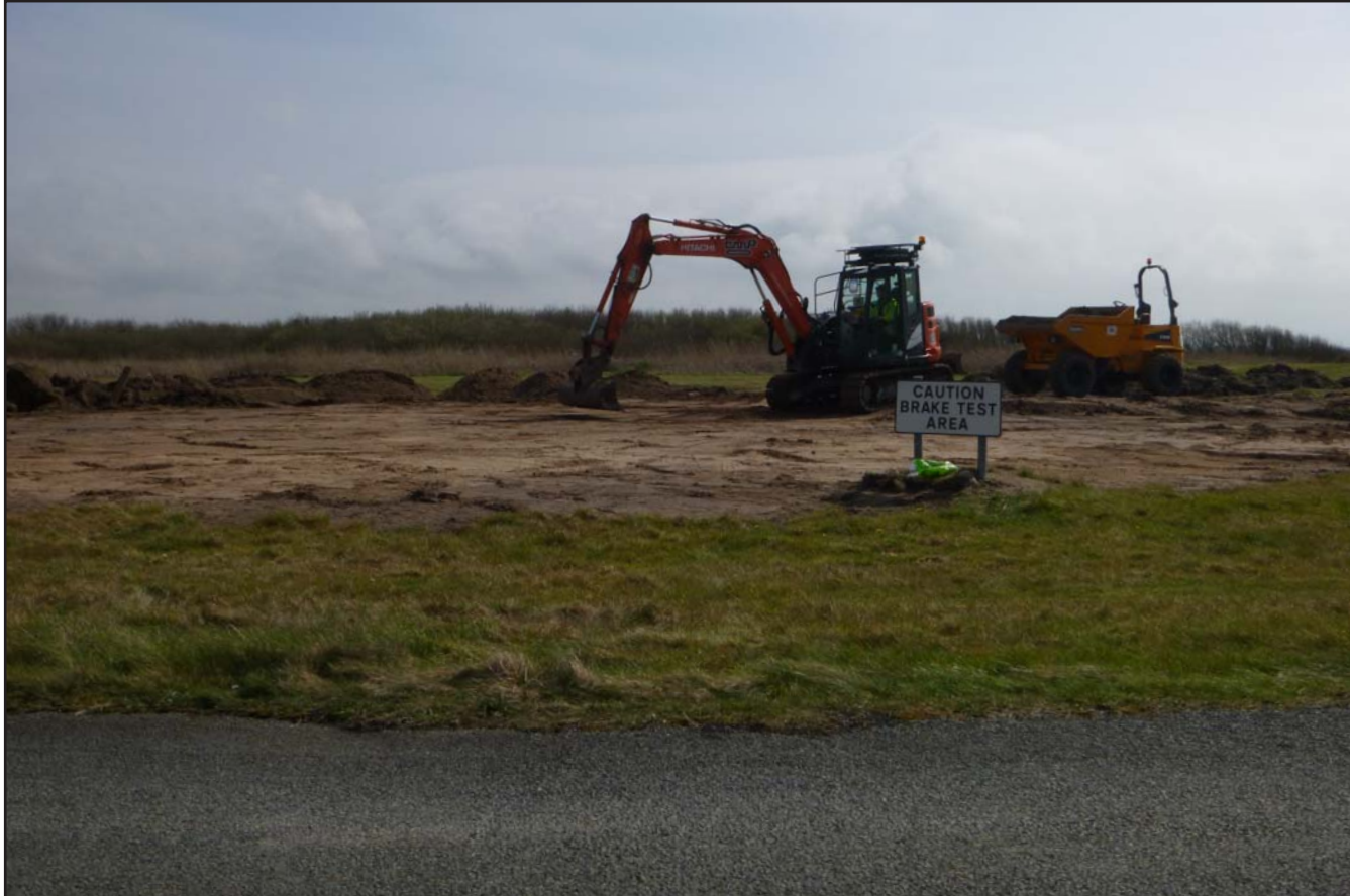
Plate 16: Brake Test Area - reduced dig on 'golf-tee' and south eastern quadrant of compass calibration base (CCB) - from the west - no scale
