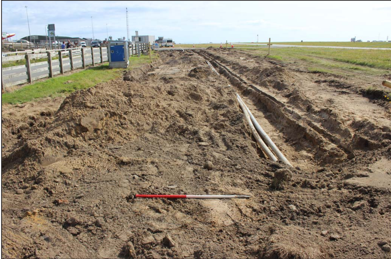
Plate 32: Perimeter road topsoil strip to north of Runway 19 (550.0m to 600.0m) - from the north - 1m scale
