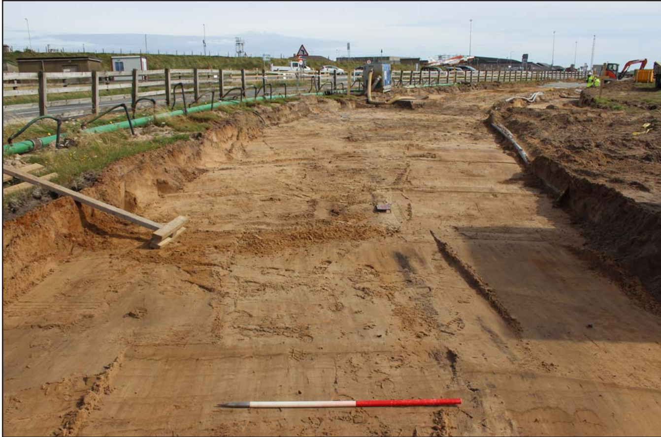
Plate 31: Perimeter road topsoil strip to north of Runway 19 (500.0m to 550.0m) - from the north - 1m scale
