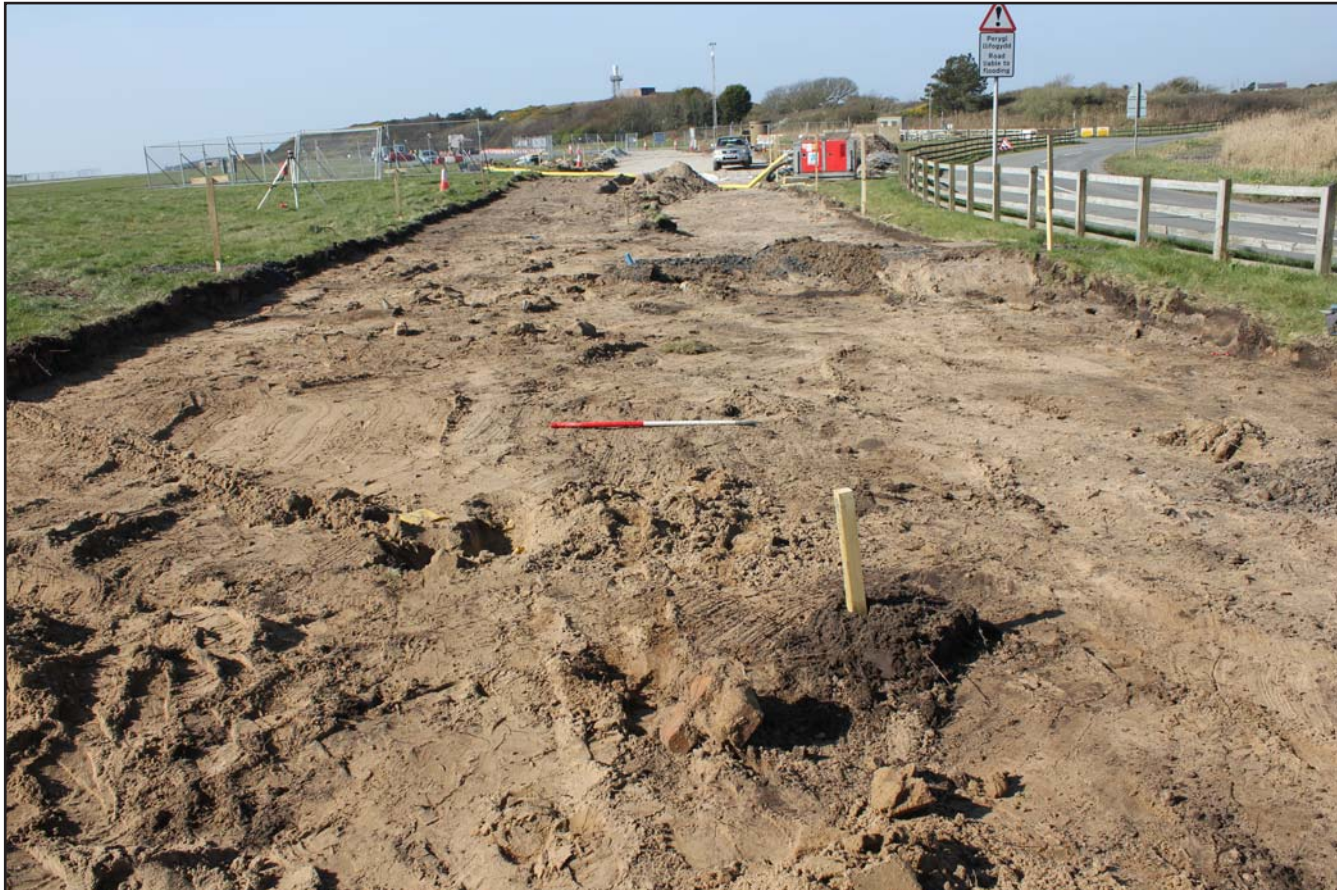
Plate 24: Perimeter road topsoil strip to north of Runway 19 (130.0m to 0m) - from the east - 1m scale
