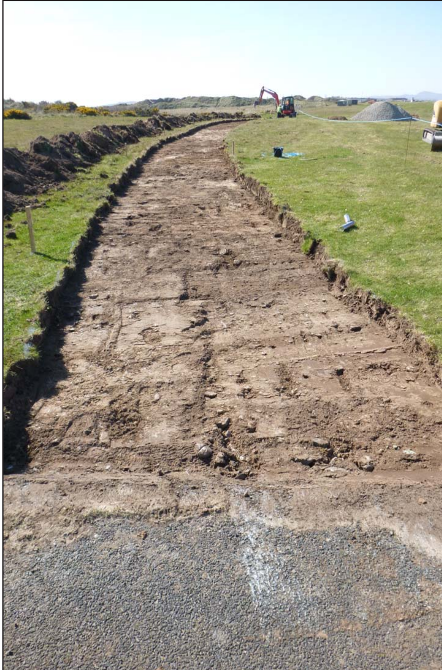
Plate 08: Commencement of Cycle path South (from Rhosneigr cycle path) - from the southeast - no scale
