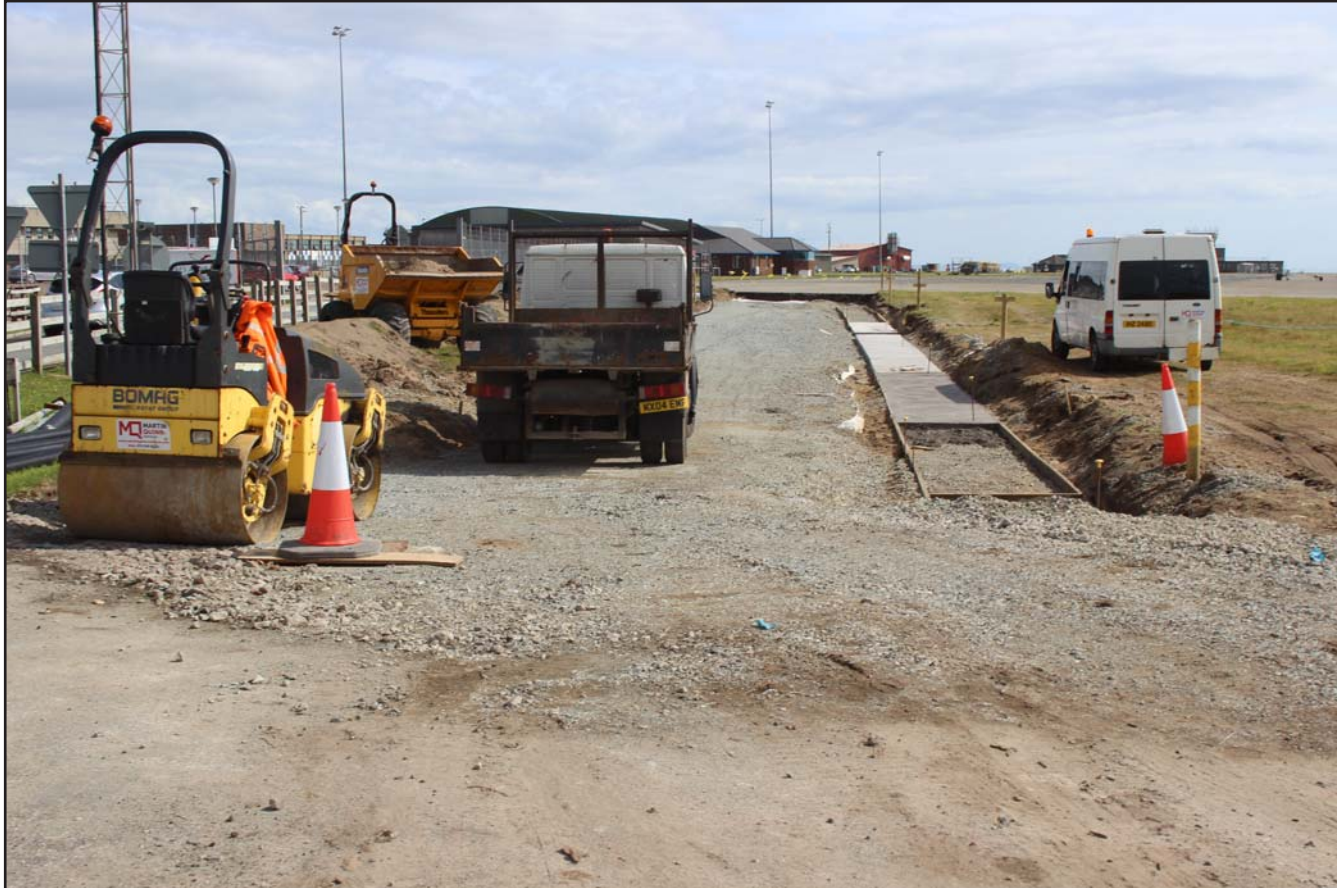
Plate 33: Perimeter road stoned up and concreted (600.0m to 650.0m) - from the north - no scale
