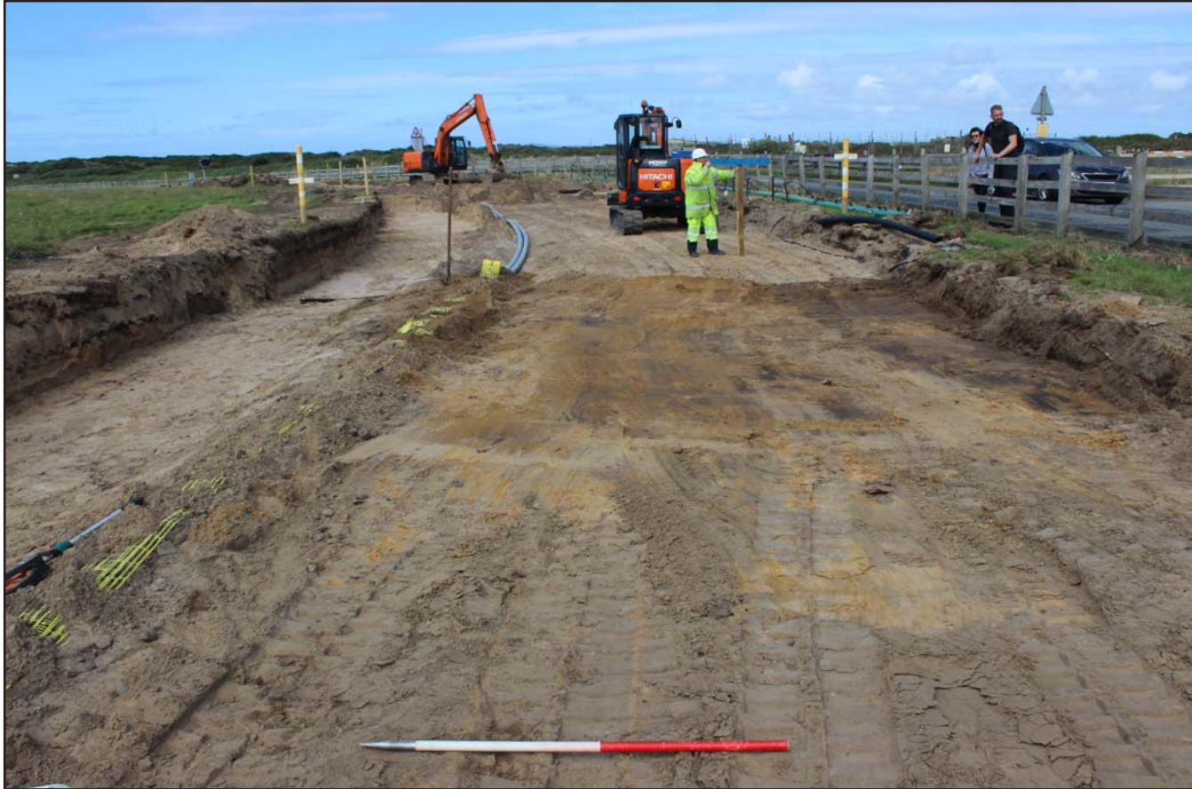
Plate 30: Perimeter road topsoil strip to north of Runway 19 (500.0m to 450.0m) - from the south - 1m scale
