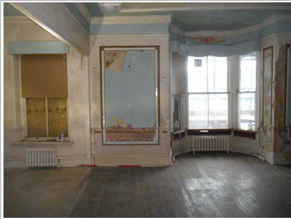
Plate 33. Detail of wall evidencing different layers of decoration, looking NW.
