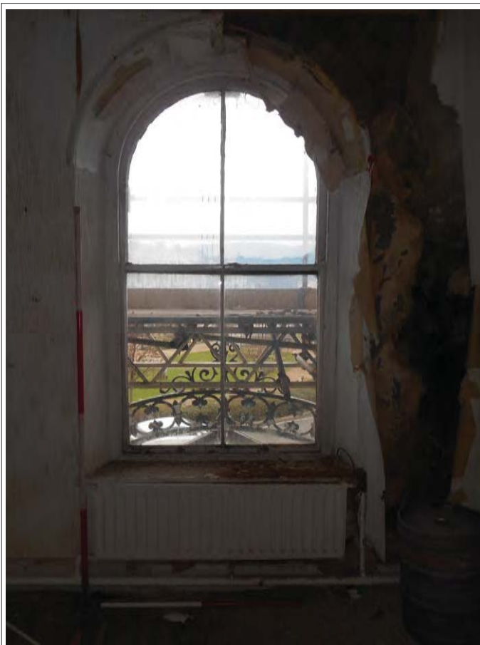
Plate 64. View of Room 6 with round headed sash window, above main entrance, looking W.
