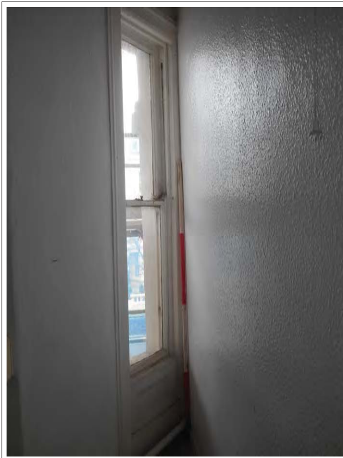
Plate 72. View of Room 7. Storeyed canted three-light window blocked by wall addition, looking N.
