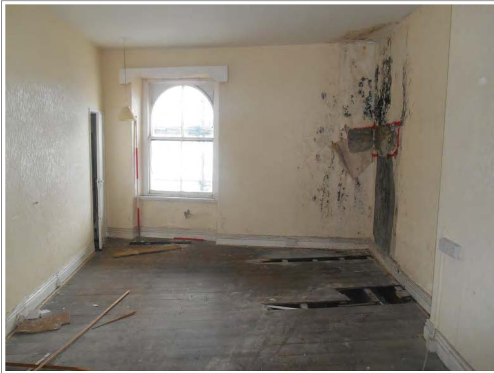
Plate 81. View of Room 1 with round-headed sash window and access to Room 11, looking SSW.
