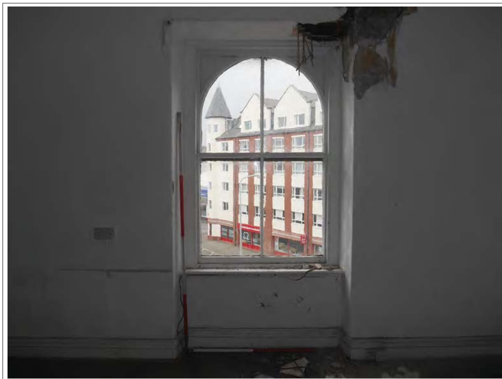
Plate 80. View of Room 11 with round-headed sash window and modern electrical fittings, looking SSE.
