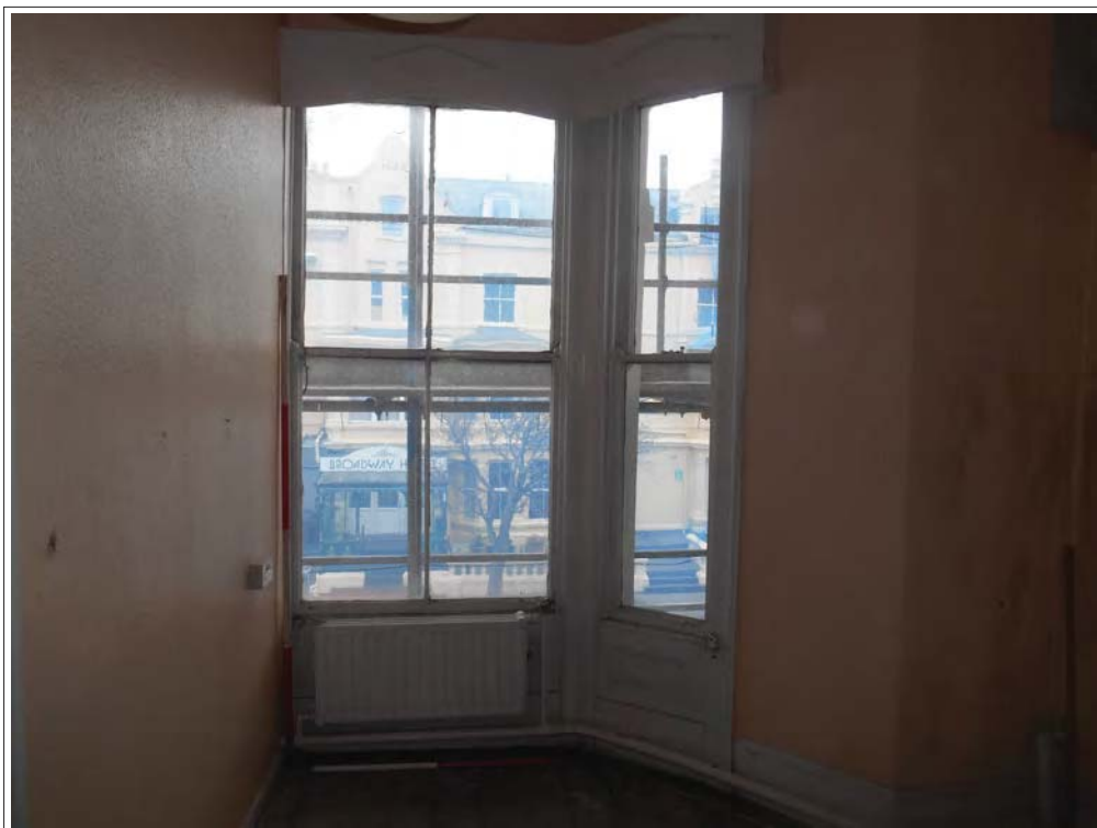
Plate 68. View of Room 8. Storeyed canted three-light window blocked by wall addition, looking N.
