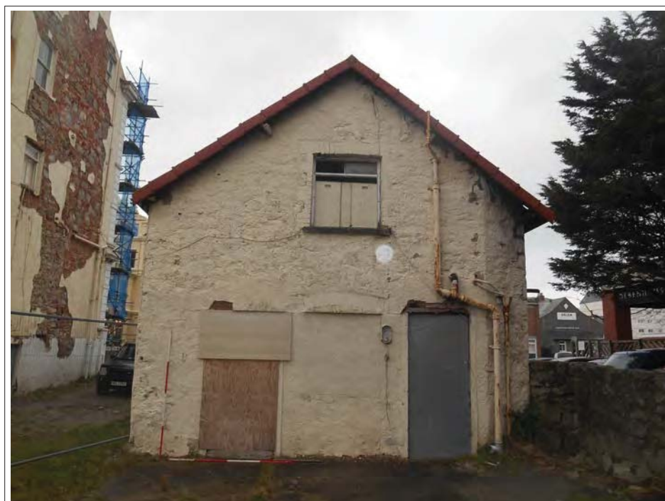
Plate 151. View of back entrance. Windows and doors are not original and demonstrate a number of alterations over time. 1960's hoods. First floor window with reveal toothed brick effect. Scales 2 x 2m
