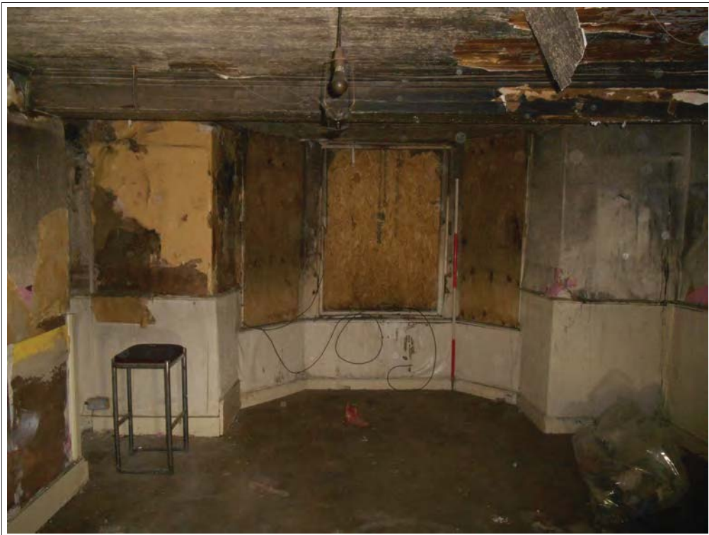
Plate 127. View of room affected by fire, looking NW.
