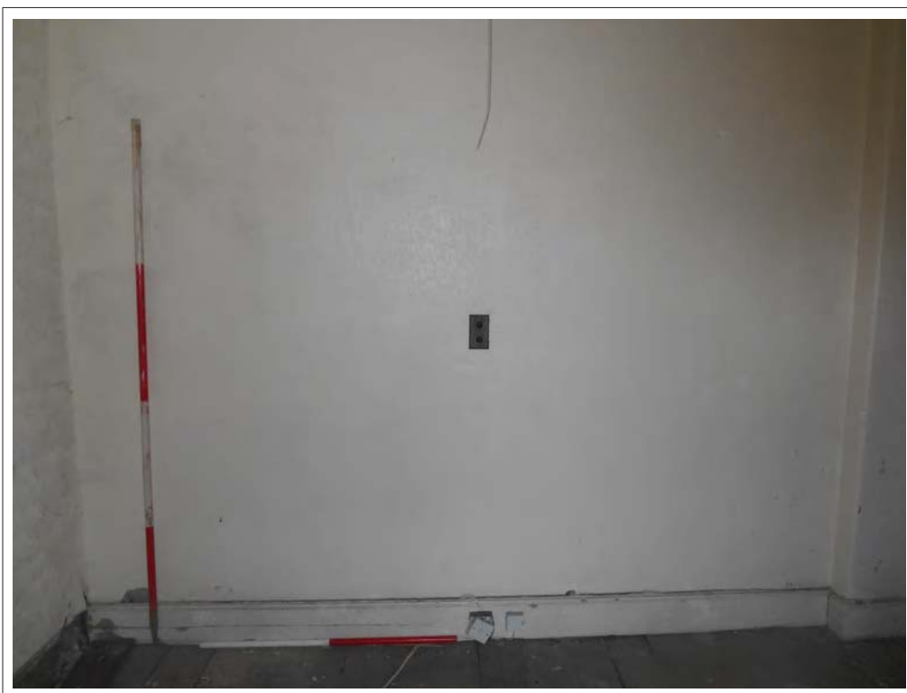
Plate 92. Detail of electrical fitting from Room 7, looking E.
