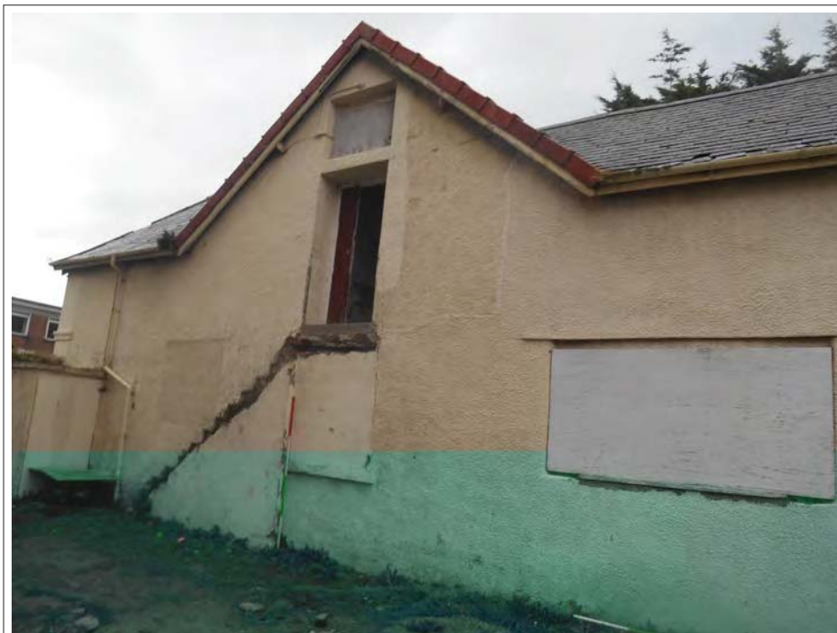
Plate 166. Detail of first floor door and exterior stair case, east facing wall.
