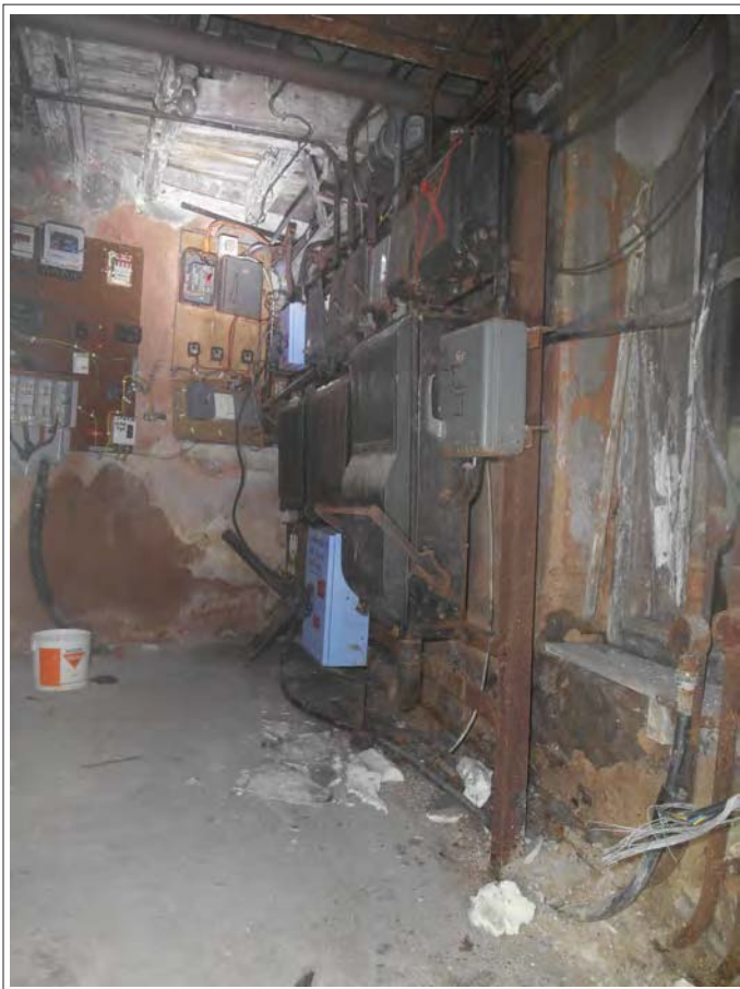
Plate 116. Meter room, looking S.
