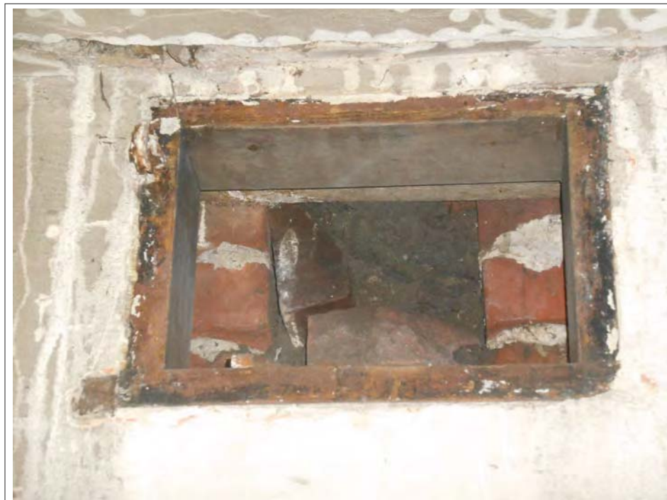
Plate 143. Blocked vent, west facing wall.
