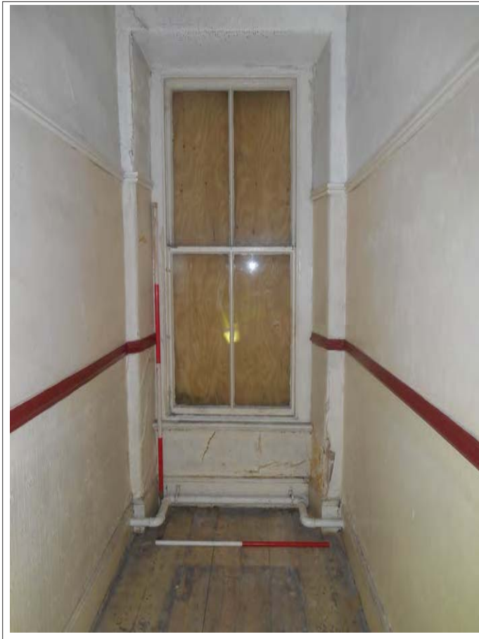
Plate 55. View of corridor looking SSE with centre bar sash window, looking SSE.
