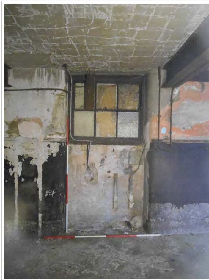
Plate 133. Remains of early door, subsequently transformed into a window which is currently blocked. Eastern facing interior wall.
