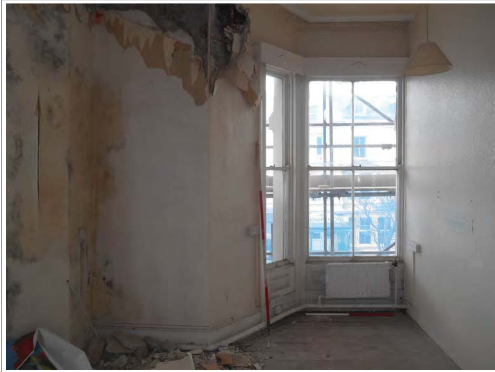
Plate 73. View of Room 7. Canted three-light window blocked by wall addition looking N.
