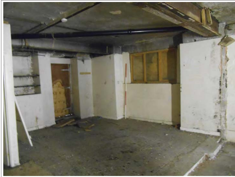
Plate 136. East facing wall. 1960's Window subsequently repaired. North facing wall with back entrance. Not original.
