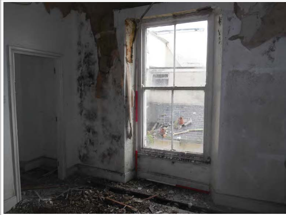
Plate 87. View of Room 9 with centre bar window and ensuite bathroom, looking E.
