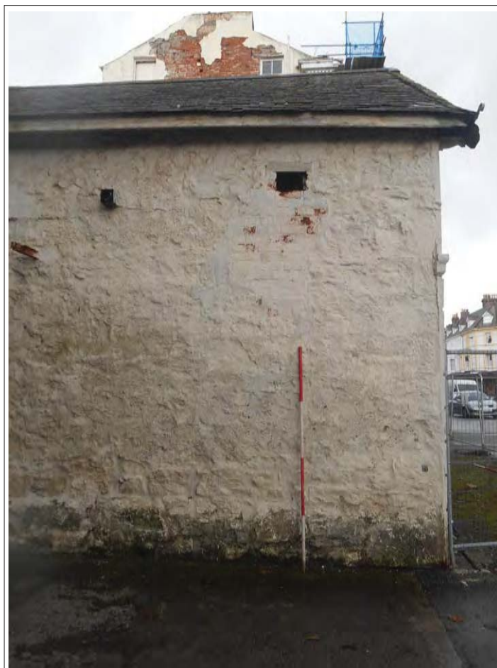
Plate 149. Detail of repair or alteration of possible window or vent.
