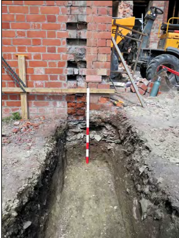
Plate 5. The southwest footing, showing Section A (below modern brick wall). Scale: 1m. Looking northwest.
