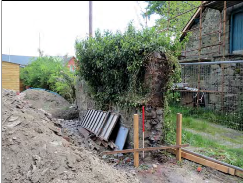
Plate 11. General view of stone wall along the southwest site boundary. Scale: 1m. Looking south-southeast.
