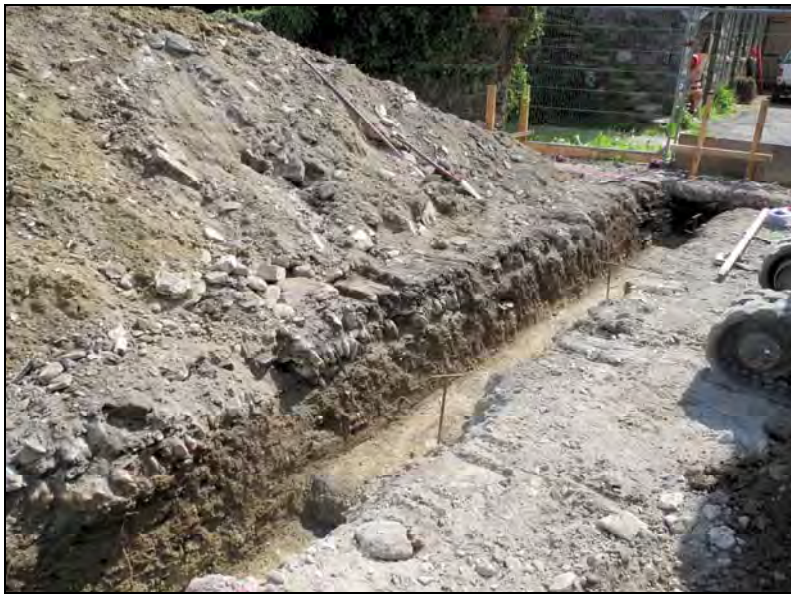
Plate 18. Oblique view of northwest-facing section along the southeast footing, showing layer of cobbles. Looking south-southwest.
