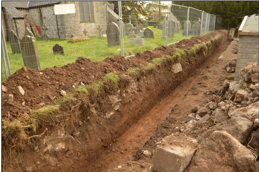
Fig. 4: The machine-excavated trench for the new wall foundations, from the north-east. CPAT 4558-0012
