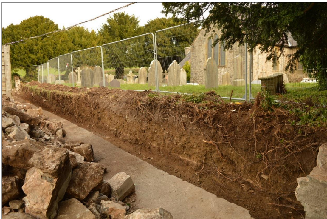
Fig. 3: The machine excavated trench for the new wall foundations, from the north-west. CPAT 4558-0009
