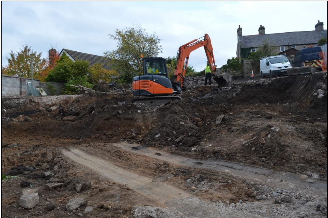
Photo 8. Ground reductions in the eastern area of the site, beyond the (demolished) modern wall. Note the depths of modern deposits on the left side of the picture, at the north-eastern area of the site. CPAT Photo 4078-0045
