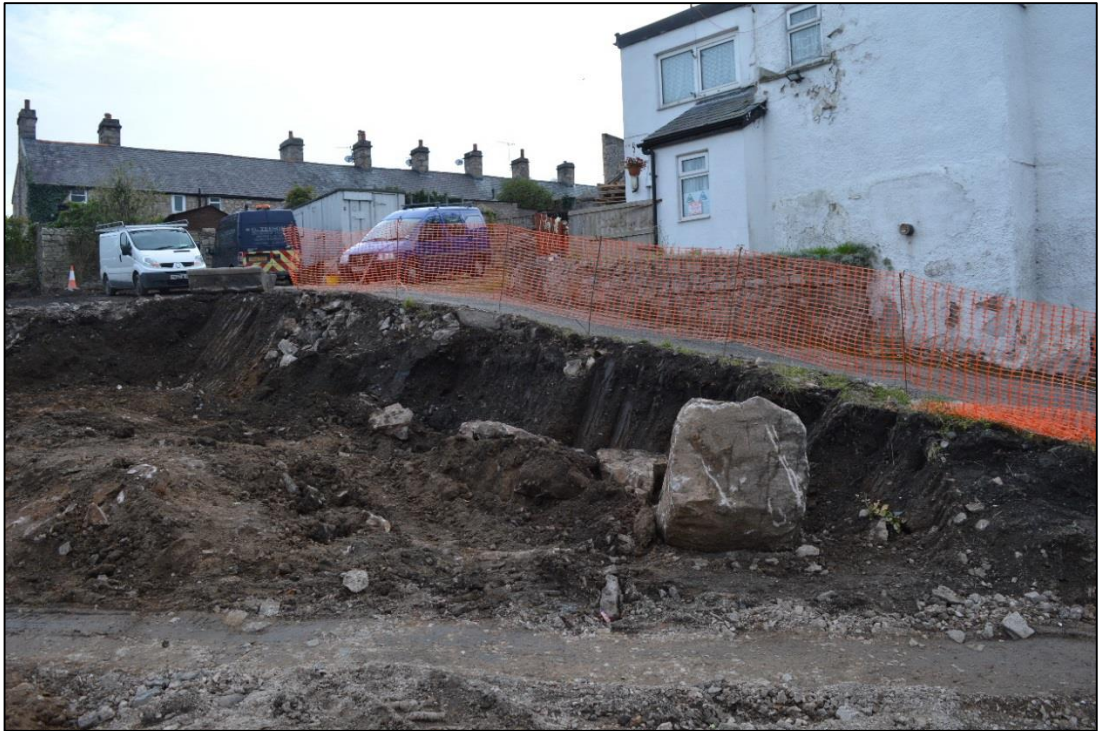
Photo 3. Ground reductions in the south-western area of the site revealed large limestone boulders in the sandy boulder clay subsoil. CPAT Photo 4078-0044
