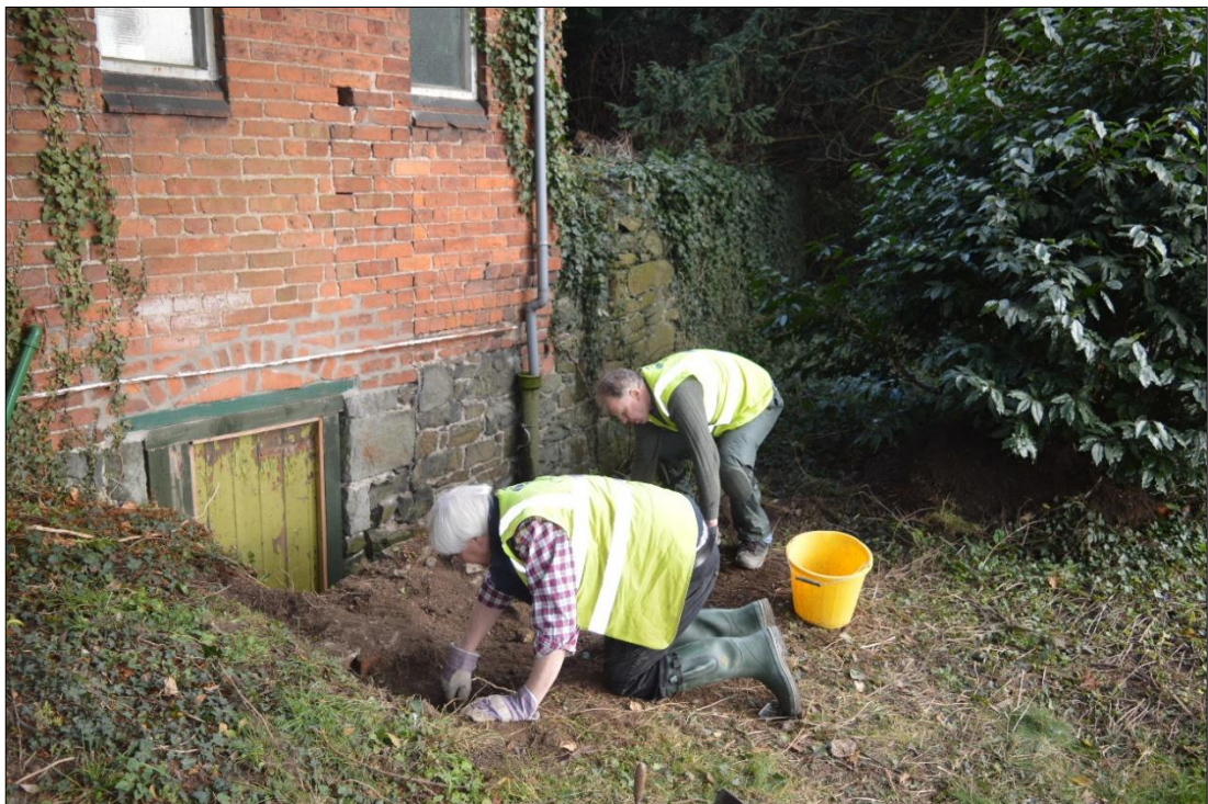
Fig. 7 Volunteers excavating Trench 2, located adjacent to the basement wall of the pavilion clubhouse, viewed from the west. Photo CPAT 4467-0026
