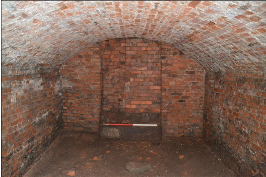
Fig. 4 The interior of the cellar, showing the blocked southern entrance. Photo CPAT 4699-0009
