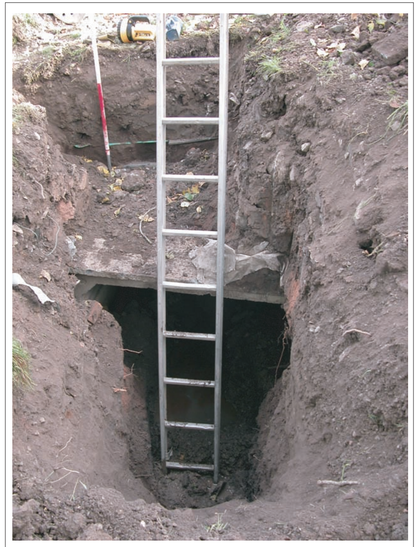
Plate 2: View of end of culvert in Trench 1, looking north-east, scale 1 x 1m.
